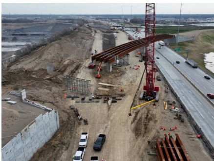
Bridge on IH-10 at US-69 EB Overpass at 11th Street Location: Beaumont, TX Client: TXDOT
