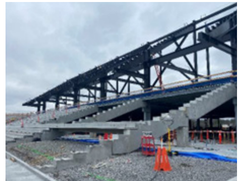
Testing and observation can occur during or after the erection process for connections that are welded, bolted, or between precast elements and the structural frame.
