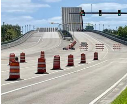
CEI Annual Services Contract 2021052 - Task Work Order 5: Donald Ross Rd Bascule Bridge Location: Palm Beach County, FL Client: FDOT District 4
