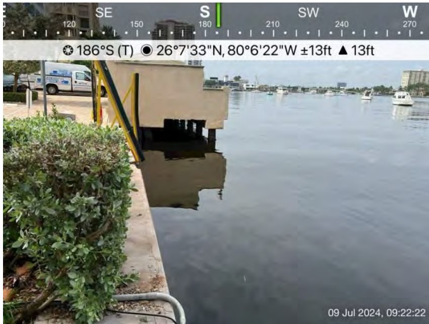
Photo 2 – Photo of Seville St seawall facing South. Note concrete panel wall with concrete cap.
