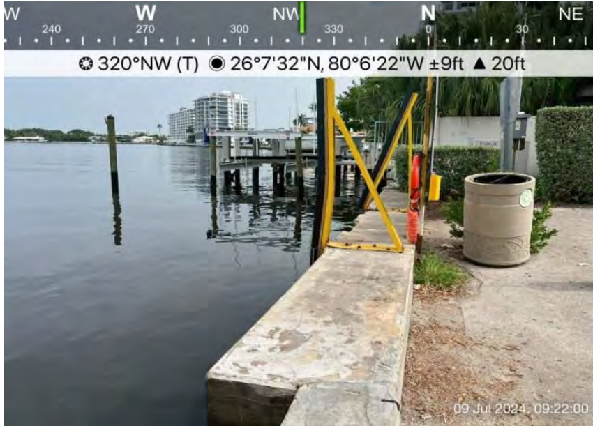
Photo 1 – Photo of Seville St seawall facing Northwest. Note concrete panel wall with concrete cap.
