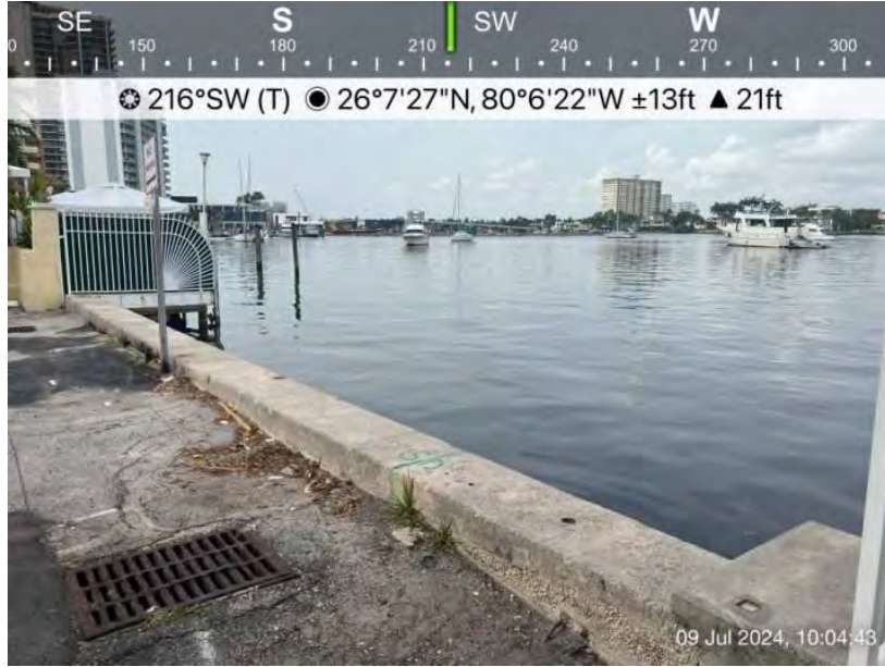
Photo 1 – Photo of Sebastian St seawall facing southwest. Note concrete panel wall and two storm drains with outfalls.
