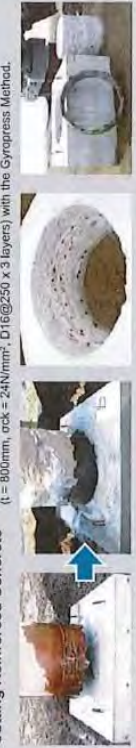
The images below show the cutting and penetrating into reinforced concrete (t = 800mm, rck = 24N/mm², D16@250 x 3 layers) with the Gyopress Method.
