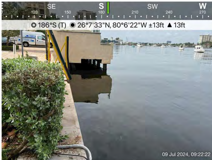
Photo 2 – Photo of Seville St seawall facing South. Note concrete panel wall with concrete cap.
