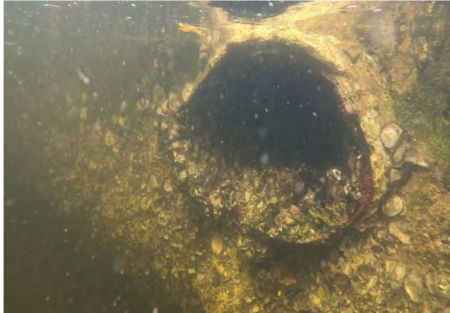
Photo 5 – Photo of survey area. Note one of the two outfalls and oysters on sea wall.
