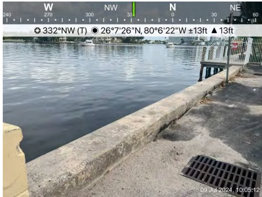
Photo 2 – Photo of Sebastian St seawall facing northwest. Note concrete panel wall and two storm drains with outfalls.
