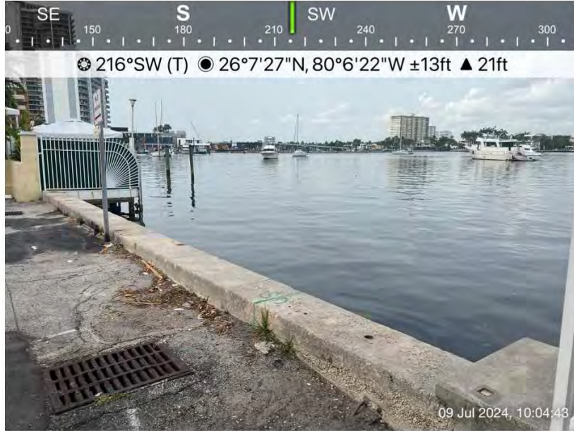
Photo 1 – Photo of Sebastian St seawall facing southwest. Note concrete panel wall and two storm drains with outfalls.
