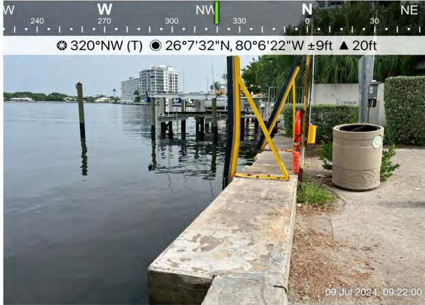
Photo 1 – Photo of Seville St seawall facing Northwest. Note concrete panel wall with concrete cap.
