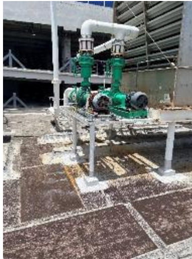
Figure 2B.2.7 Corrosion at chiller frame/pump bases
