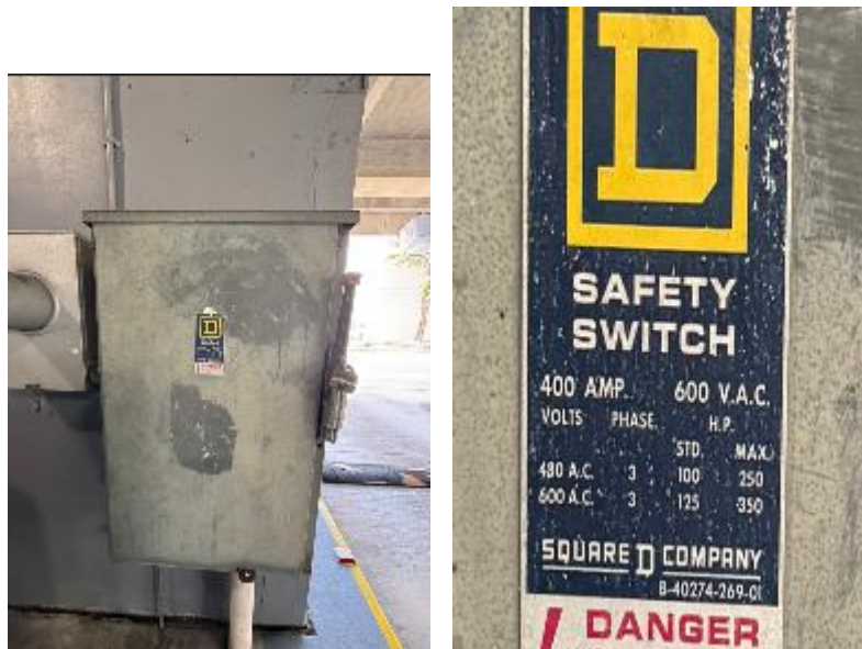
Figure 2A.6.24 Existing garage electrical service
