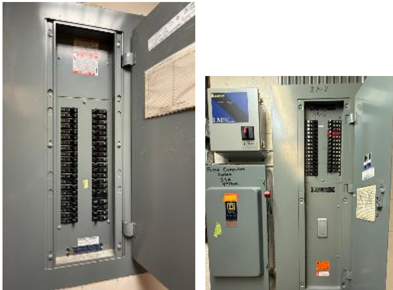
Figure 2C.6.10 Electrical Panels with Missing Breaker Identification
