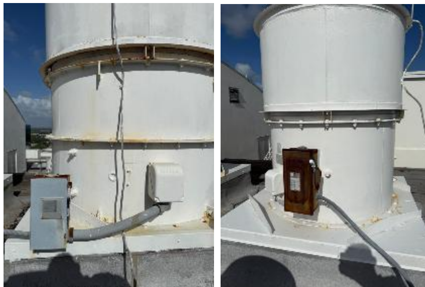
Figure 2B.6.22 Isolated corrosion, aging disconnect switches on the roof
