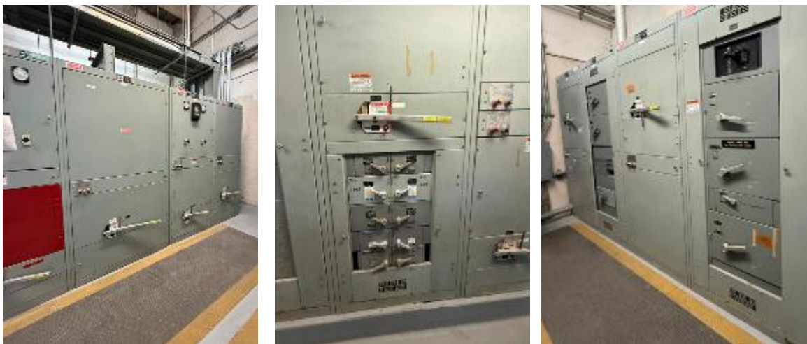
Figure 2A.6.4 Electrical main switchboards and primary electrical distribution
