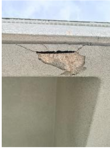
Figure 2C.2.3 Spalling at exterior framing edges
