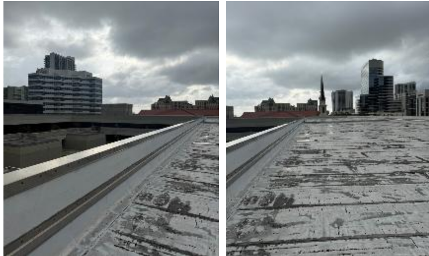
Figure 2C.6.21 Existing roof - no lightning protection system
