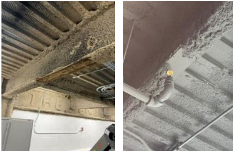
Figure 2A.5.5 Fire Proofing
