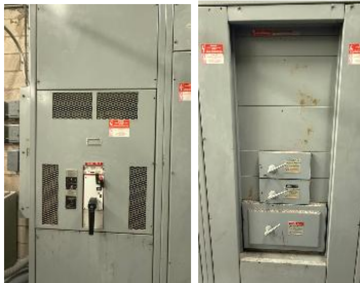
Figure 2B.6.3 Electrical Distribution equipment serving the 6-story tower
