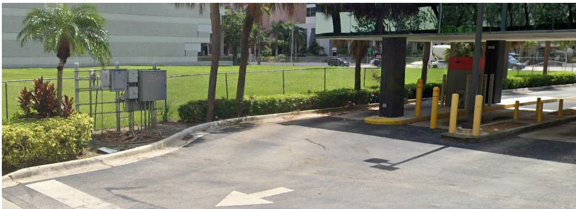
Electrical service for drive through. (low point of equipment est. 24-30 inches above grade)
