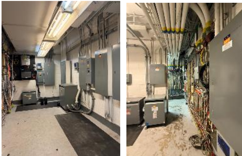
Figure 2C.6.10 Electrical rooms limited space
