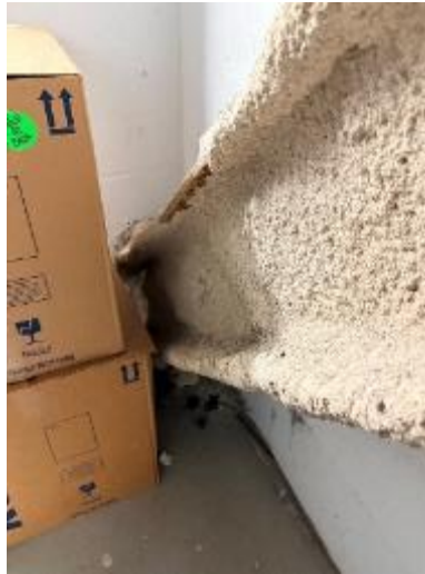
Figure 2A.2.5 Spray-applied fire proofing damage
