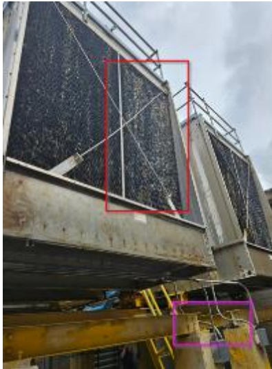
Figure 2C.4.2 Cooling tower fouling (red) and rusted framing (magenta)
