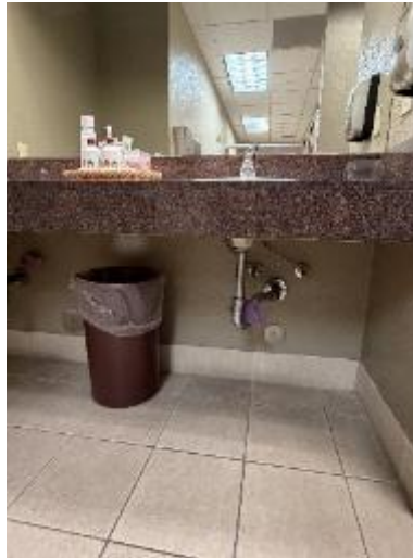
Figure 2B.3.6 No pipe protection
