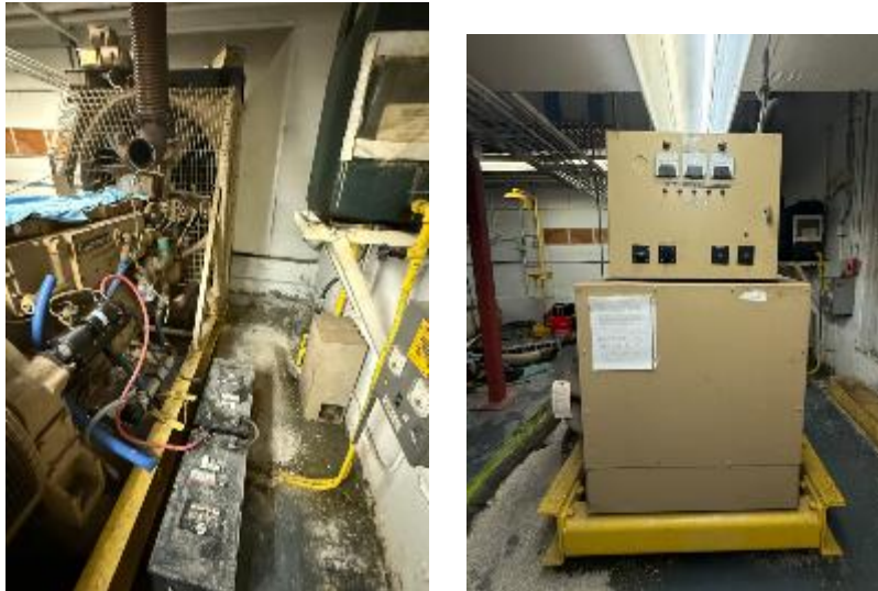
Figure 2C.6.16 Existing electrical generator
