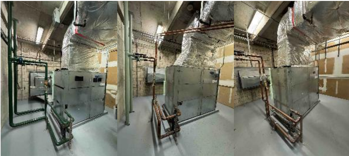
Figure 2B.4.3 AHUs in good condition
