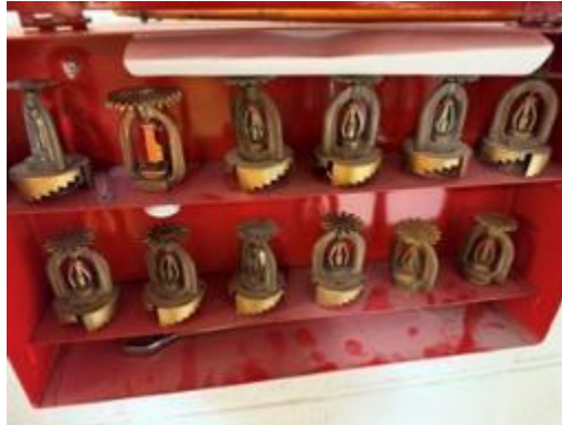
Figure 4.1- Sprinkler head cabinet
