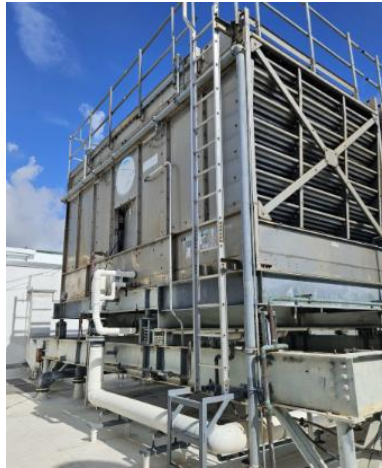
Figure 2A.4.3 Cooling Tower
