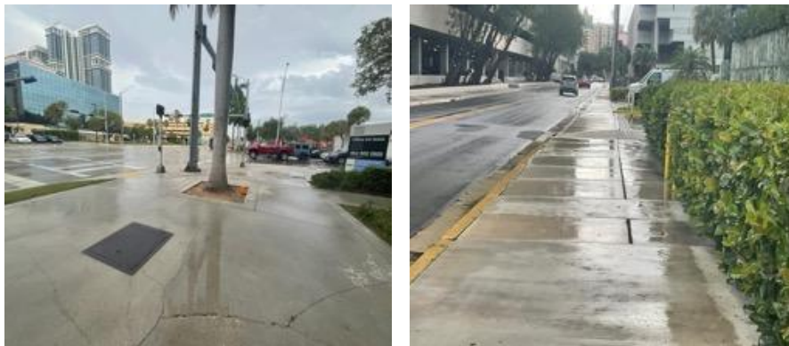
Figure 2A.8.2 Existing sidewalk cracks & horizontal gaps
