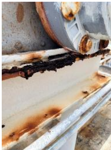
Figure 2B.2.8 Corrosion at chiller frame/pump bases
