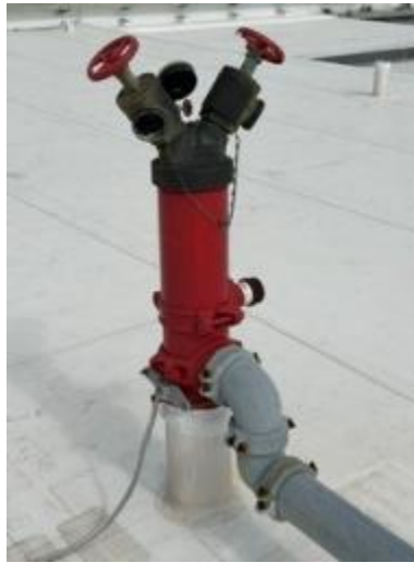
Figure 2A.5.3 Roof Manifold
