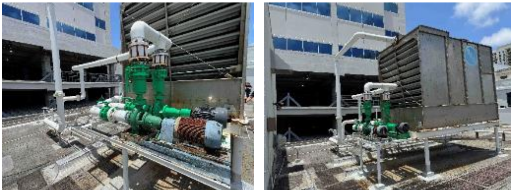
Figure 2B.4.8 Cooling tower
