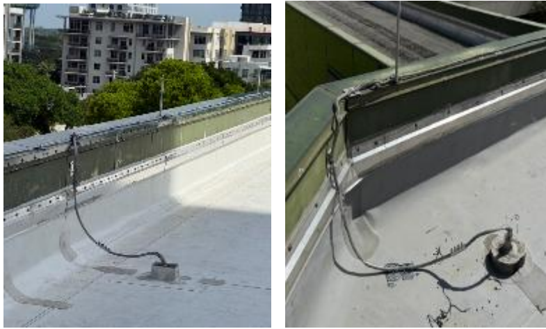
Figure 2A.6.17 Existing lightning protection system on roof
