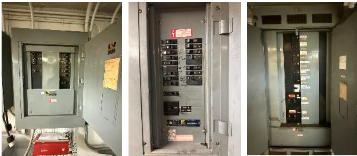
Figure 2C.6.2 Condition of existing electrical panels
