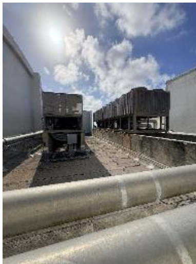
Figure 2B.2.6 Rooftop equipment
