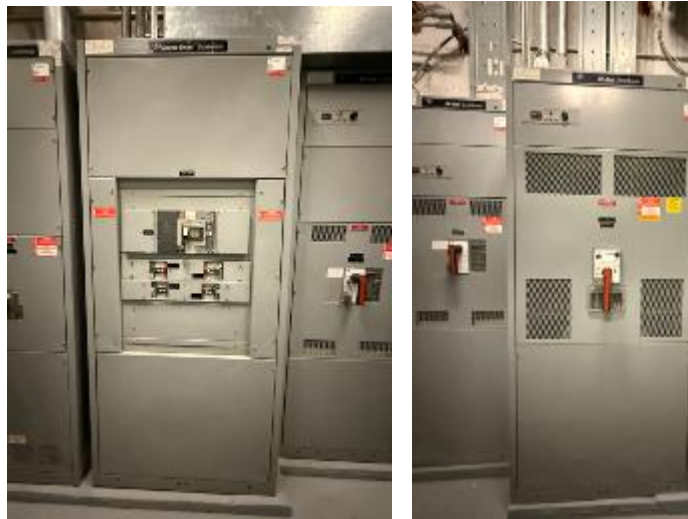
Figure 2B.6.1 Electrical distribution equipment (Tower)
