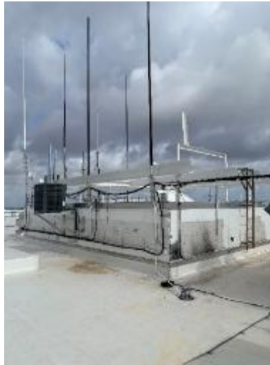
Figure 2A.2.7 Antenna farm frame
