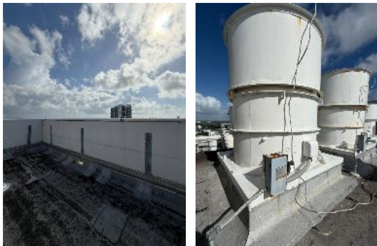
Figure 2B.6.21 Existing lightning protection on the roof
