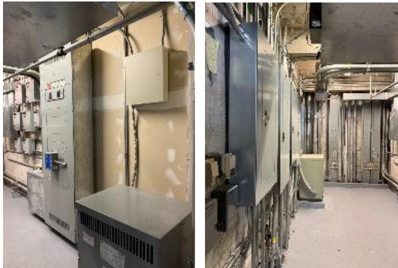
Figure 2B.6.30 Electrical room in the Parking Garage
