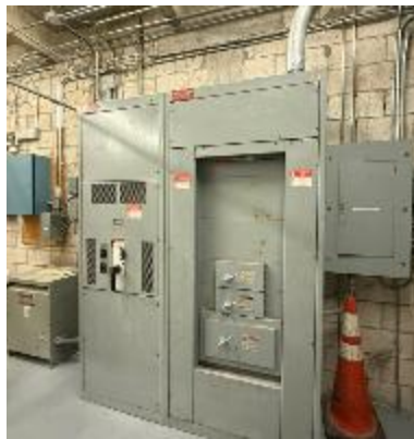
Figure 2B.6.2 Electrical distribution equipment (Center)
