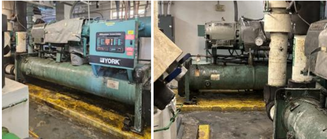
2C.4 1 Chillers with visible wear
