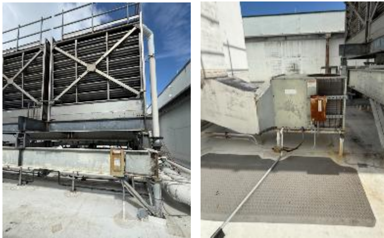
Figure 2A.6.20 Existing disconnect switches on roof
