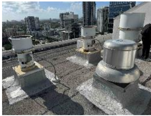
Figure 2B.4.6 Exhaust fans
