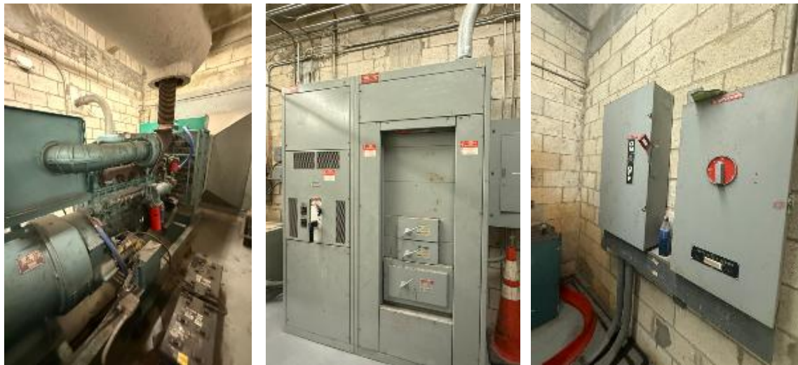
Figure 2B.6.16 Center generator and associated emergency power distribution
