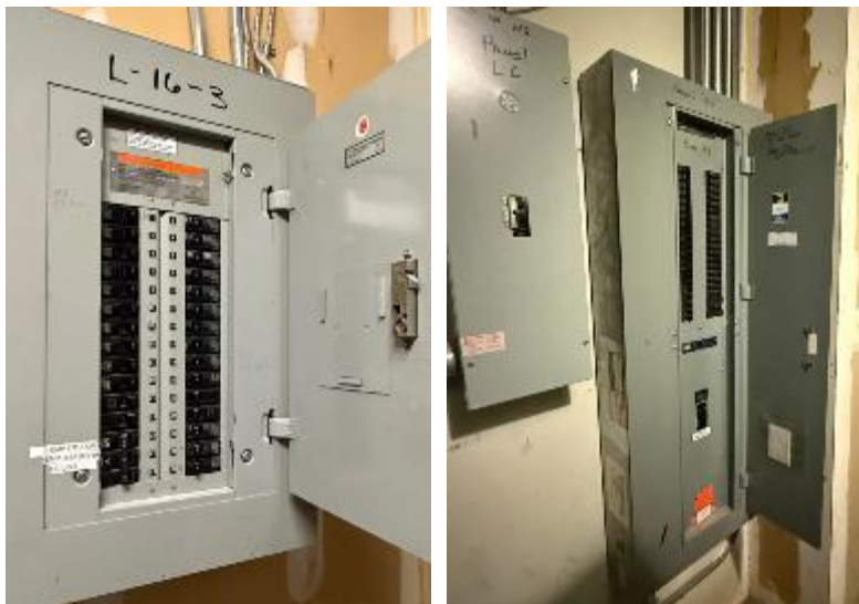
Figure 2A.6.1 Electrical working clearance deficiencies
