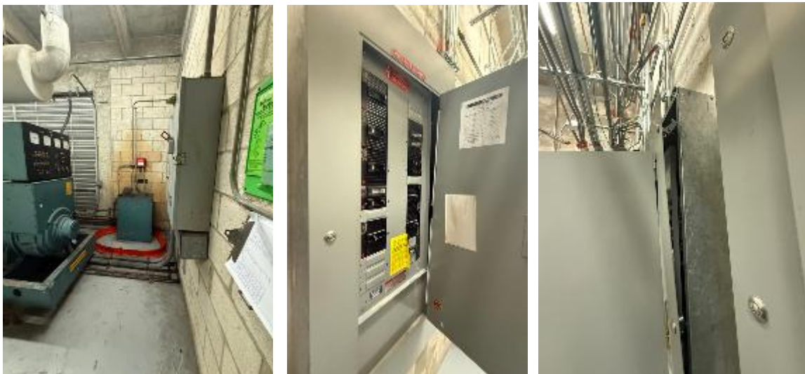
Figure 2B.6.7 Existing electrical equipment
