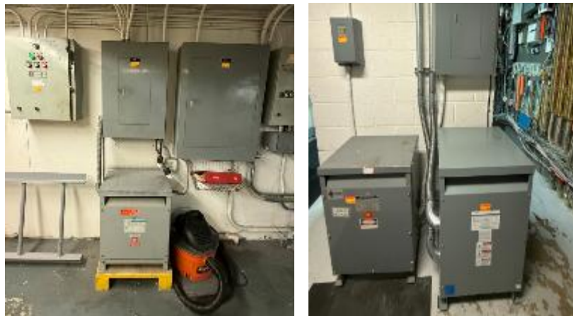
Figure 2C.6.7 Electrical panels with accessibility and clearance deficiencies
