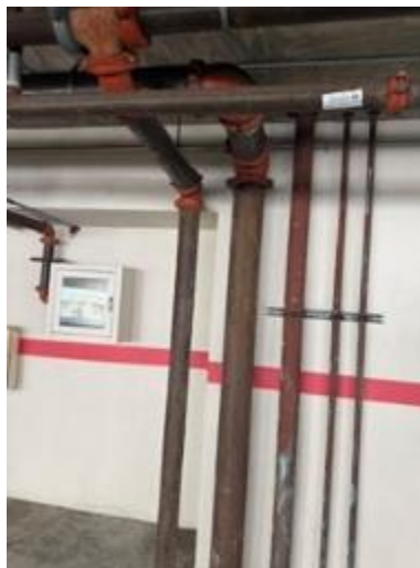
Figure 2B.5.5 Corroded Piping
