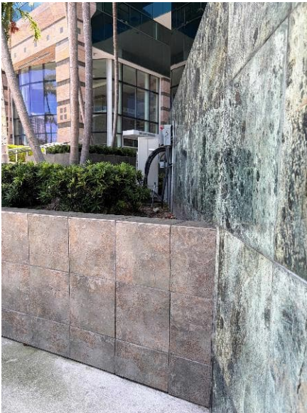
North side. This mini split AC unit sits at approx. 32" above grade.
