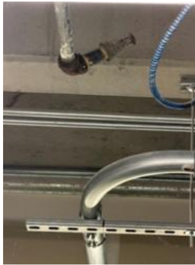
Figure 2B.5.6 Misaligned Sprinkler
