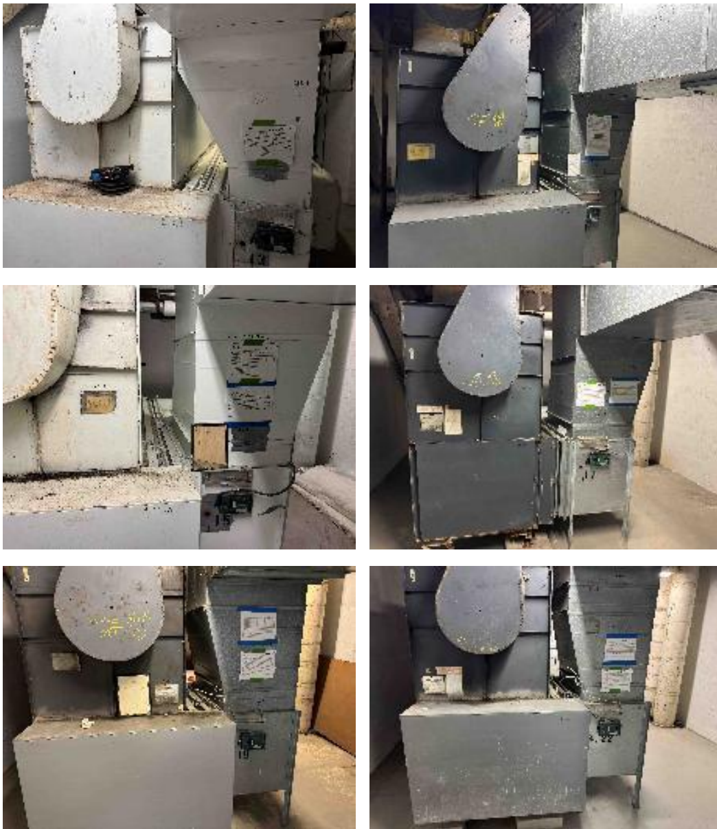
Figure 2A.4.2 AHUs requiring replacement
