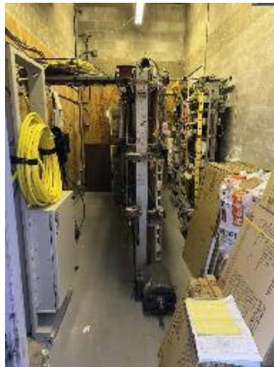
Figure 2A.7.3 TS-1E-001 First Floor Telephone Room
