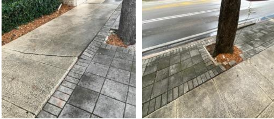
Figure 2B.8.1 Existing sidewalk cracks & Recommend tree grates (typical)
