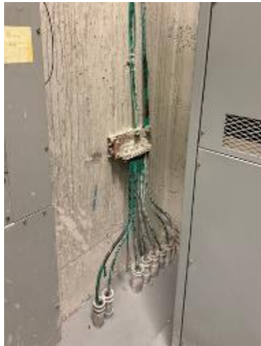
Figure 2B.6.21 Grounding bar located in the main electrical room
