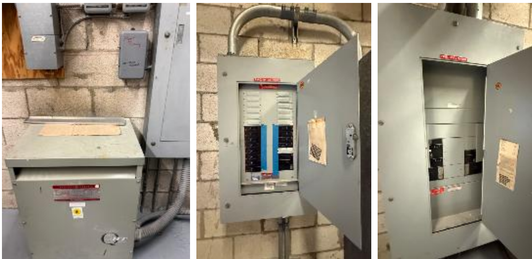
Figure 2B.6.4 Existing electrical panels (Center)
