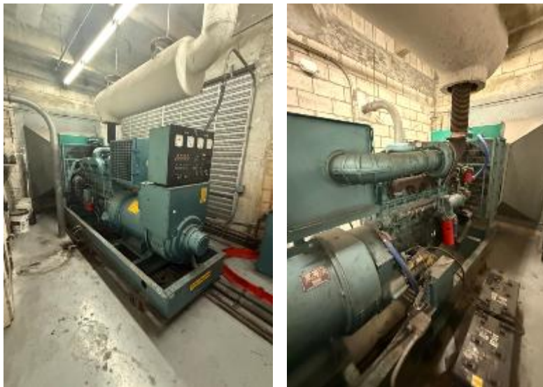
Figure 2B.6.14 Emergency generator (Center)
