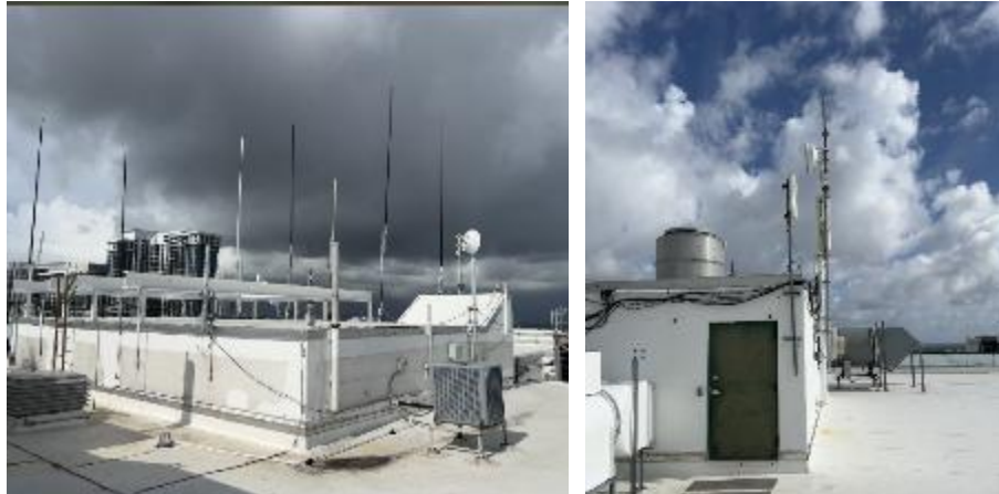
Figure 2A.7.29 Antennas on the Roof
