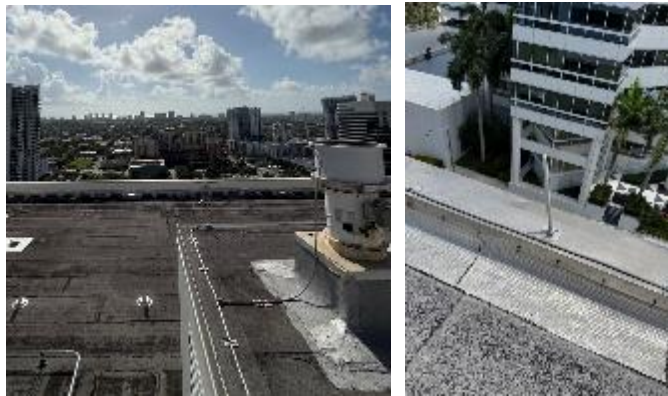
Figure 2B.6.21 Existing Lightning Protection System
