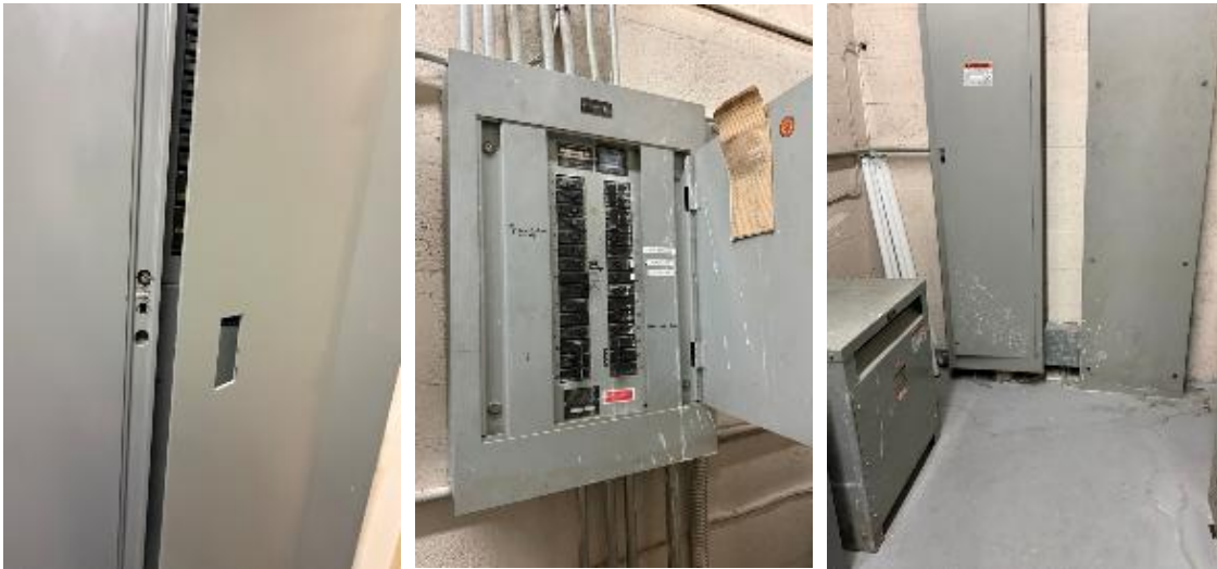
Figure 2A.6.3 Electrical panelboards condition and deficiencies
