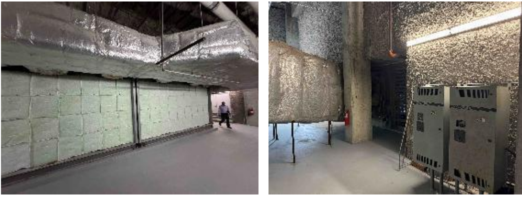
Figure 2B.4.2 Penthouse AHUs
