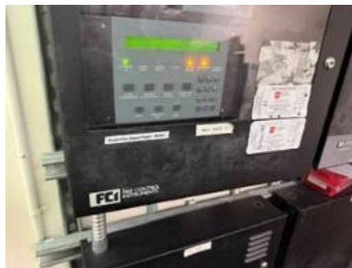
Figure 4.3.2- Fire Alarm Control Panel
