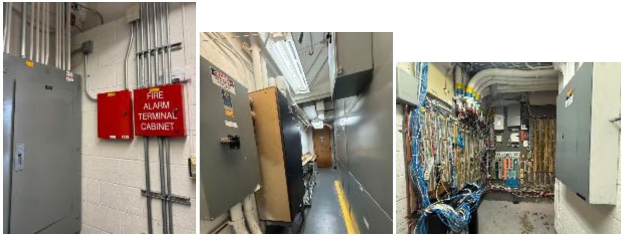
Figure 2C.6.6 Examples of electrical room working clearance deficiencies
