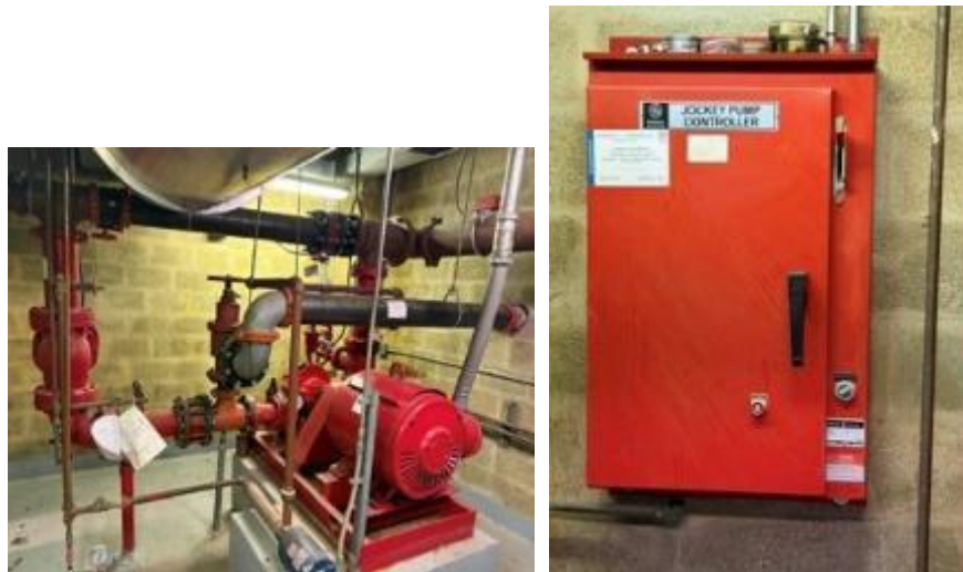
Figure 2A.5.1 Fire Pump/Controller
