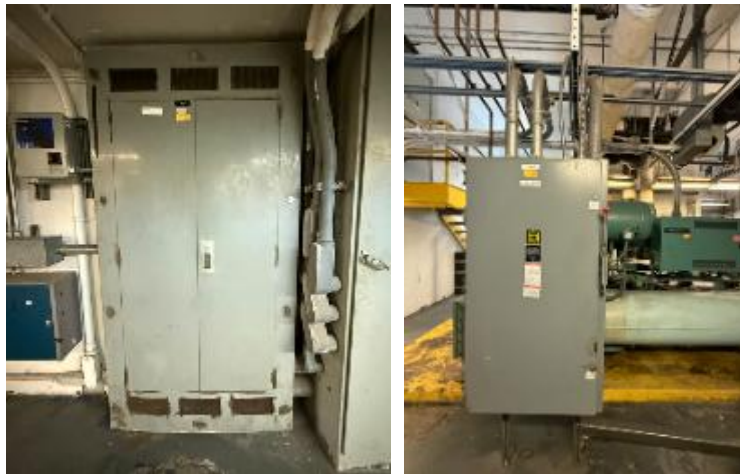
Figure 2C.6.23 Existing electrical equipment
