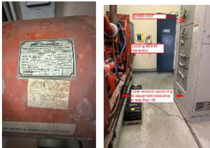
Figure 2A.6.14 Existing emergency generator
