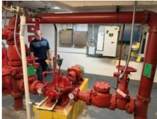
Figure 4.3.3- Fire Pump Room
