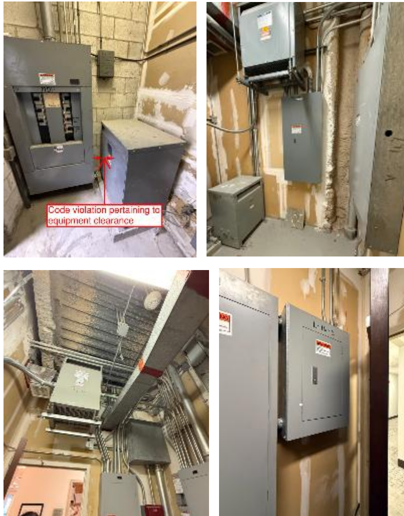
Figure 2A.6.6 Electrical equipment working clearance deficiencies
