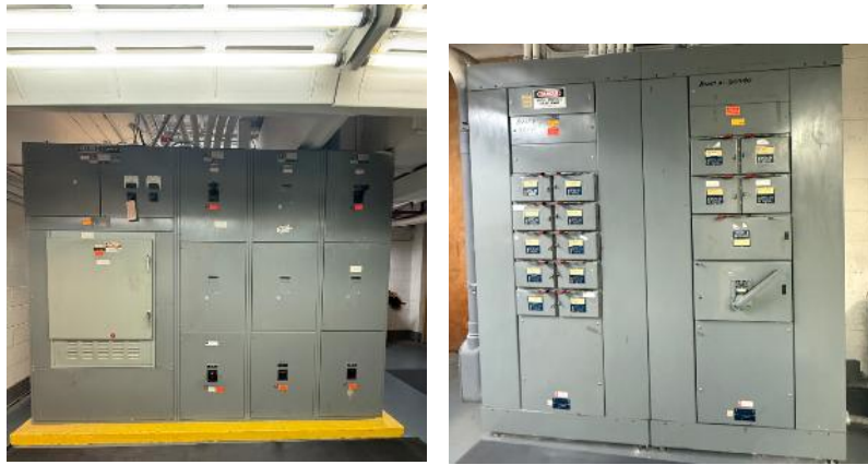
Figure 2C.6.1 Electrical distribution equipment
