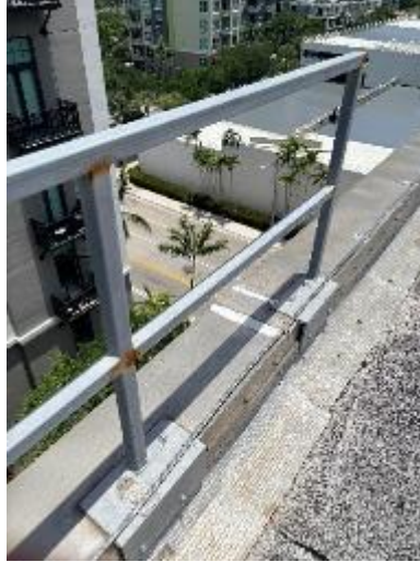
Figure 2B.2.9 Corrosion at railing welds
