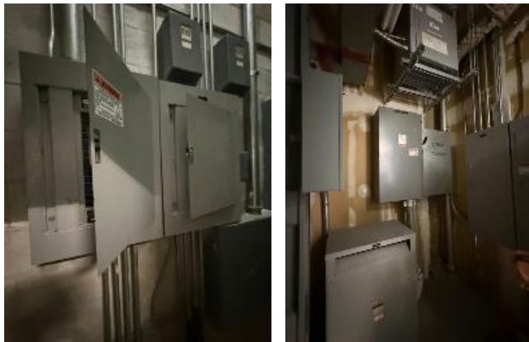
Figure 2A.6.7 Electrical rooms inadequate lighting levels
