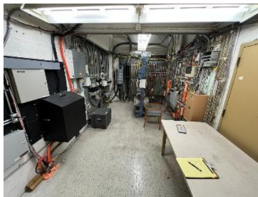
Figure 2C.7.1 Main telephone room
