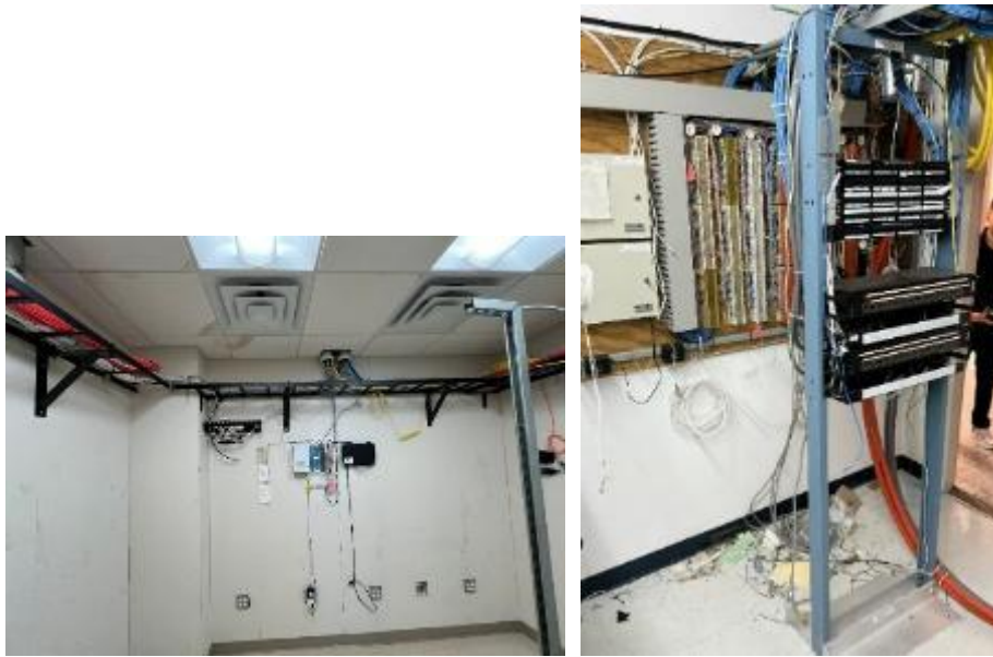
Figure 2A.7.17 Tenant Owned Telephone Closets (TS 1E-009, 9 th Floor & TS 1E-017, 17 th Floor)
