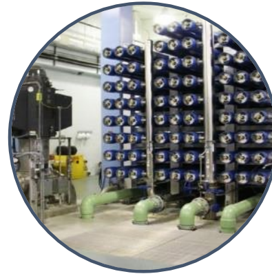
Dixie WTP Nanofiltration Constructed 2008
