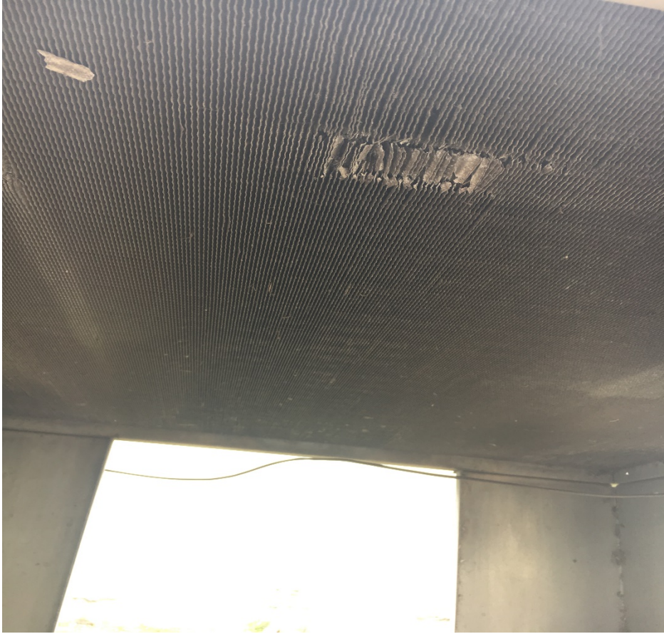
Stulz CRAC condensing unit coil badly corroded. View from bottom shows flaking fins that are typical in 10+ year old condensing units in humid environments.
