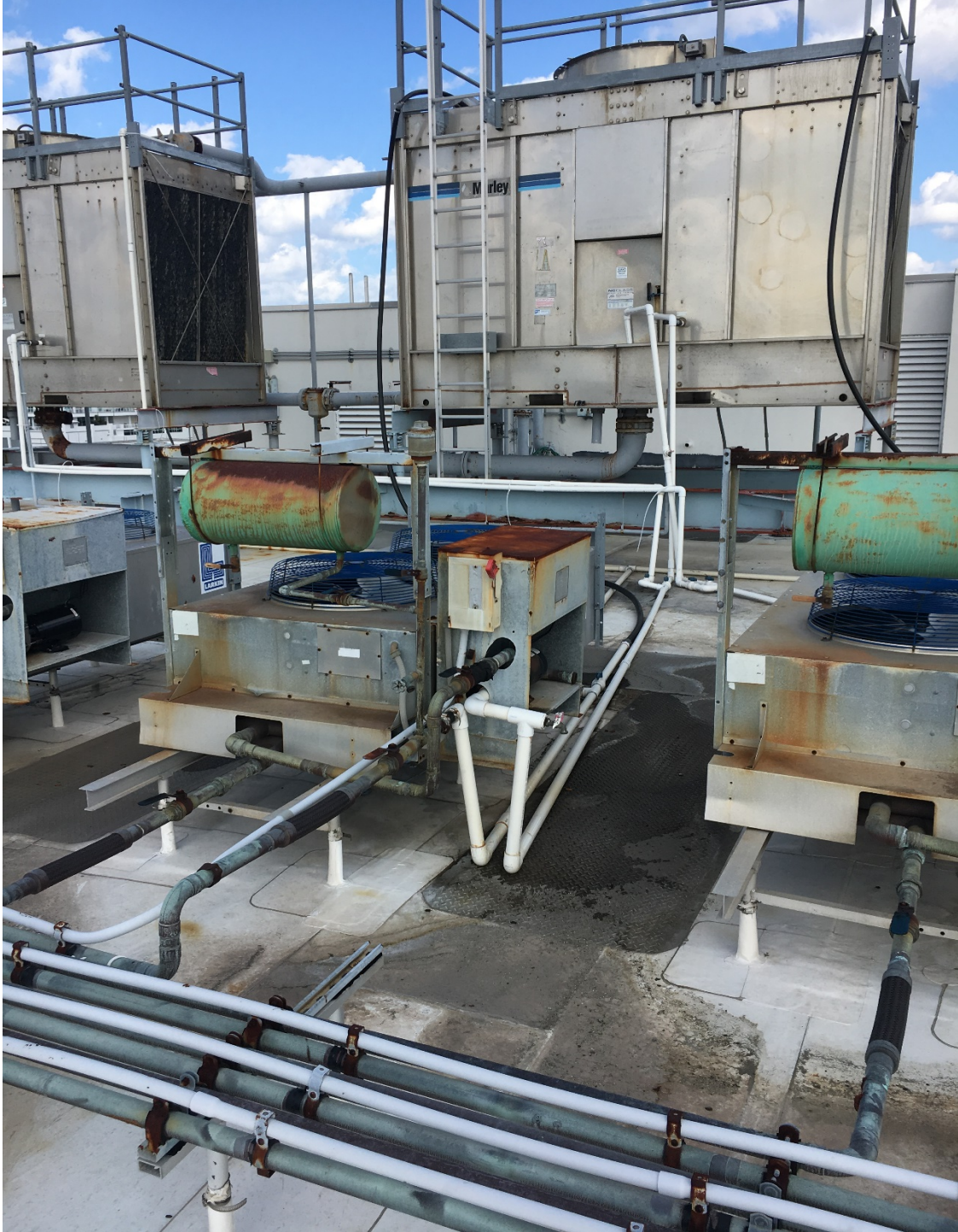
Dry-coolers bypassed and connected to cooling tower open loop.
