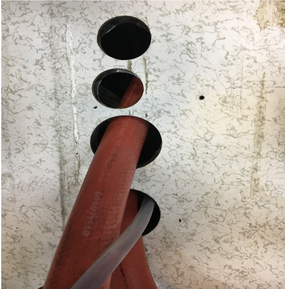
Flexible water lines being cut by sharp edges of floor tiles.
