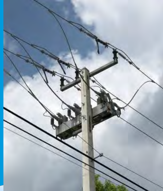
Main power line
