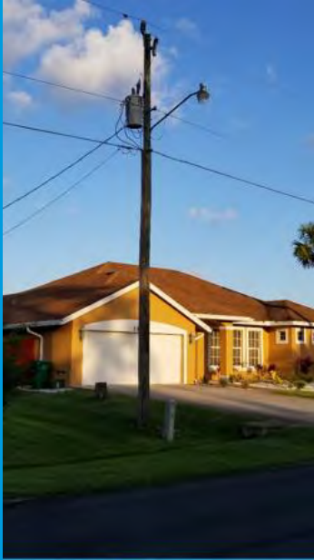
Neighborhood power line
