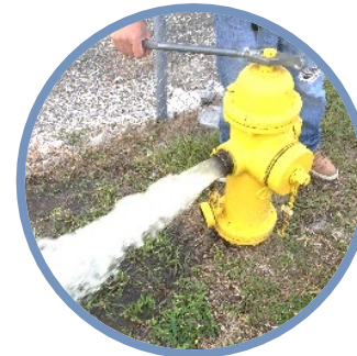
Distribution System Testing
