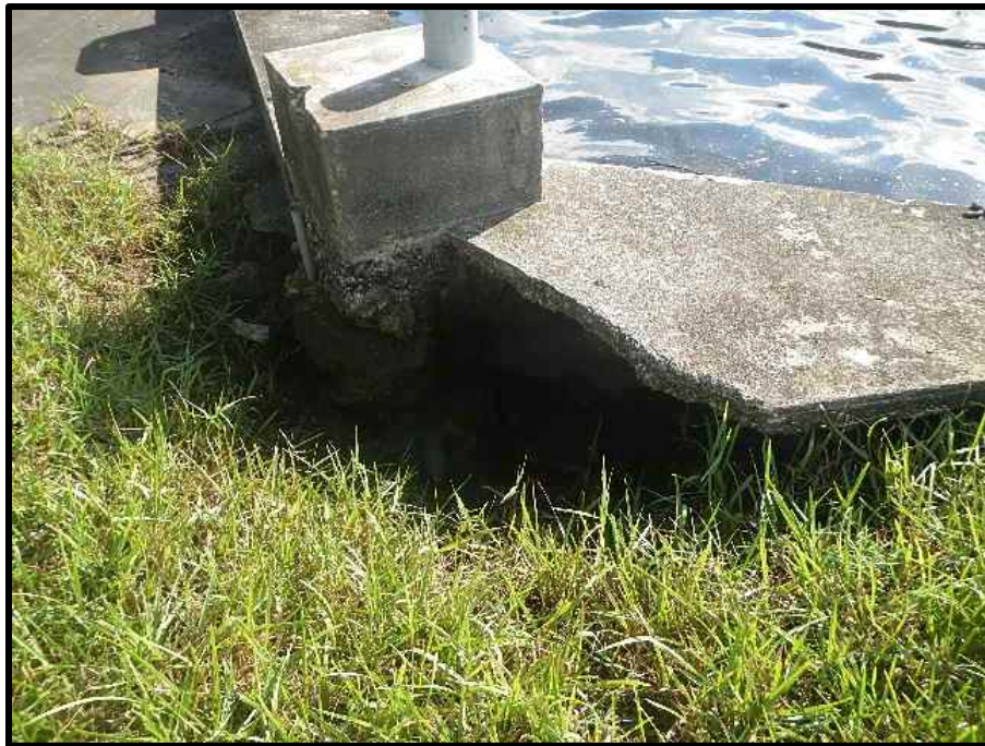
Above: 7. View of undermining of corner of seawall along the river.
