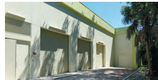
Figure 17. Acoustical measurements will be taken once construction is complete to verify the sound levels measured during the simulation. This image shows the installation of doors and roll-up doors in the chiller building. The man door to the right of the image opens into the cooling tower well.
