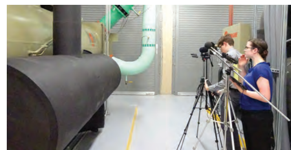
Figure 10. Acoustical measurements and recordings of the chillers and pumps inside an existing facility similar to the proposed central energy plant.
