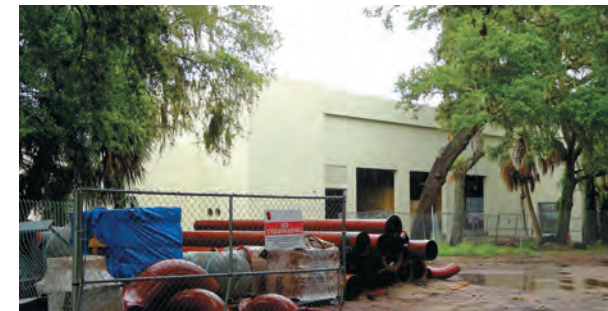
Figure 16. Acoustical measurements will be taken once construction is complete to verify the sound levels measured during the simulation. This image shows the chiller building before doors are installed and chilled water pipes stored on site.
