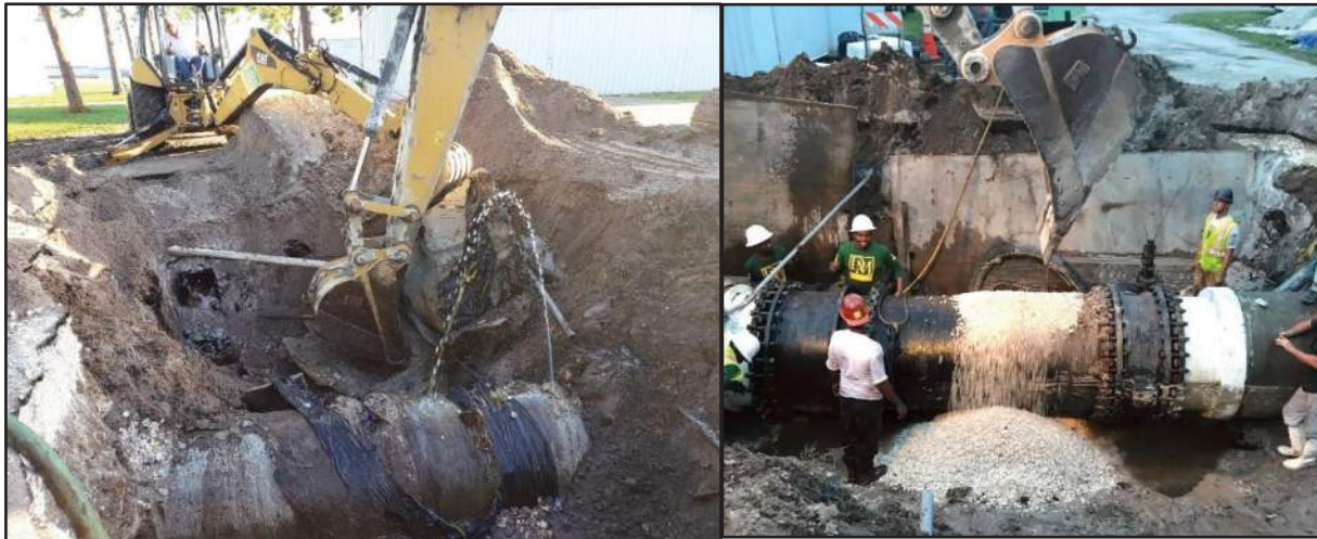
Figure #2: DMSI mobilized and completed repair of 42-inch raw Water main break in day one (Prospect Wellfield)
