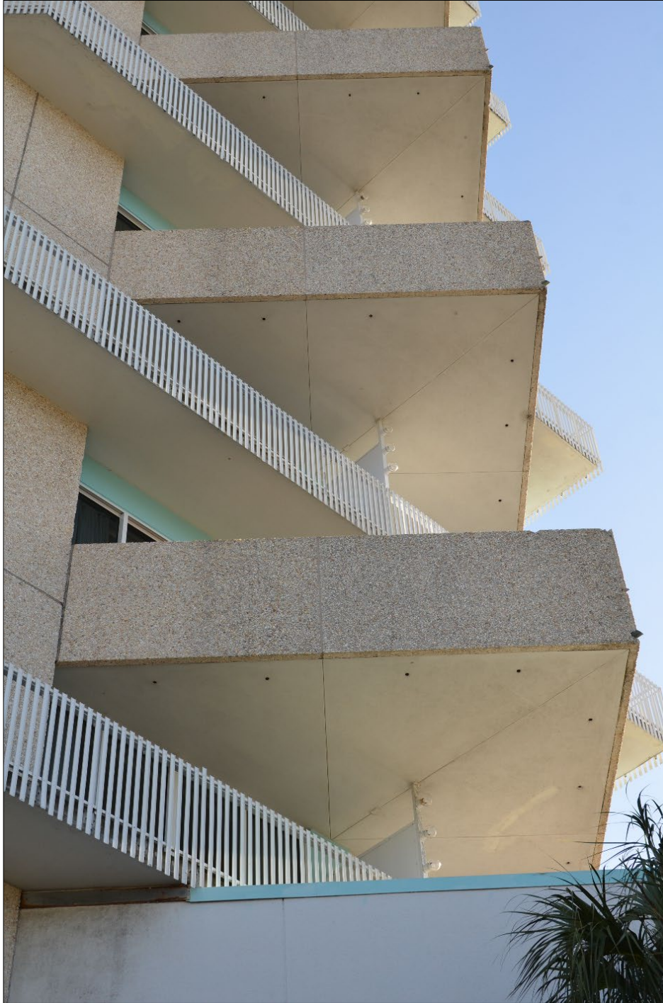
Figure 5. Pier 66 Hotel Tower. Partial west elevation, camera facing up and southeast. Photograph taken January, 2018.
