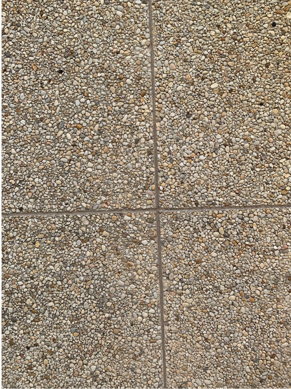
Figure 15. Pier 66 Hotel Tower. Precast concrete panels with expose Chattahoochee aggregate, camera facing north. Photograph taken October 18, 2022.
