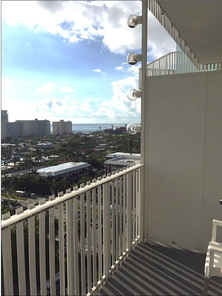
Figure 8. Pier 66 Hotel Tower. Aluminum balconies, room dividers and exterior light post. Camera facing southeast. Photograph taken October, 2017.
