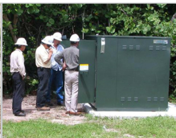
FPL Capacitor bank
