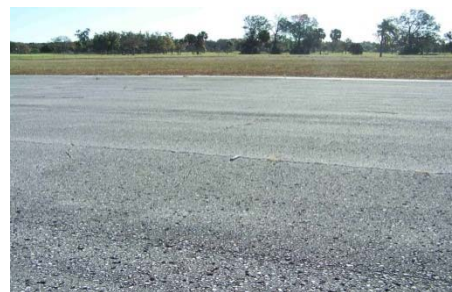
Figure 2 - Corrugation (Ripple) Distress
