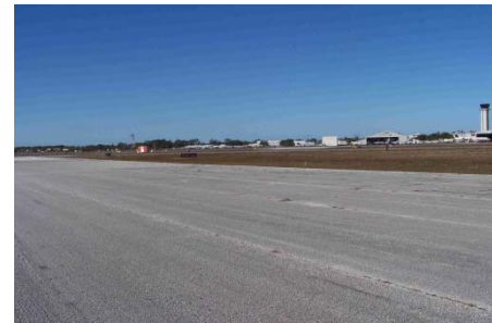
Figure 1 - Longitudinal Crack Distress
