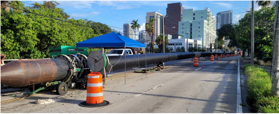
30-inch HDPE Water Main - Approximately 1,000 LF to cross under the Tarpon River.
