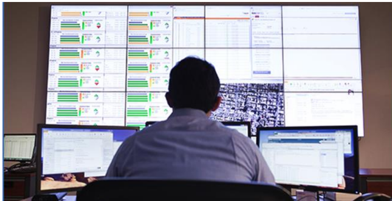
Figure 2: Wall panel of the NOC in Atlanta, Georgia
