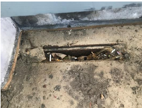
Debris in Drain
