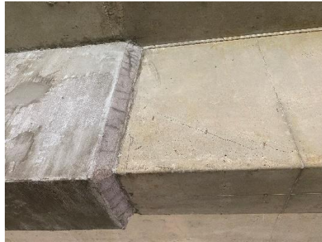
Overhead Beam Crack
