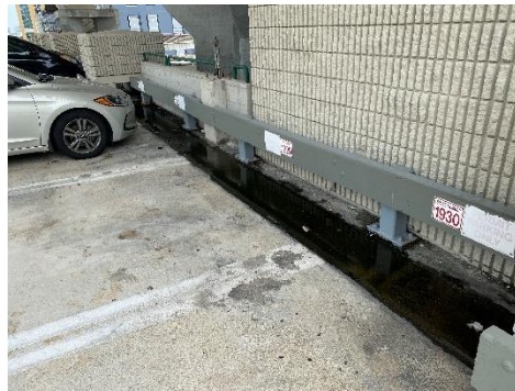
Water Ponding – Trench Area
