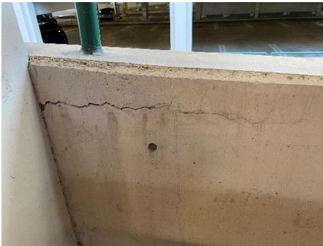
Concrete Wall Spall
