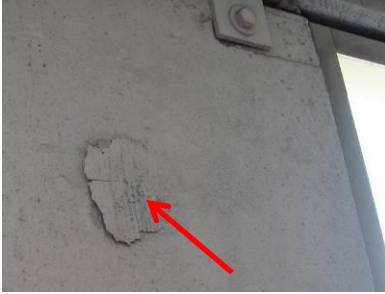
Figure 1: Failing Concrete Patch
