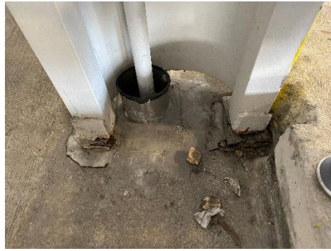
Pipe Support Rust
