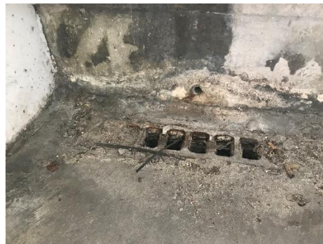
Debris in Drain
