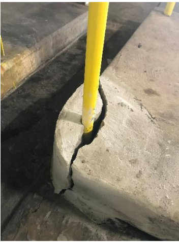
Pipe Support Rust
