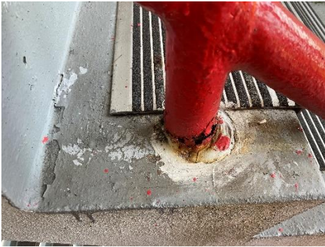
Stair Railing Post Corrosion
