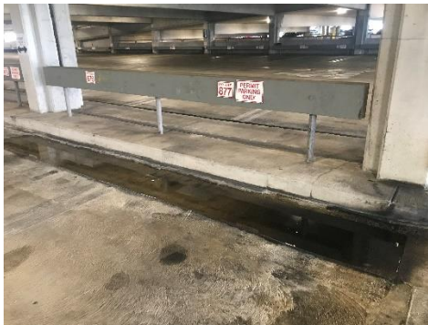
Water Ponding – Trench Area
