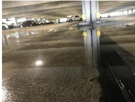
Water Ponding at Expansion Joint
