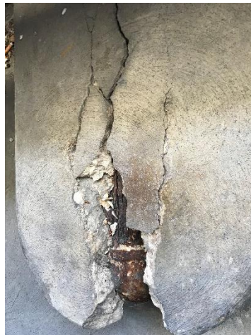
Steel Pipe Rust
