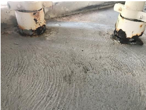
Pipe Support Rust
