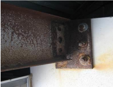
Figure 9: Structural Steel Rust and Scaling
