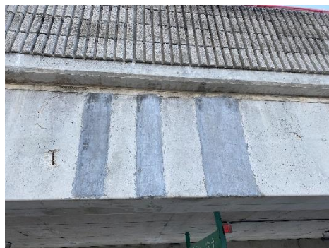
Overhead Beam Spalls
