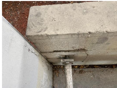
Masonry Wall at Angle
