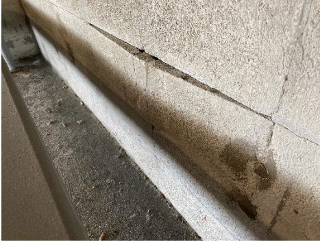
Masonry Wall Spall
