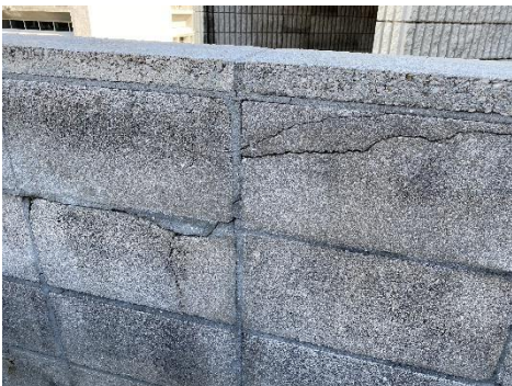
Masonry Wall Crack
