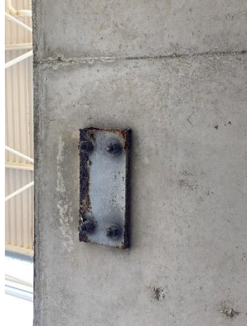
Steel Plate Rust
