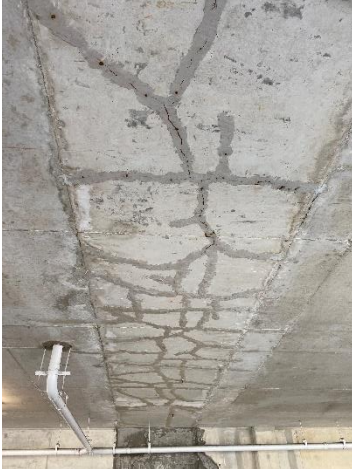
Overhead Floor Cracks
