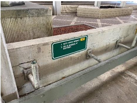
Masonry Wall Spall
