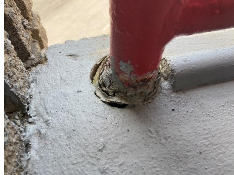
Stair Railing Post Corrosion
