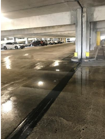
Water Ponding at Expansion Joint
