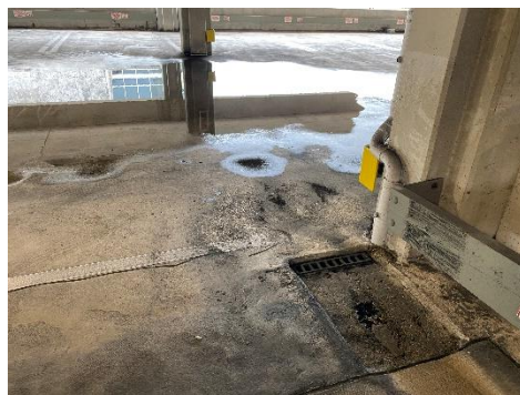
Pipe Discharging to Trench Area
