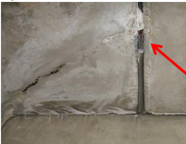
Figure 7: Leaking and Leaching Concrete
