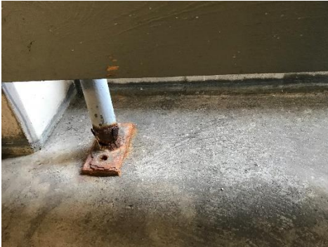
Steel Plate Rust
