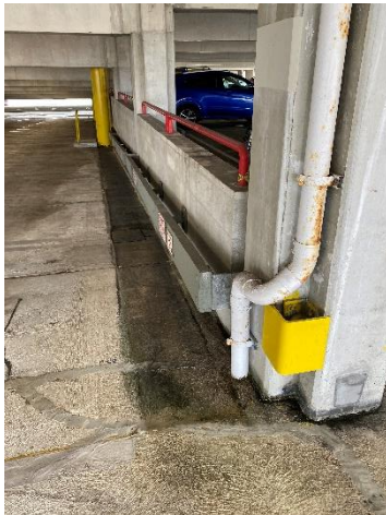
Pipe Discharging to Trench Area
