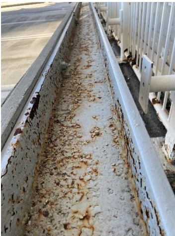
Steel Beam Rust
