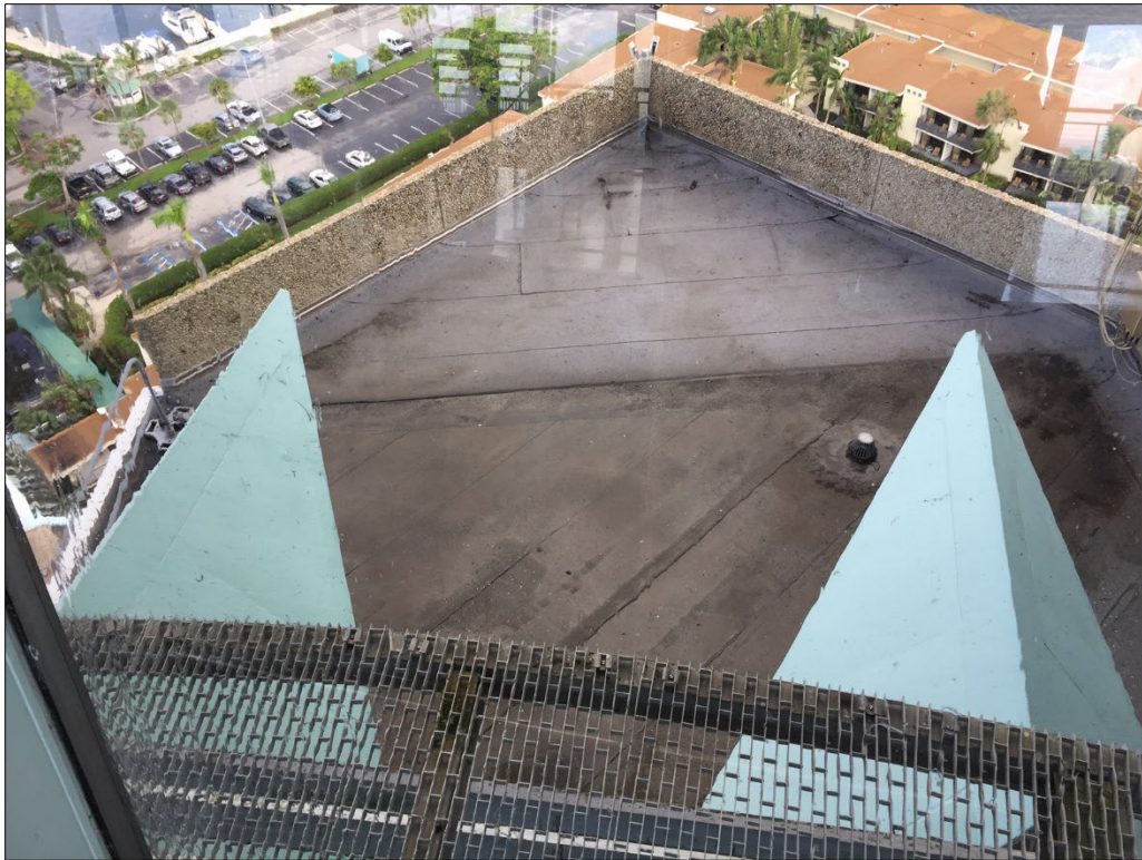
Figure 7. Pier 66 Hotel Tower. Trihedrons. Camera facing down and northwest. Photograph taken October, 2017.
