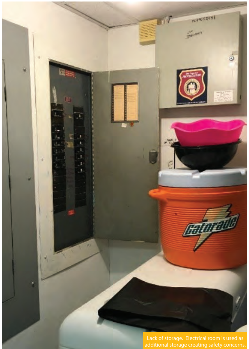
Convoluted Rooms not intended for Storage Space creating hazardous conditions.
