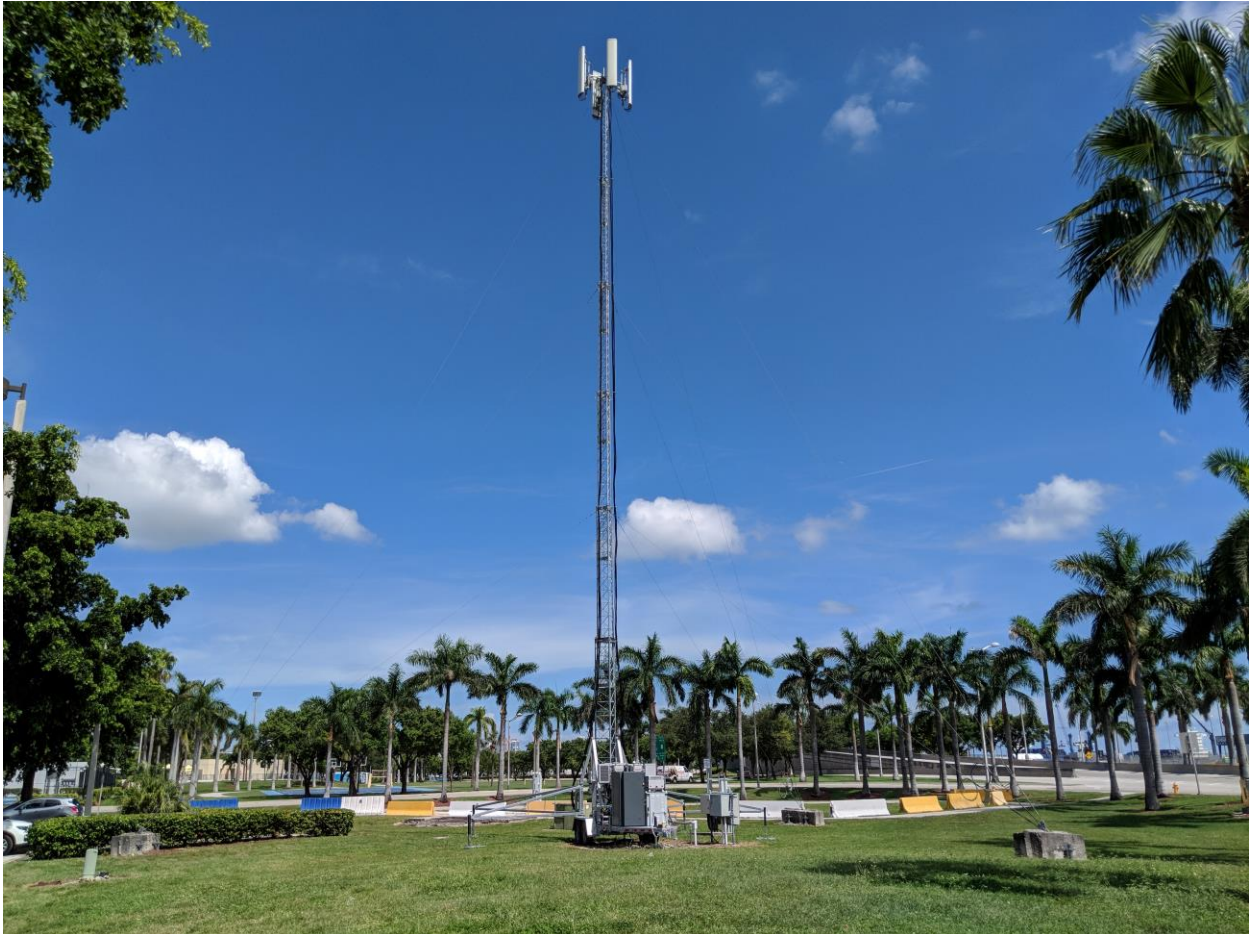
Alltech Tower At Port Of Miami Guyed To Concrete Blocks
