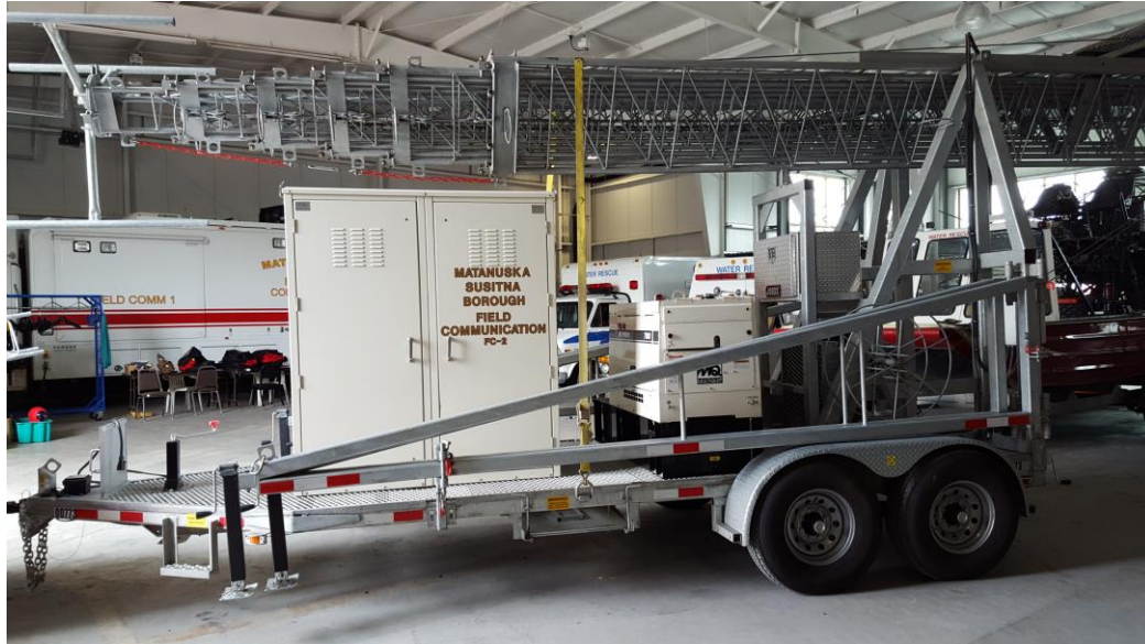
Emergency Management System With Enclosure and Generator
