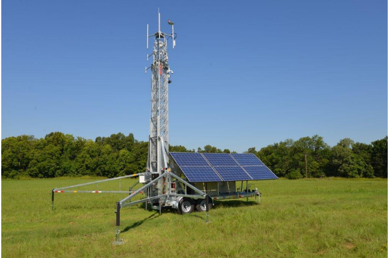
Generator and Solar Package
