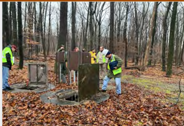
Camp Greentop Lift Station
