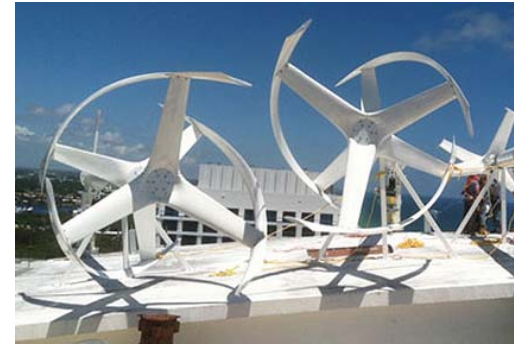
[Figure 4.266] Wind turbines on top of a hotel at Fort Lauderdale beach.
