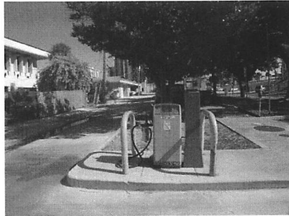
Diesel Fuel Dispenser and Pumping Station
