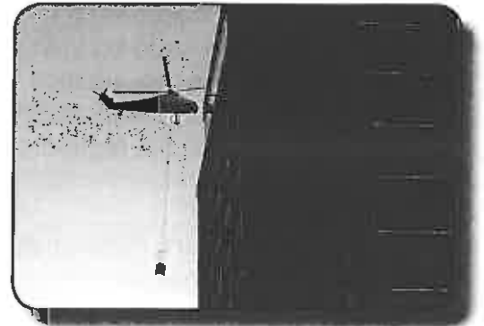
A helicopter was used to transport the elevator pressurizer fans on top of the towers.
