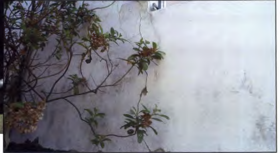
Major Wall Crack
