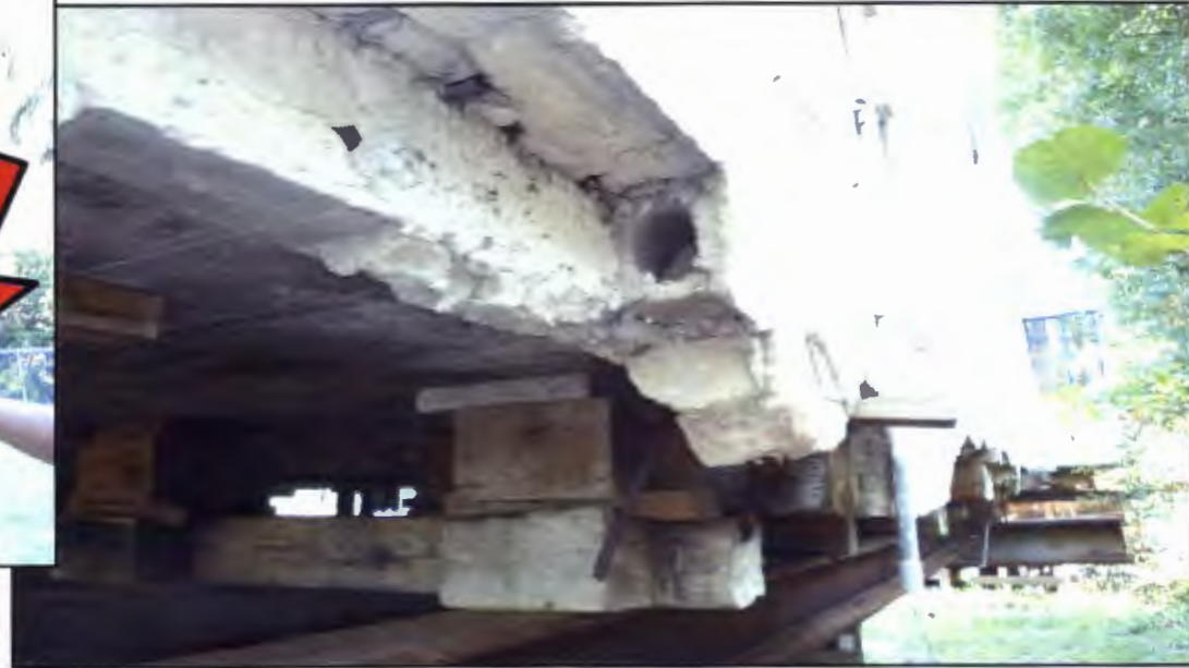
Foundation Cracks/ Parts falling off
