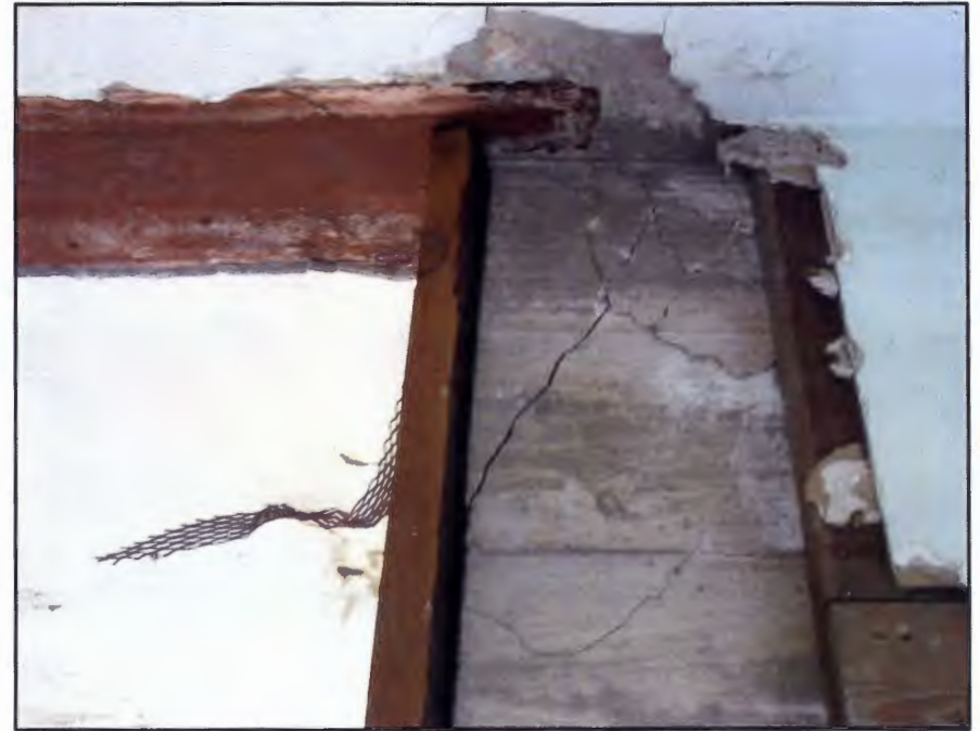
Major cracks in support beams
