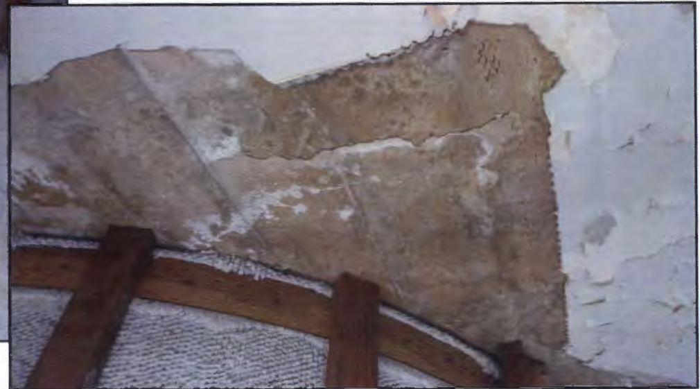
Looks like plaster but roof concrete is splitting.
