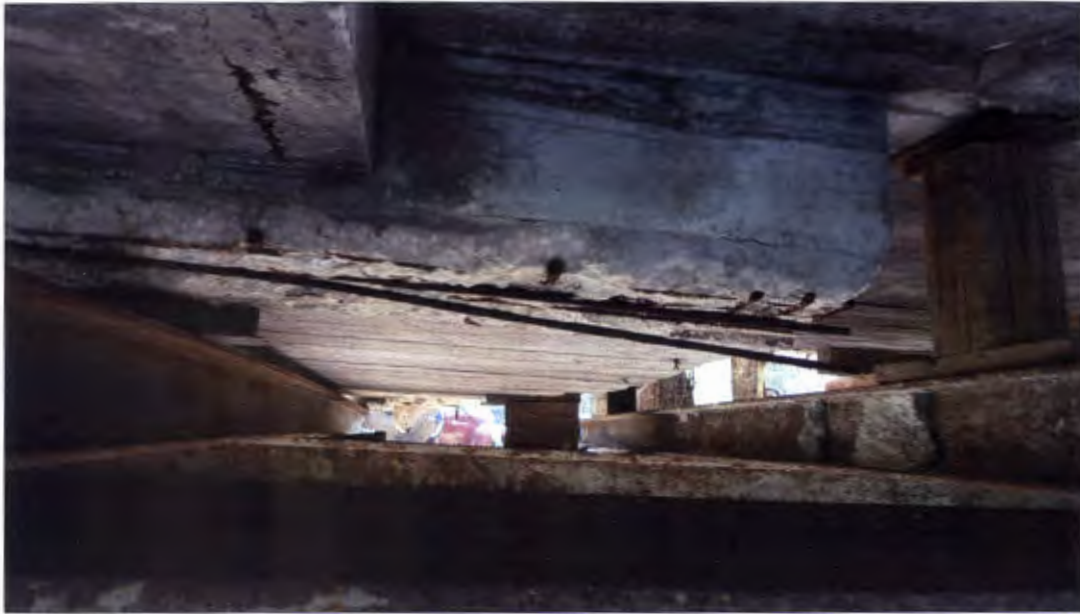
Rusting rebar on the floor
