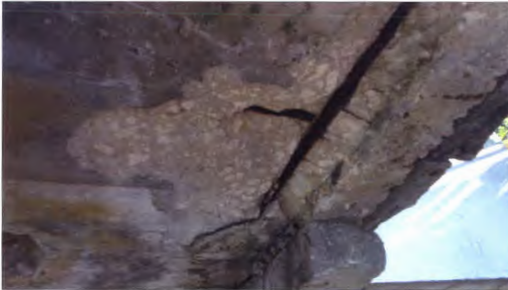
Rusting rebar breaking up concrete
