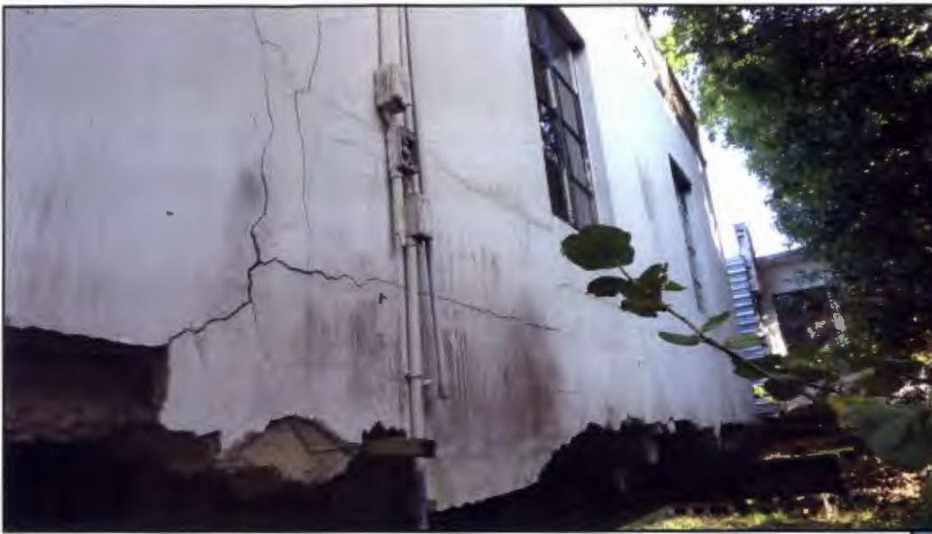
Foundation Cracking and large parts falling off
