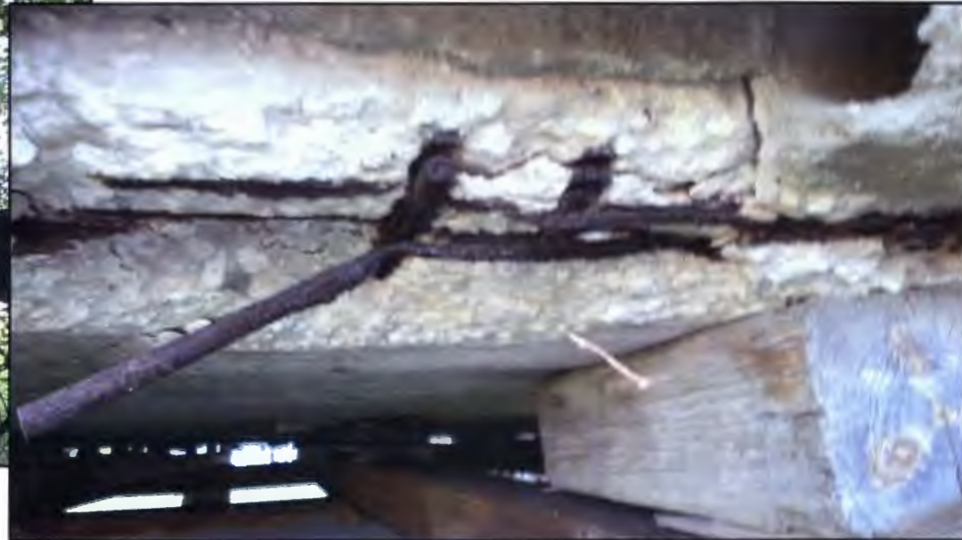
Floor Cracking and falling off
