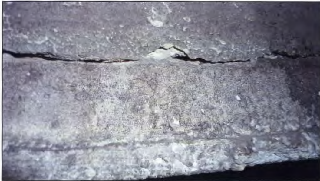
Major grade beam crack 2
