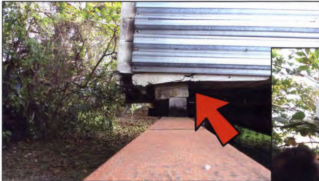
East foundation cracking and falling off
