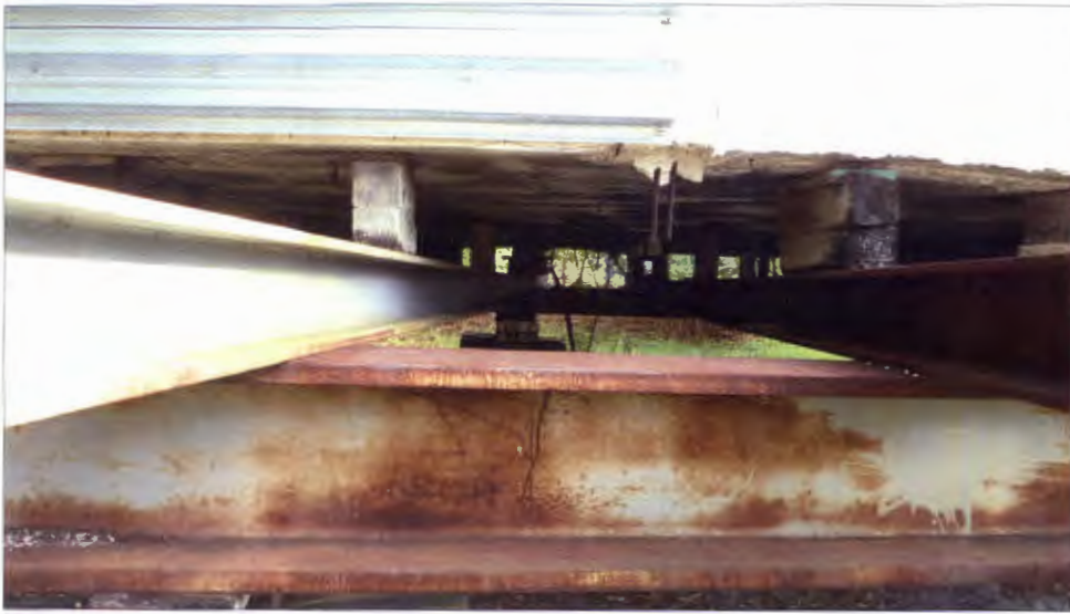
More bending of the steel over time
