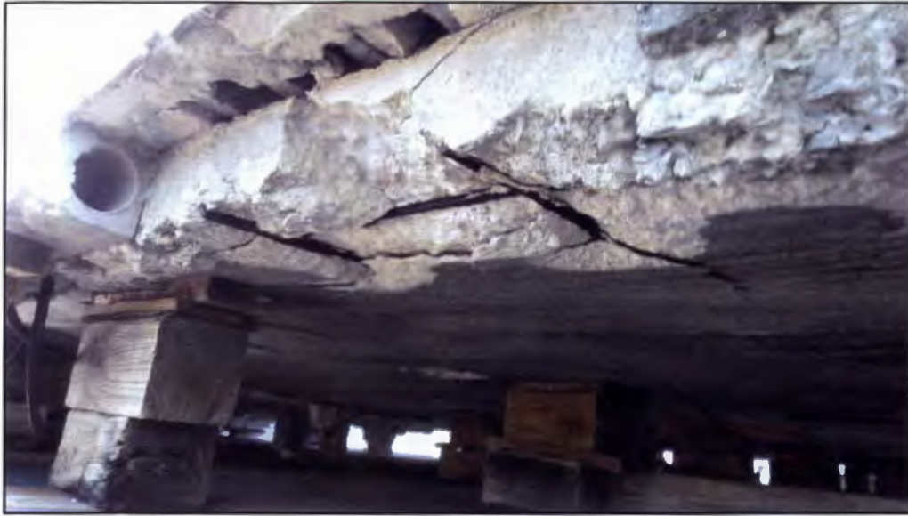
Foundation sprawling and wall and floor separated
