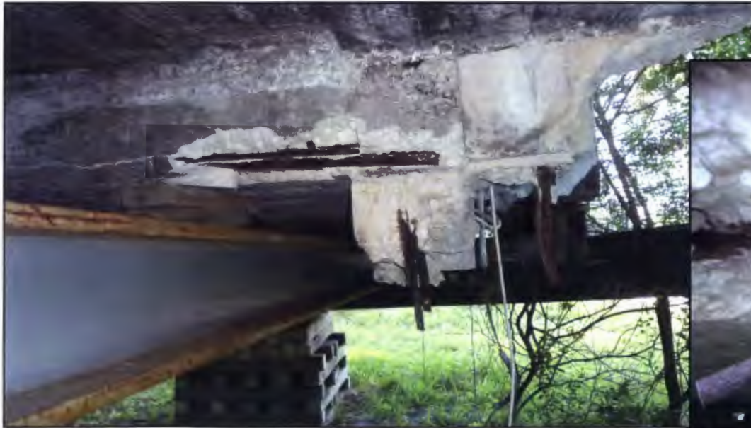
Foundation Cracking and parts falling off
