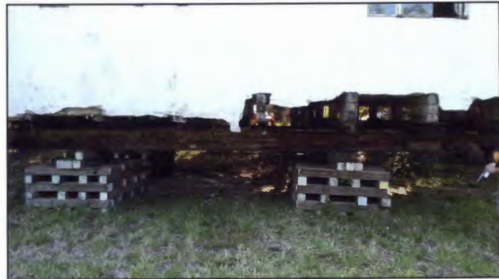
Wood supports starting to fail
