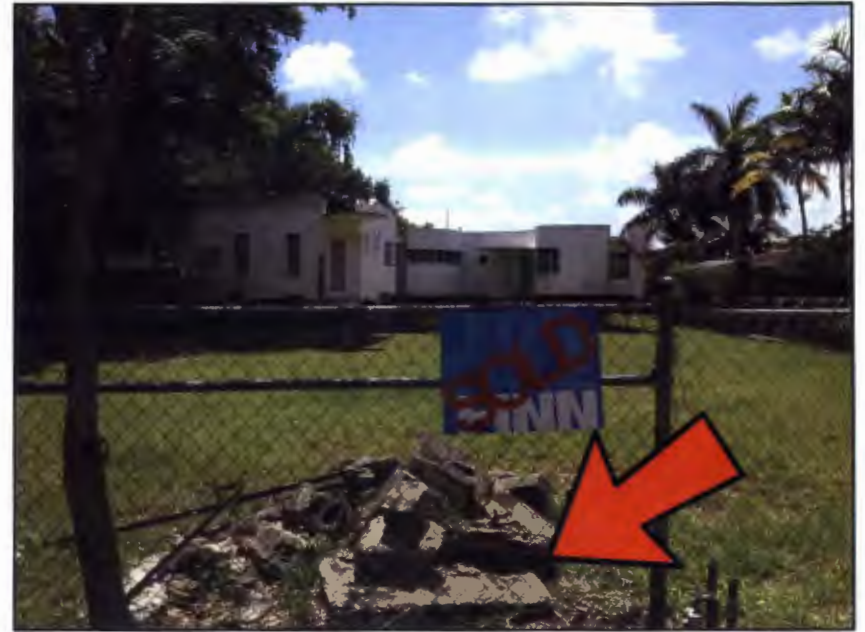
Past chunks of concrete that have fallen off.
