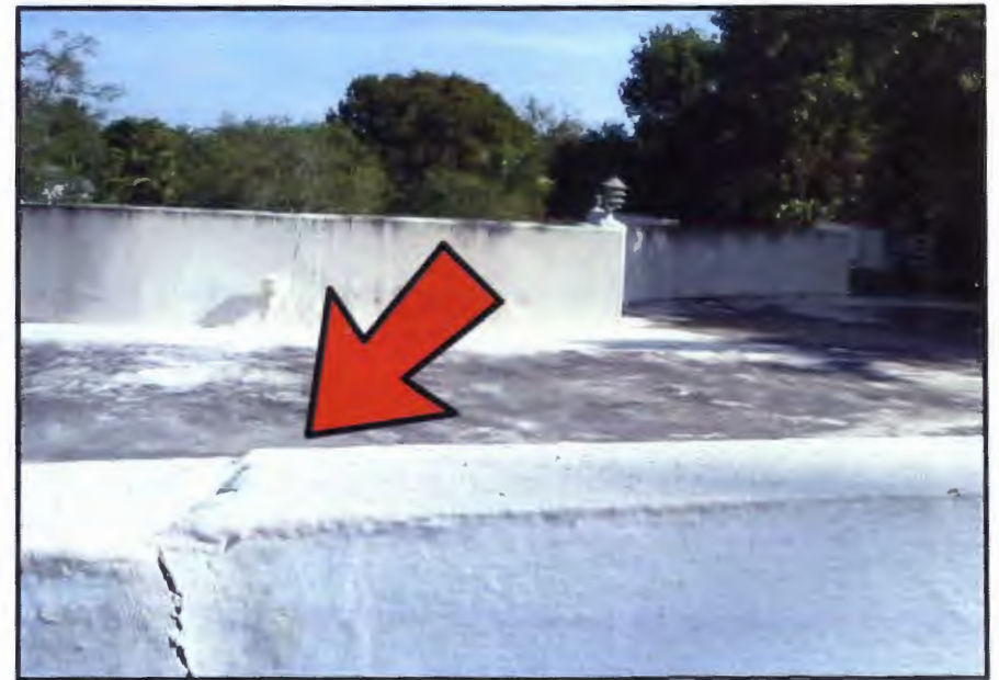
Major Wall Separation
