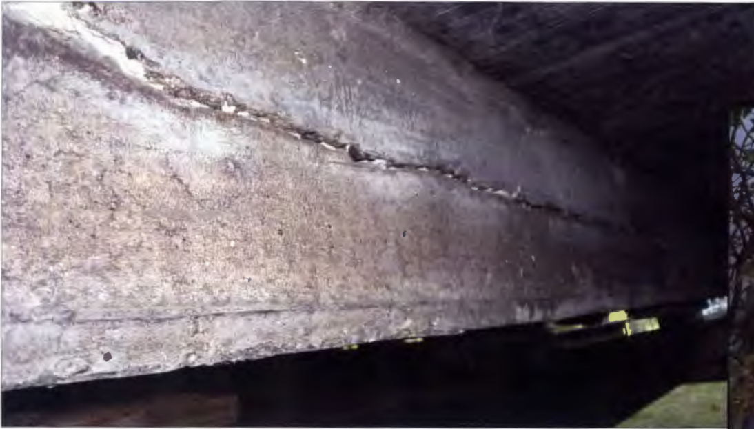
Major grade beam crack
