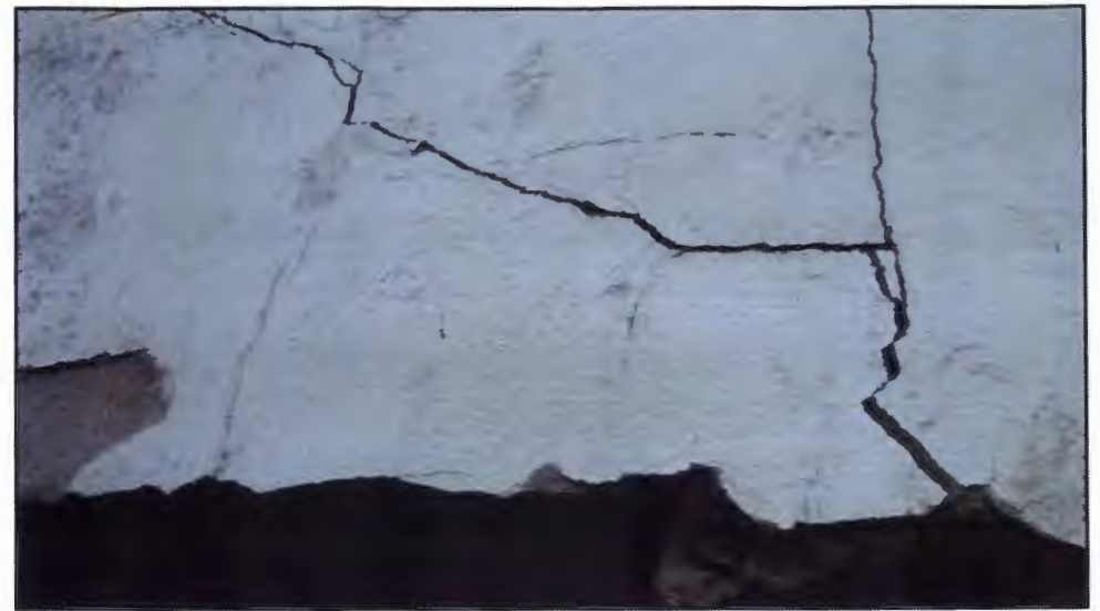
Deep Structural Wall cracks with pieces falling off
