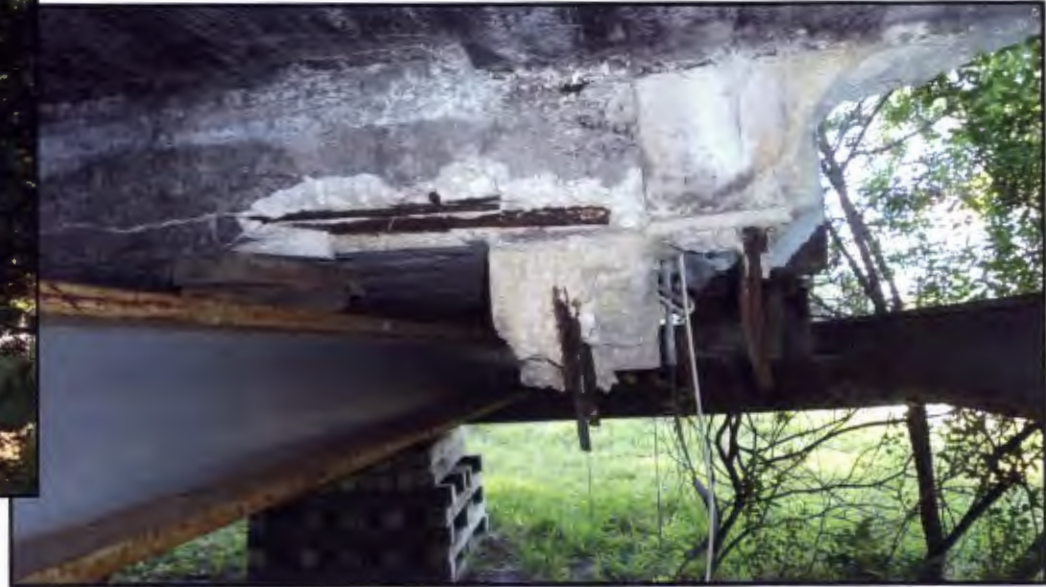
Foundation Cracks/ Parts Falling off
