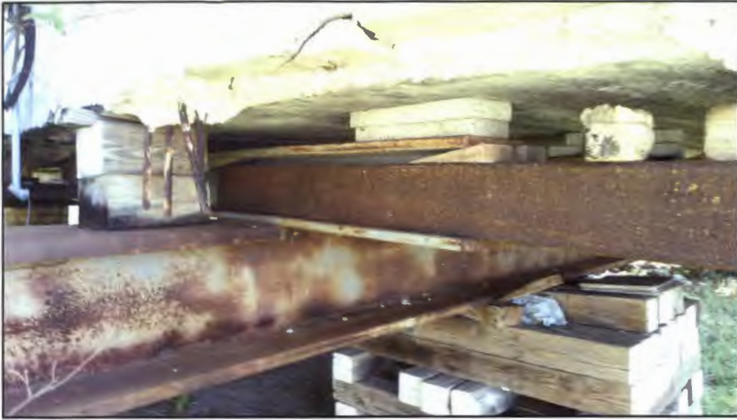
Unsafe Beam Extensions causing the cracks to get worse
