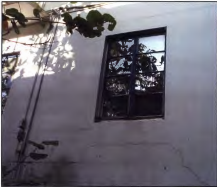
East wall Cracking
