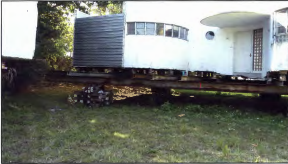
Home cut in half- View from front yard
