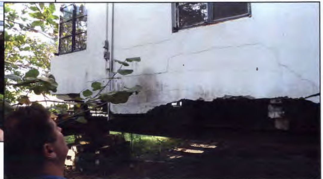
East Wall cracking to point of windows breaking.
