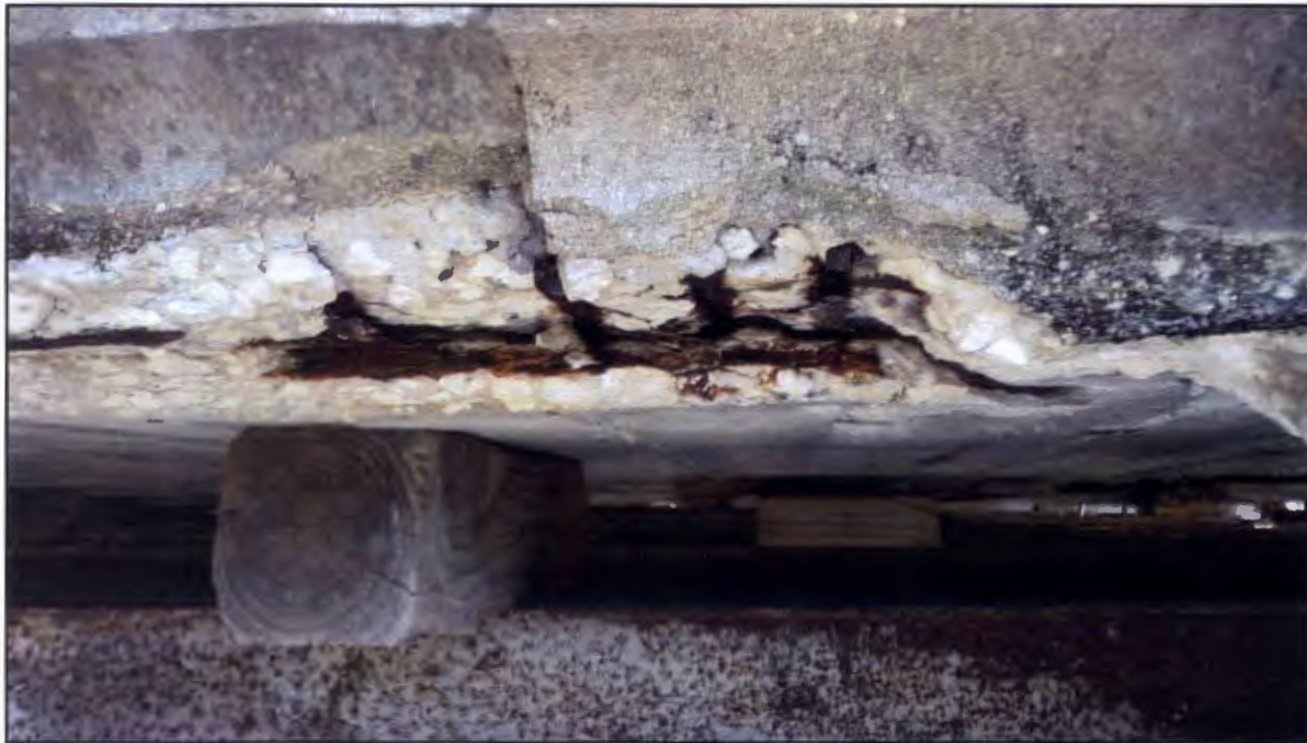
Major cracks in foundation
