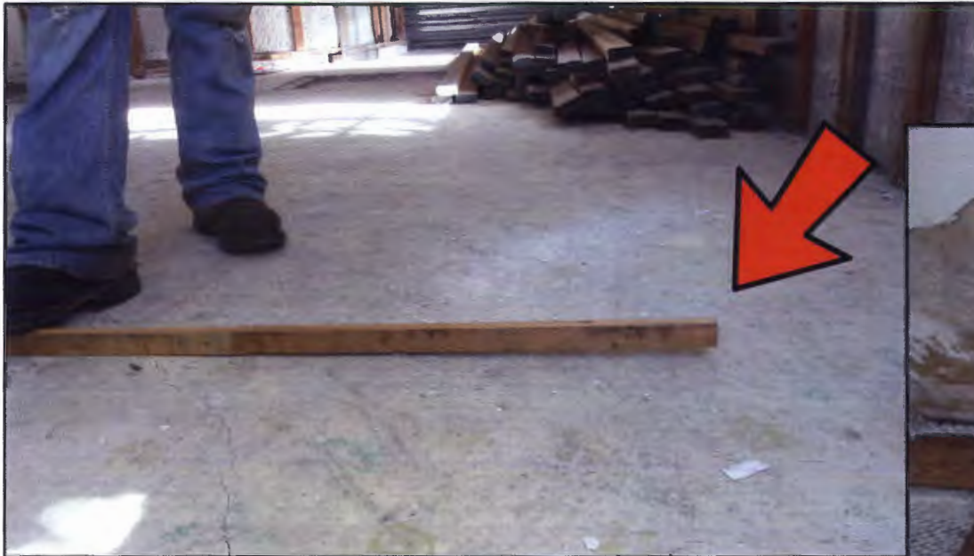
Floor cracked and falling
