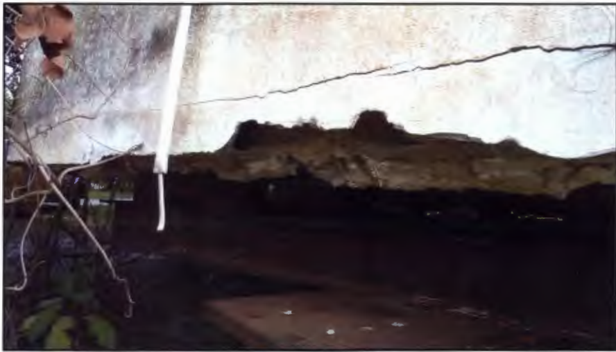
Chunks falling off of building
