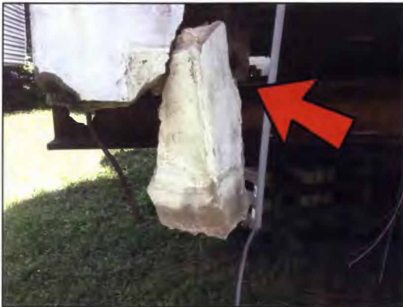
Large chunks falling off.
