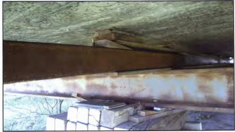
Unsafe Beam Extensions
