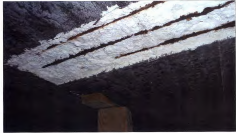
Test area rusted rebar
