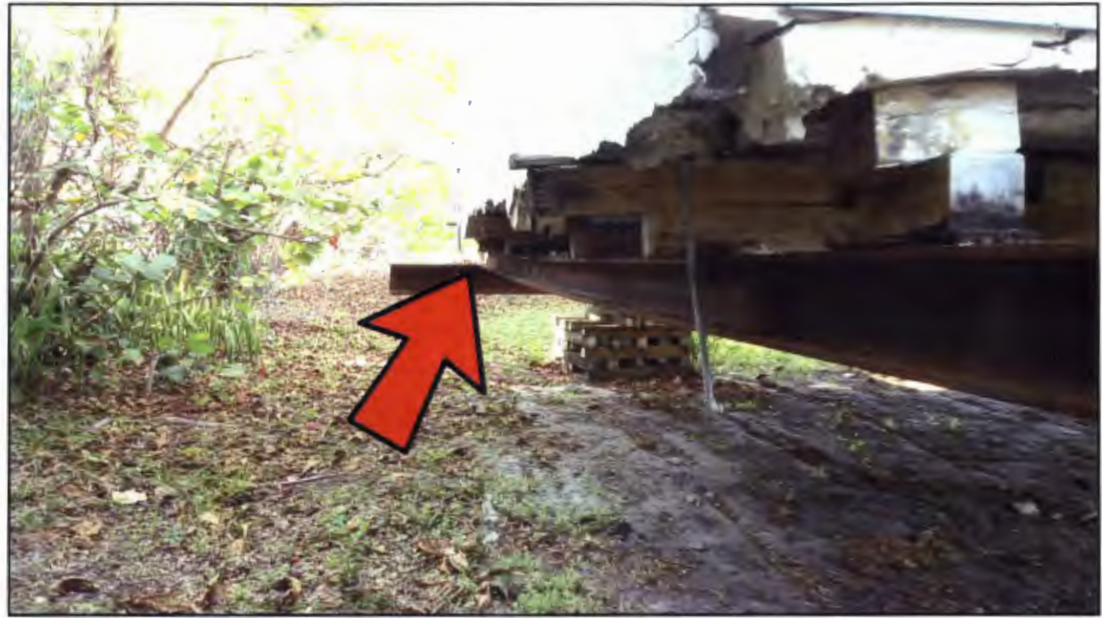
East side bowing under stress and cracked foundation and wall
