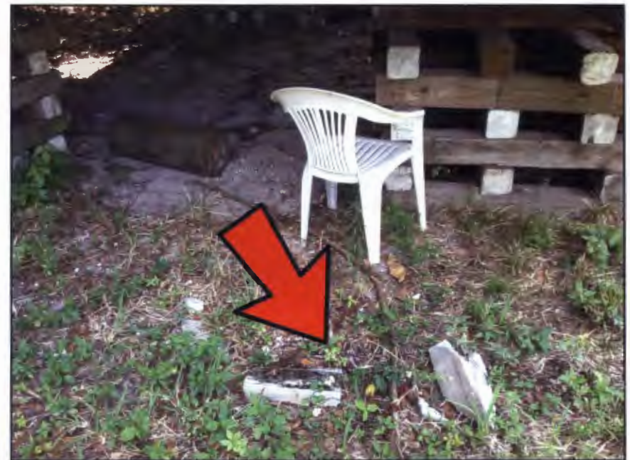
Vagrant hangout with chunks of concrete that have recently fallen off.
