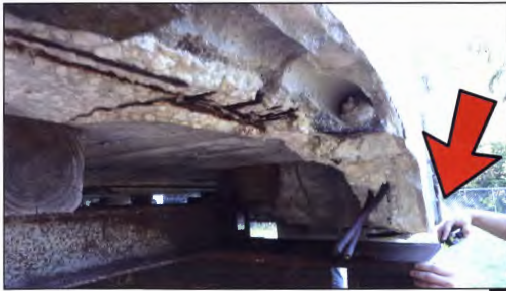
Foundation pulling away from wall
