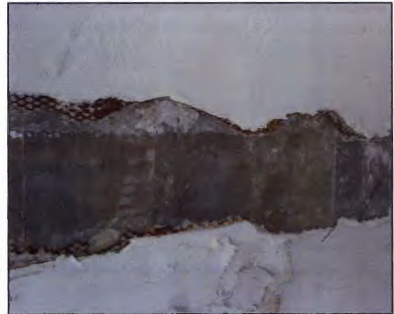
Ceiling cracking where walls were removed 8 years ago
