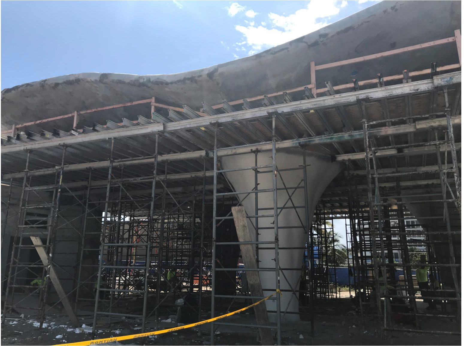
OCEANSIDE PARK PROGRESS PHOTO TAKEN ON 9-11-2019 (SHADE CANOPY – FORMWORK AND SCAFFOLDING BEING REMOVED AND CONCRETE FINISHING ONGOING)
