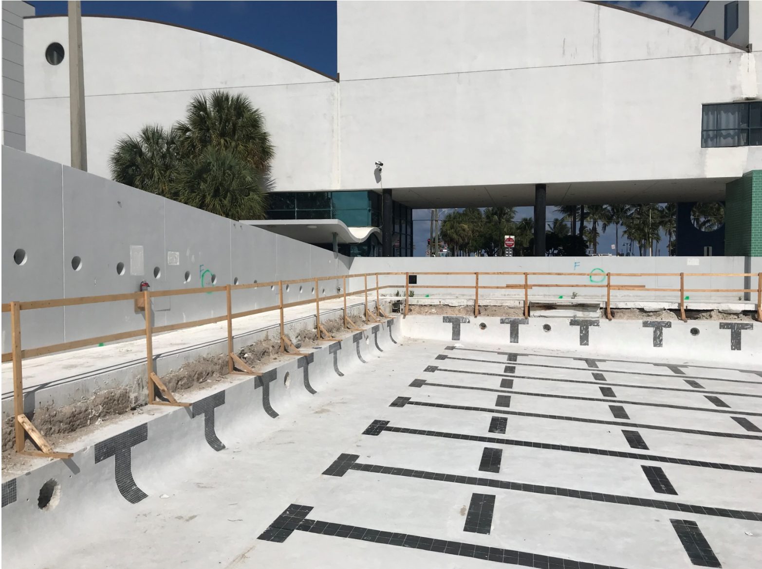
AQUATIC CENTER PHOTO TAKEN ON 9-10-2019 (FACING EAST – TRAINING POOL - GUTTER AND PLUMBING REMOVED)
