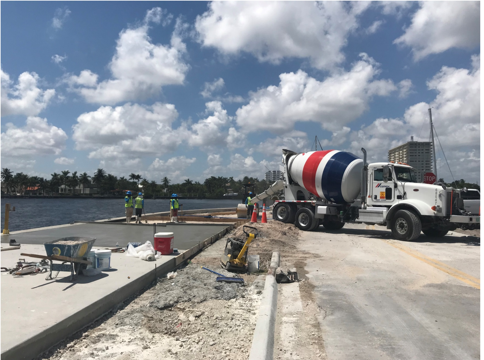
SOUTH PARK PROGRESS PHOTO TAKEN ON 9-11-2019 (SOUTH SIDE OF MARINA PROMENADE FACING WEST)
