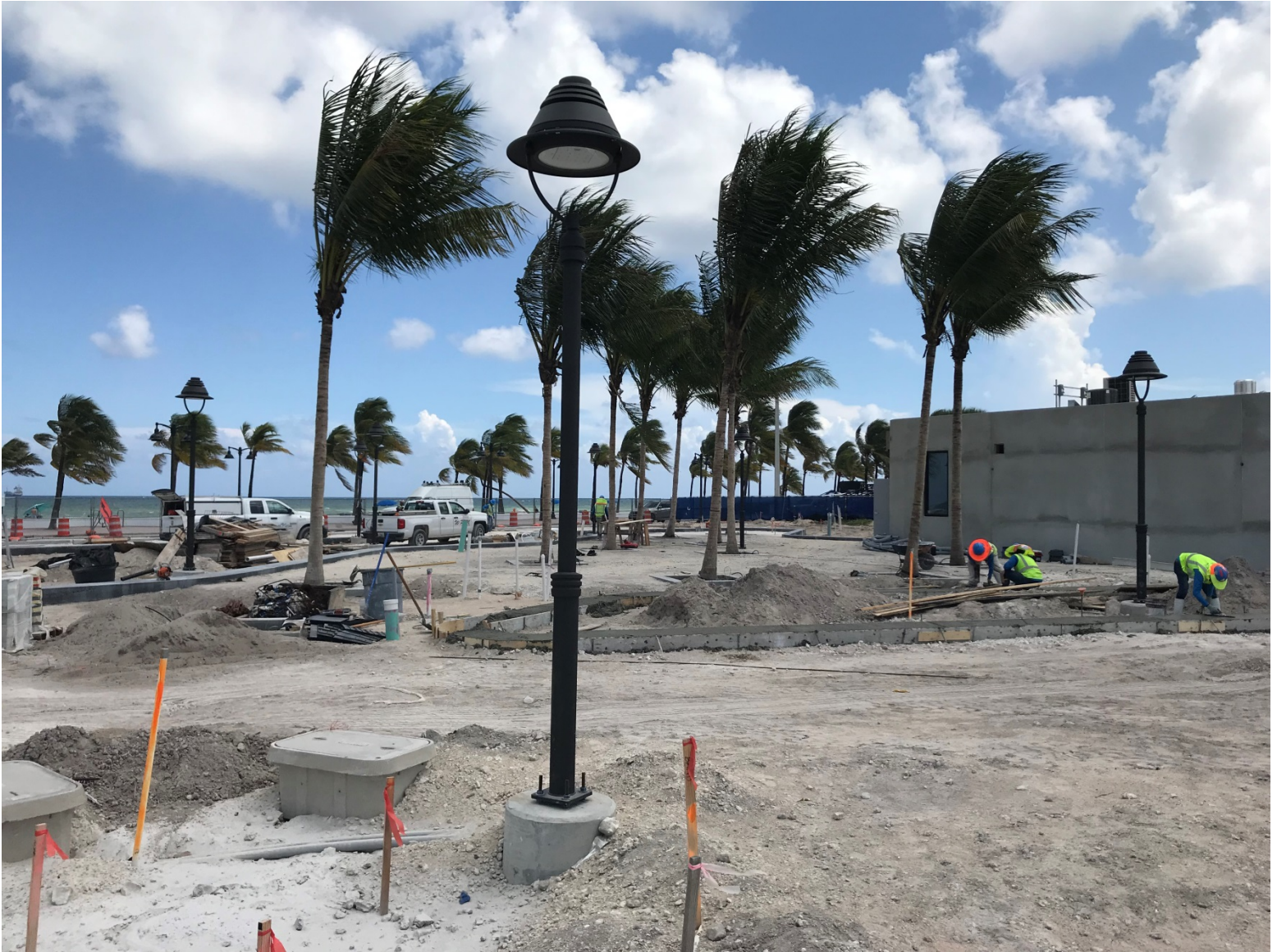
OCEANSIDE PARK PROGRESS PHOTO TAKEN ON 9-11-2019 (EAST SIDE OF PARK FACING SOUTH)
