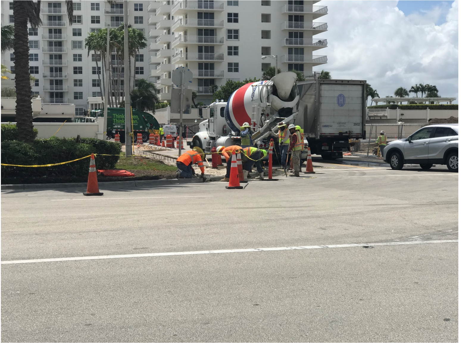
SOUTH PARK PROGRESS PHOTO TAKEN ON 9-12-2019 (LAS OLAS CIRCLE FACING SOUTH – CURB AND GUTTER CONCRETE POUR)
