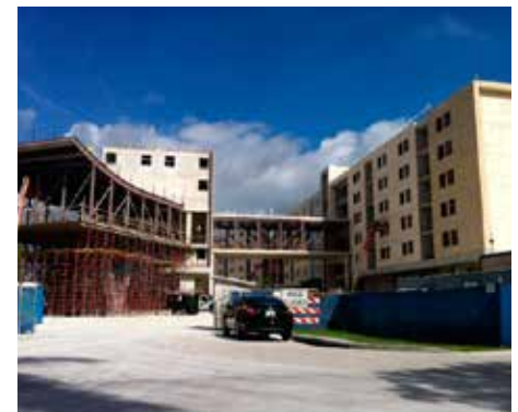
Atkins developed detailed cost estimates for the design development and permit documents for the Parkview New Student Housing Complex.
