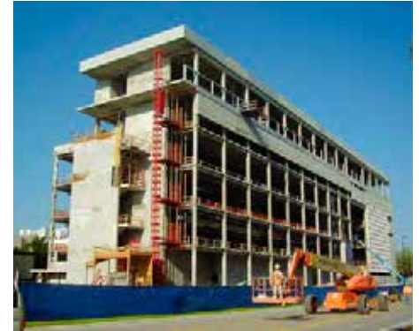
Atkins developed cost estimates and reviewed the construction manager's GMP submittal for the New Science Classroom Complex.
