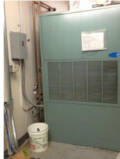
20 year old VVT Air Handling Unit which has had dampers disabled.
