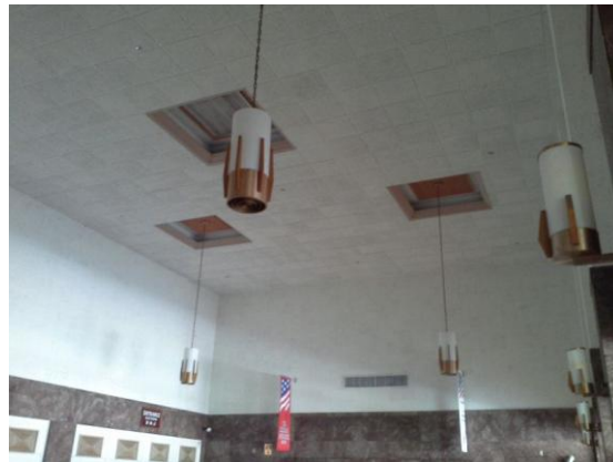
Incandescent Fixtures in Lobby
