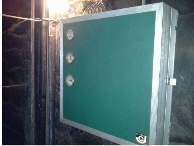
Old Pnuematic HVAC Controls
