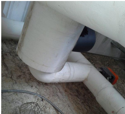
Typical 3-way valve at AHUs
