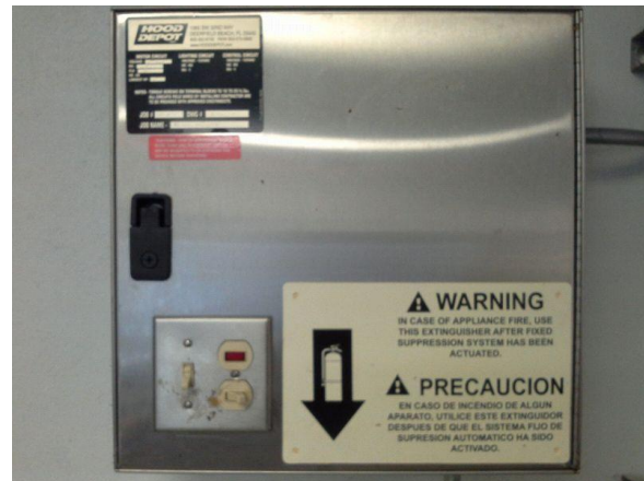
Manual Hood Controls
