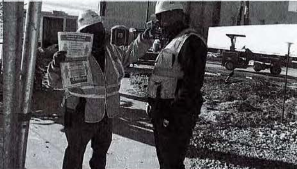
All Workers Must Be Temperature Checked and Advised Of COVID-19 Protocols at the Site Gate and Building Entrance.
