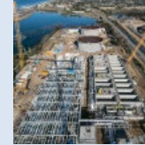
Claude "Bud" Lewis Desalination Plant IDE Technologies & Kiewit City of Santa Barbara, CA
