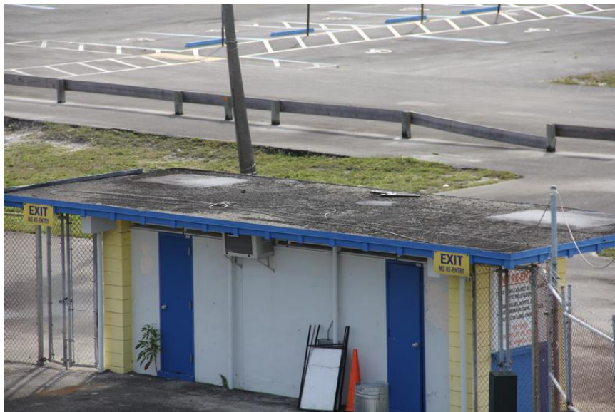
View of the deteriorated modified bituminous roof.
