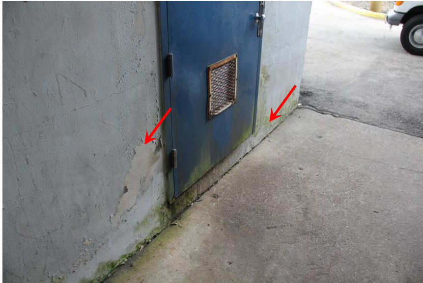
View of failing paint.
