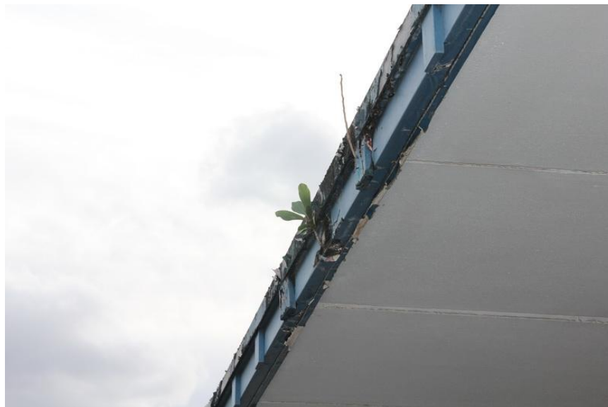
View of typical deteriorated roof edge flashing.
