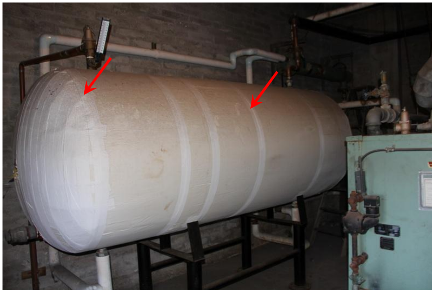
View of tank, which appears to have aged beyond its service life.
