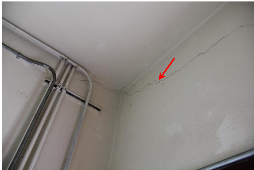
View of typical interior cracking.
