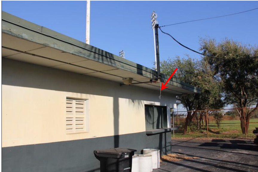
View of loose electrical wire.
