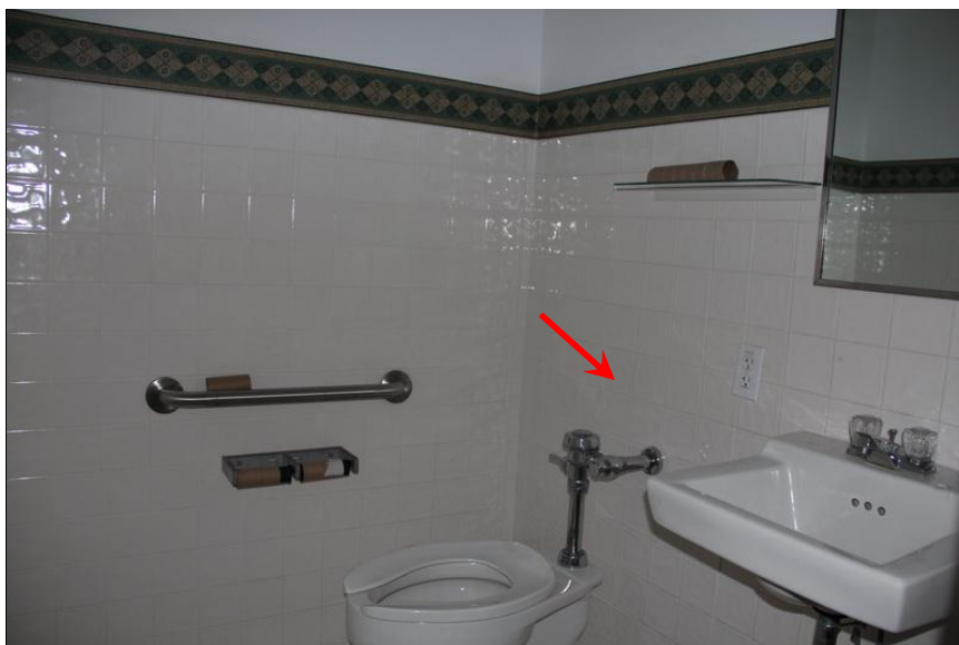
View of ADA restroom with missing grab bar.
