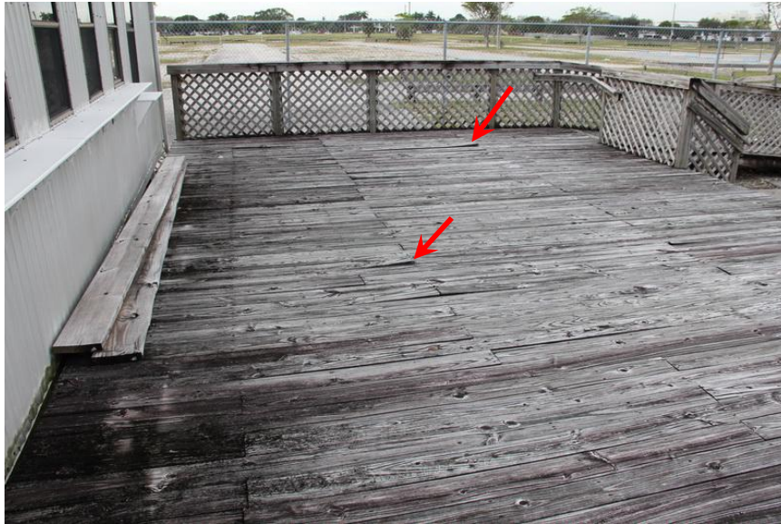
View of warped floor boards.
