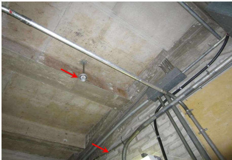
View of single light fixture in electrical room, poor lighting in room (this single fixture does not work) a fluorescent fixture above the phone board is the only working room light fixture. The above picture also shows cable not in conduit, example of one of several cables that penetrate room not in conduit.
