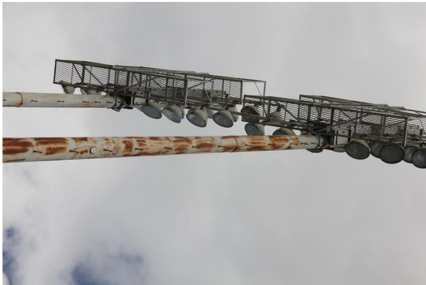
View of typical corrosion staining and missing paint on the stadium light poles.
