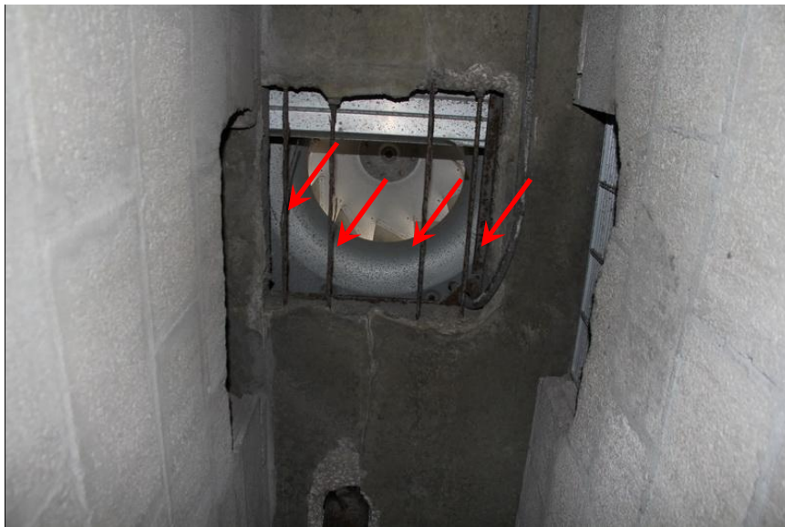
View of exposed reinforcing bars.
