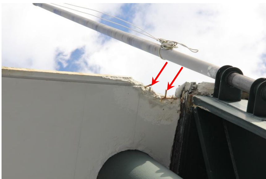
View of the spalled concrete at the awning edge. Exposed reinforcing bars are evident.
