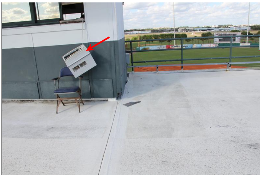
View of HVAC hanging by the cord.
