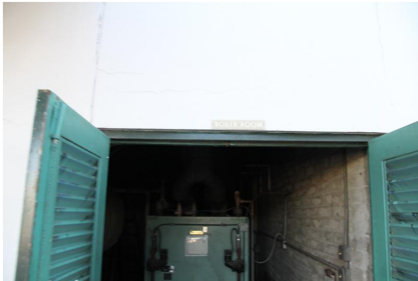
View of the Boiler Room entrance
