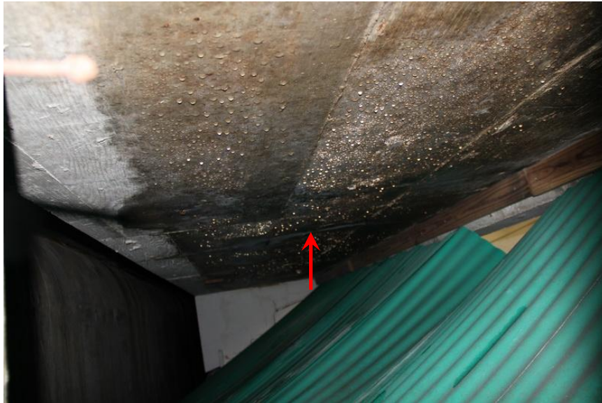
Typical view of moisture intrusion.
