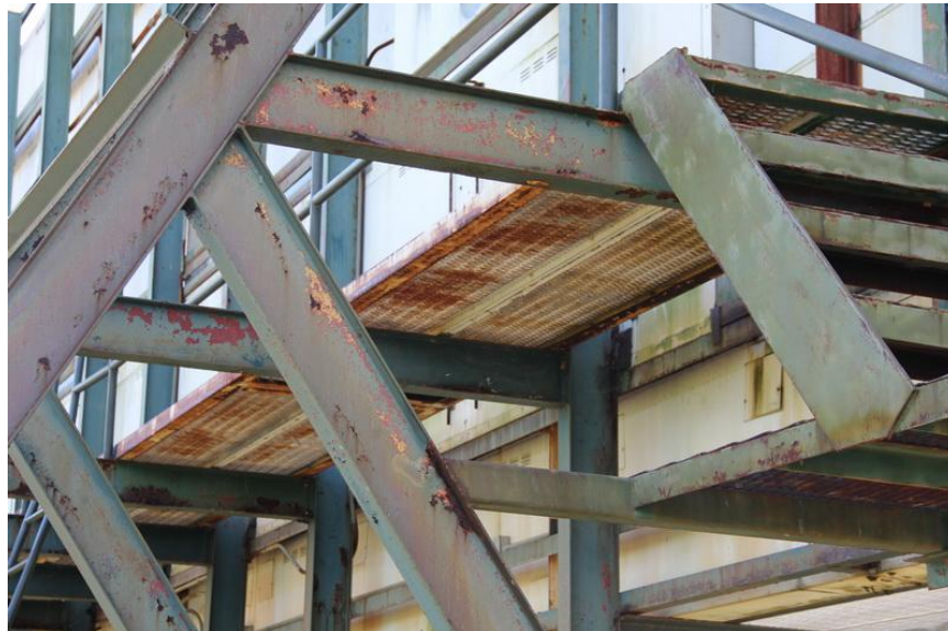
View of typical paint delamination and excessive corrosion staining on scoreboard framing.
