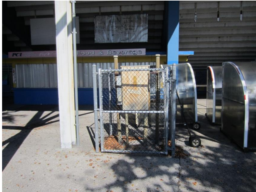
View of equipment disconnect and receptacles near the south concessions building which lacks labels.
