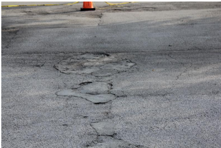
View of excessively deteriorated pavement areas which will require asphalt pavement removal and replacement.
