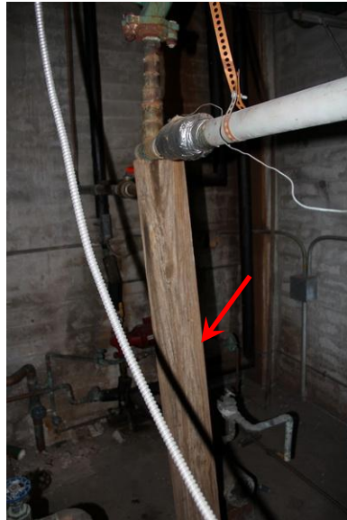
View of improper pipe support system.
