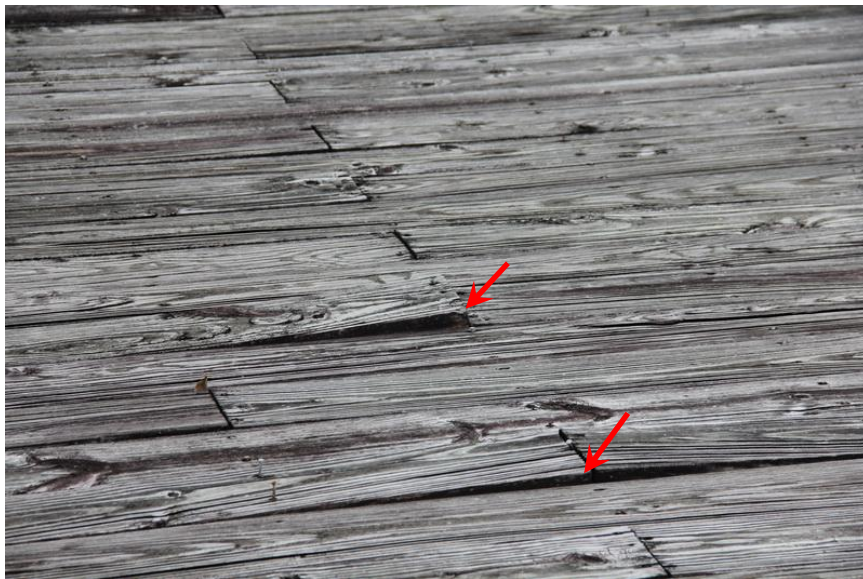
View of warped floor boards.
