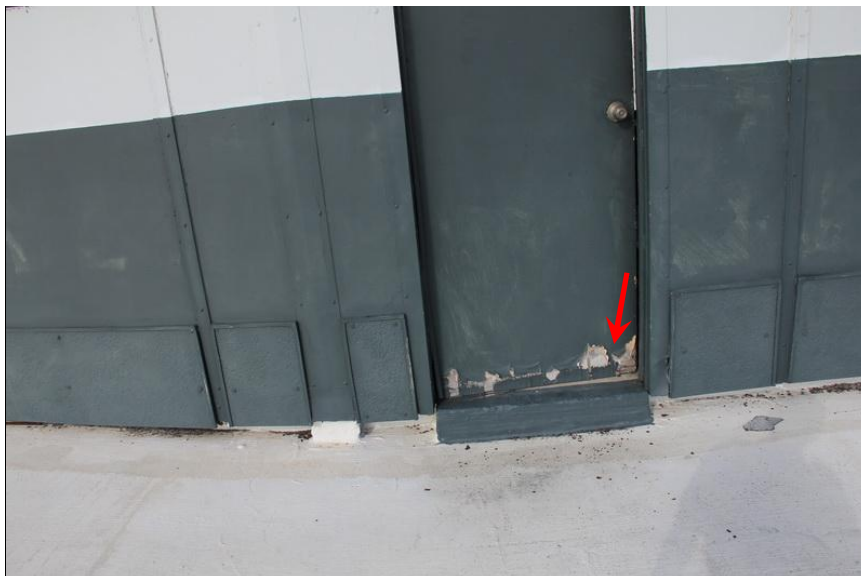
View of damaged door.
