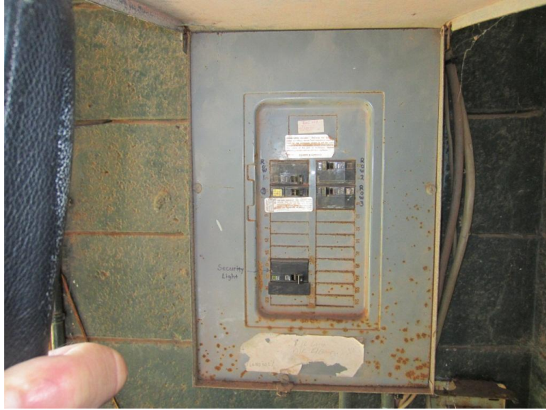
View of rusting panelboard located in the right field bull pen; a NEMA 3R rated enclosure should have been used here because the panel's location; replacement is recommended.
