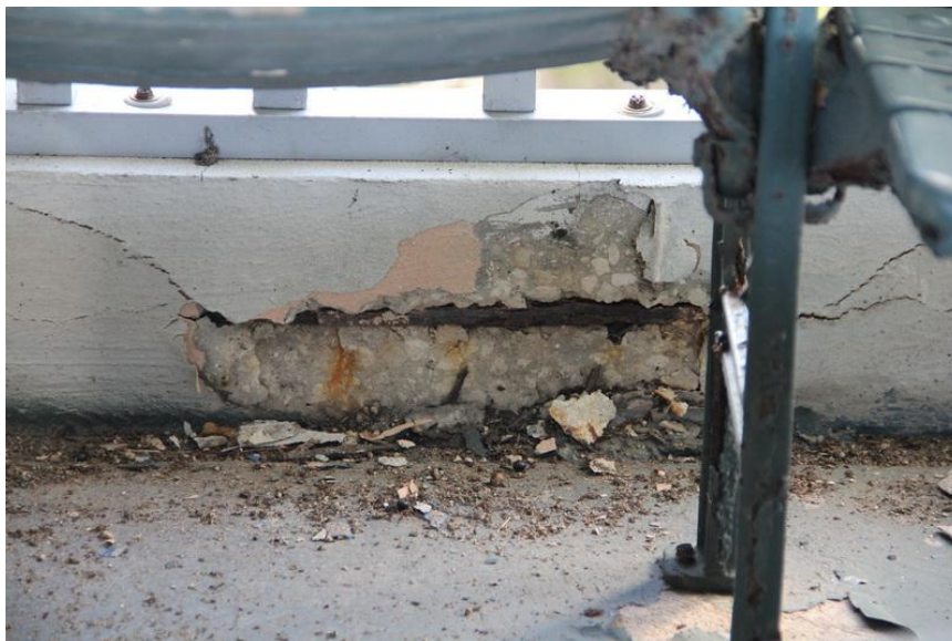
View of typical concrete spalling and exposed reinforcing bars at the top level of the stadium seats.
