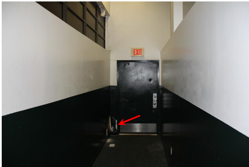
View of kicked in wall near exit.
