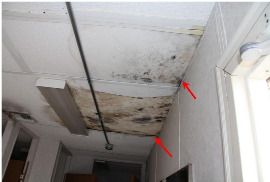
View of water intrusion/mold on interior ceiling.
