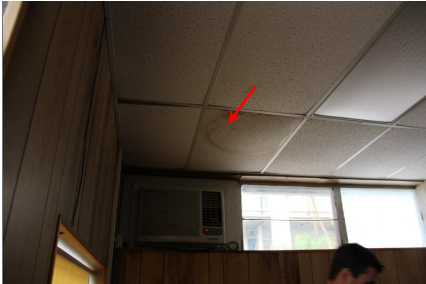
View of water intrusion.
