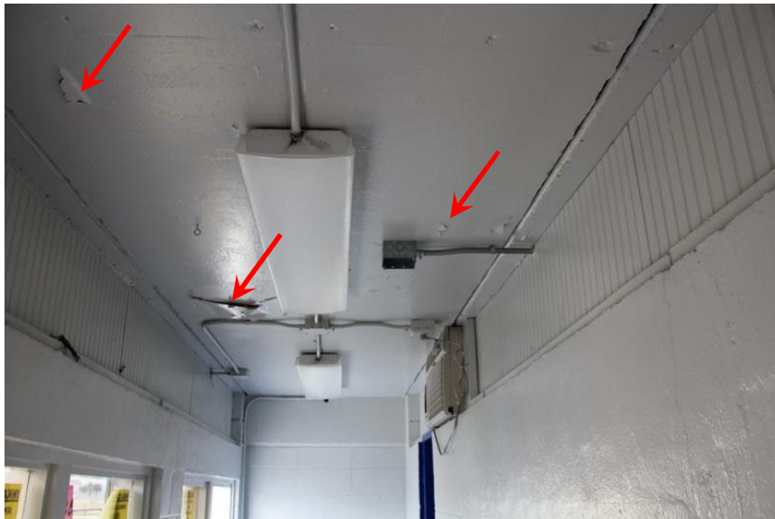
View of ceiling paint issues.
