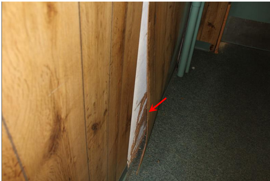
Typical view of delamination of wood panels.
