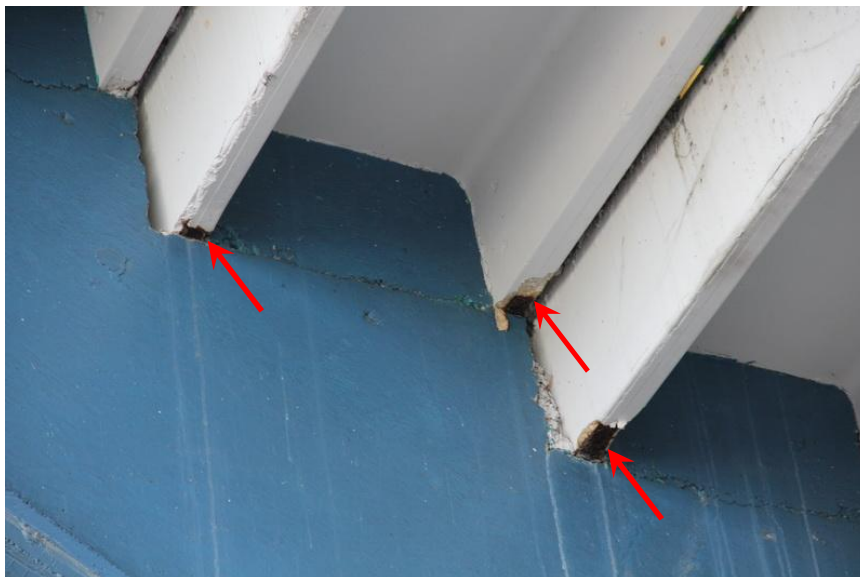
View of Corroded metal bearing plates on the double-tee concrete beams.
