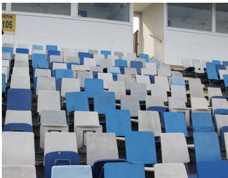
View of the Plastic and Wood seats that need removed and replaced.
