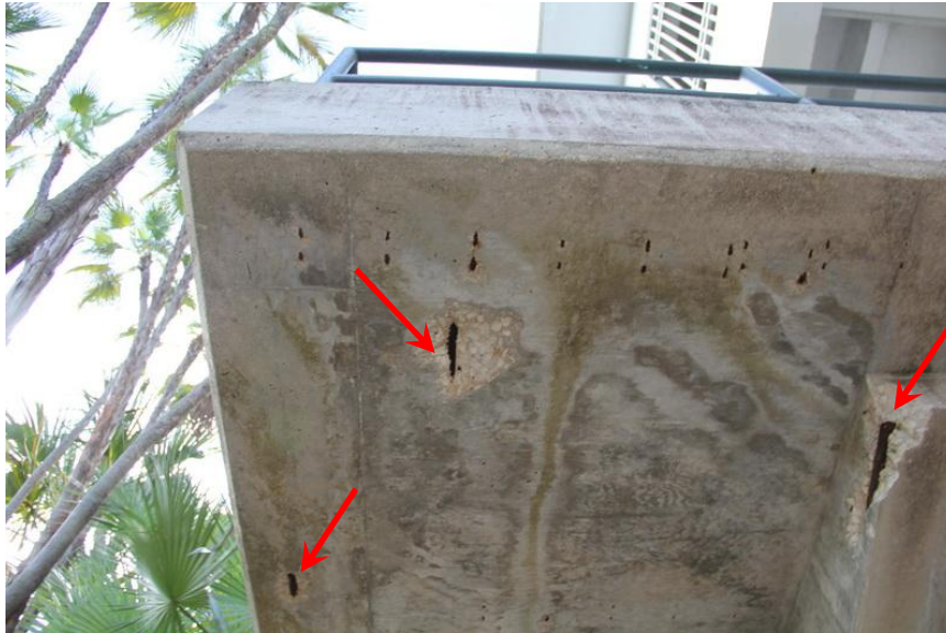
View of typical spalled concrete and exposed reinforcing bars in the underside of the stadium access ramps.
