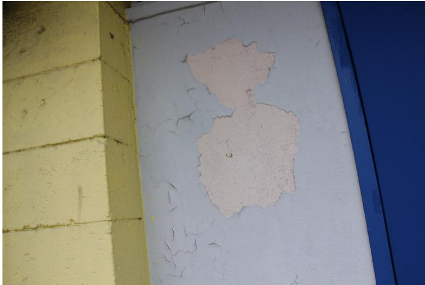
View of typical exterior paint issues.
