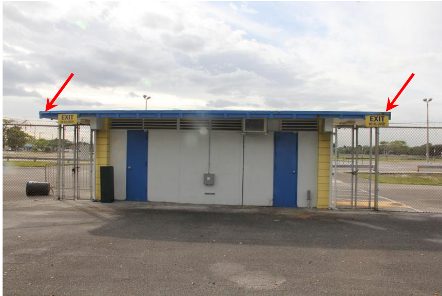
View of damaged roof edge flashing.
