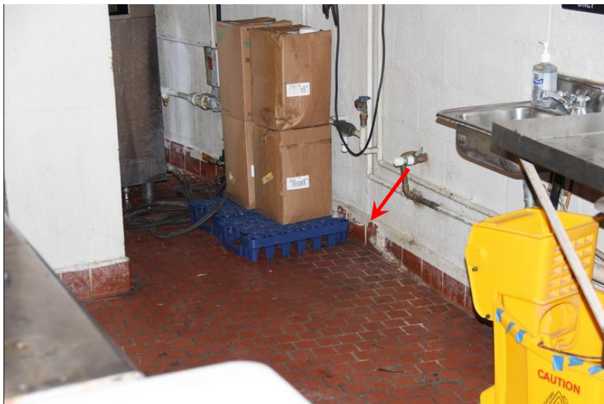
View of deteriorated tile.
