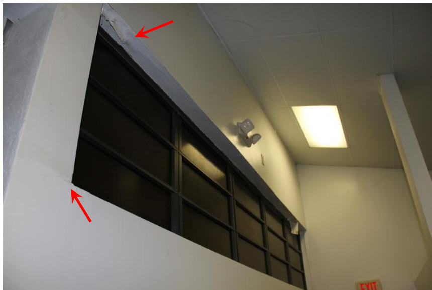
Typical view of both peeled paint and cracks at window corners.
