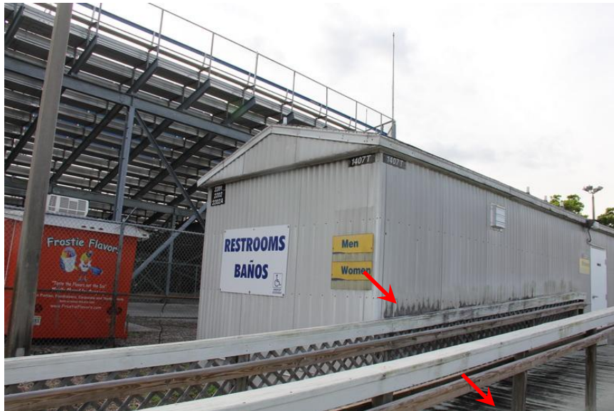
View of Wood Ramp and mold on building.
