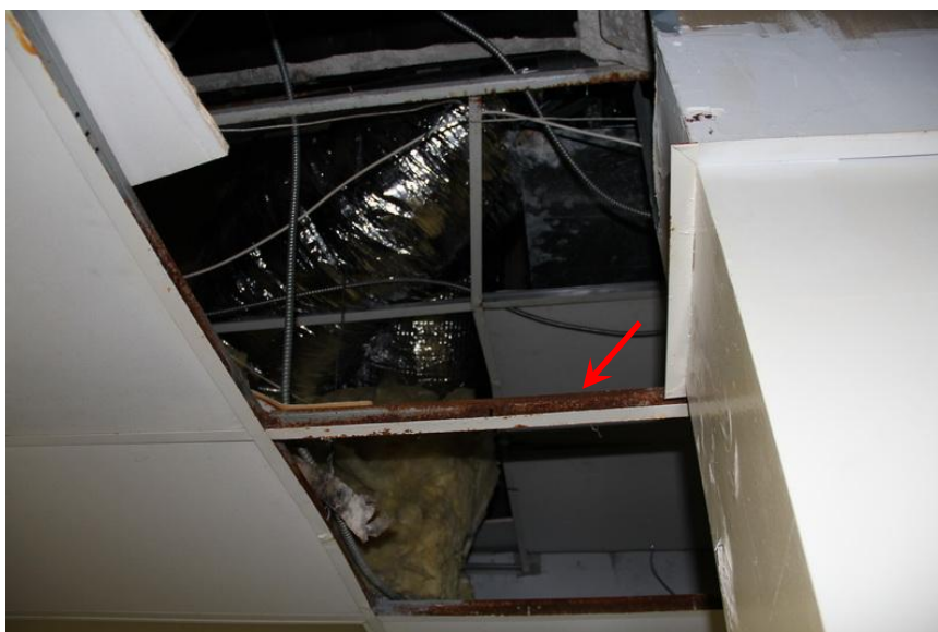
Typical view of metal frame corrosion.
