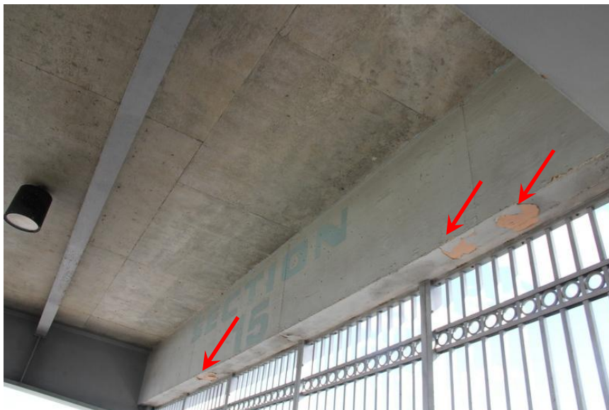
View of the chipping/fading paint along the seating section label portion of the awning.
