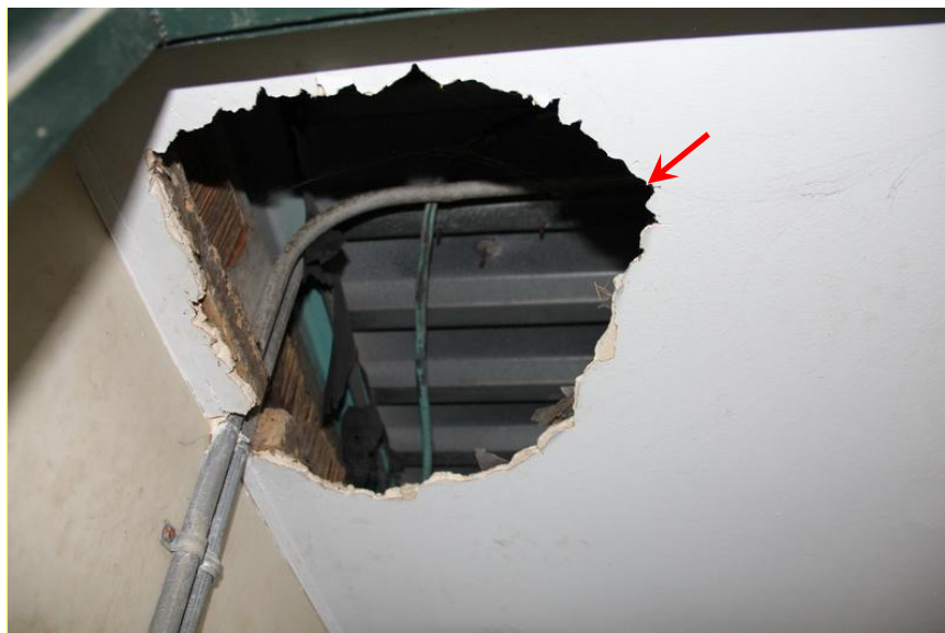
View of roof opening.
