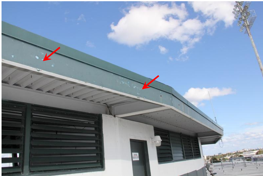
View of chipping/flaking paint on roof flashing.
