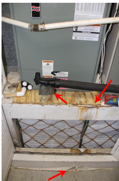
View of HVAC closet and base board damage.
