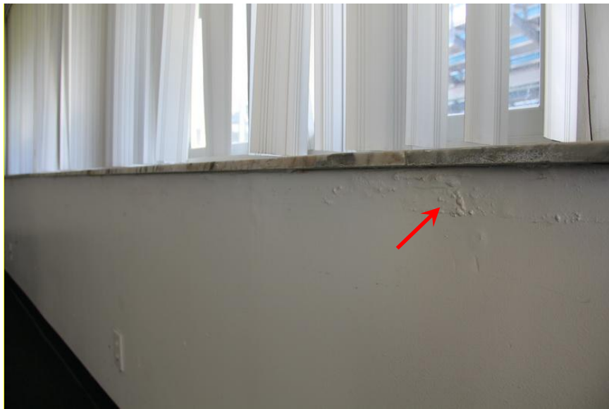
View of finished surface deviations.
