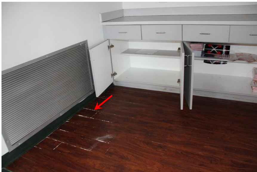
View of damaged floor boards.
