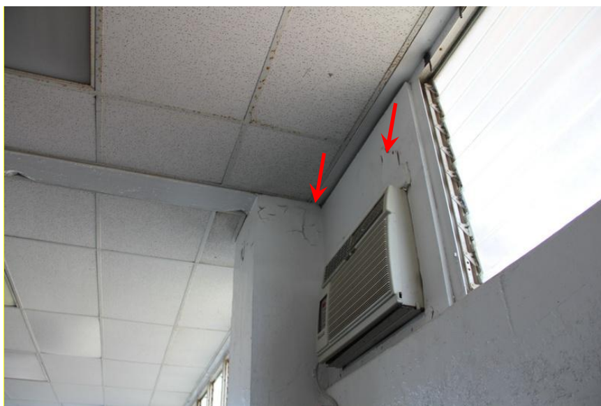
View of wall A/C unit and support column.
