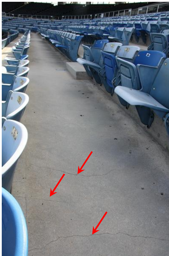
View of typical cracking in the seating concrete slabs.
