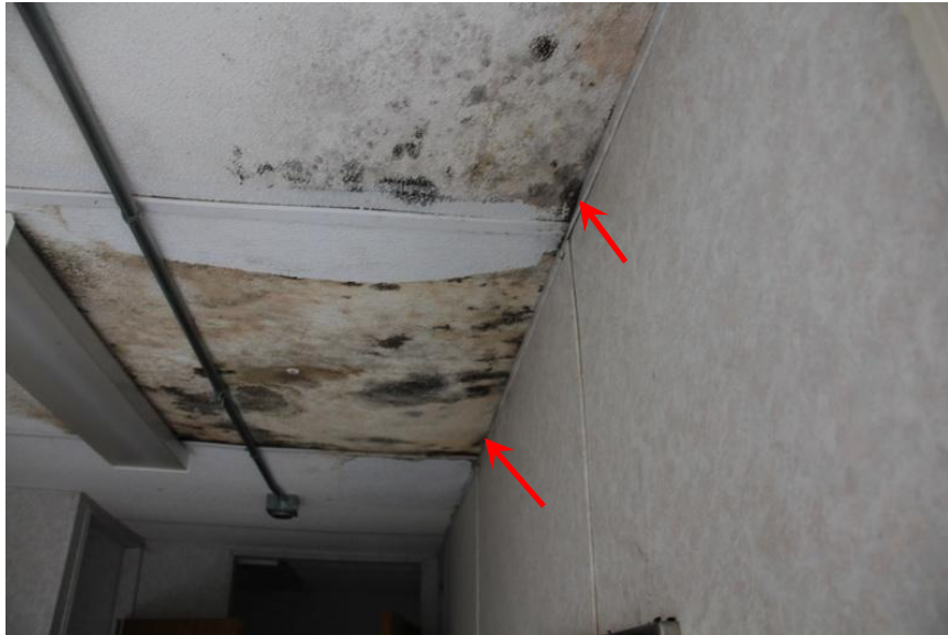
View of water intrusion/mold on interior ceiling.
