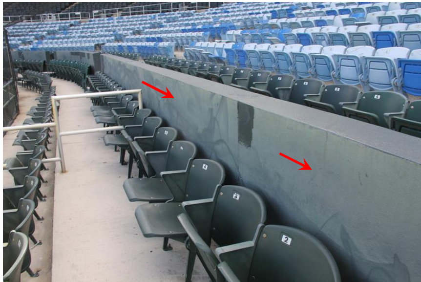
View of typical faded paint throughout the lower level perimeter wall.
