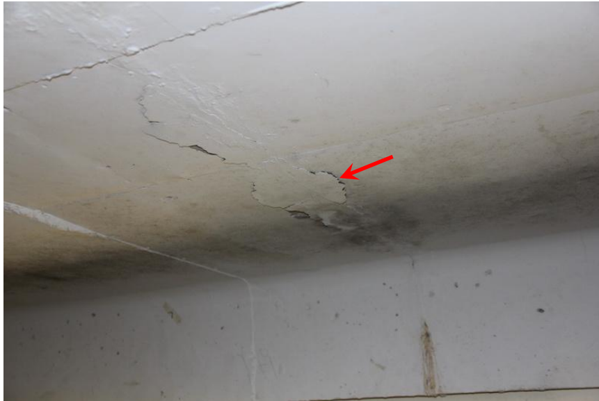
View of failing patch.
