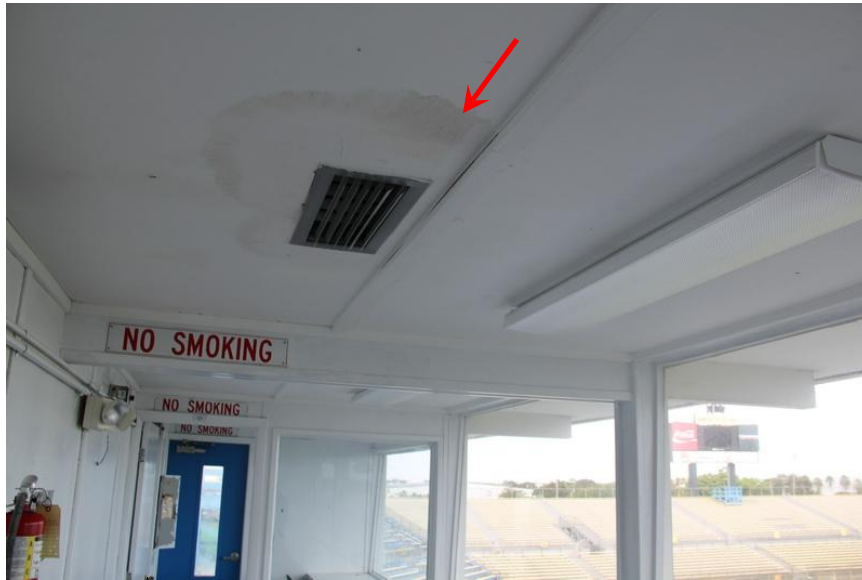
View of the Lower Press Box water intrusion.
