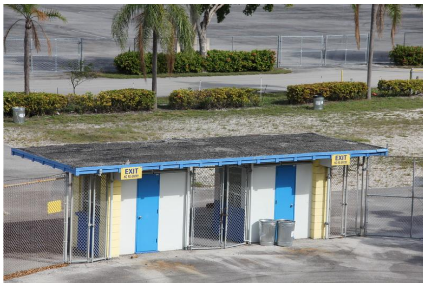
View of the deteriorated modified bituminous roof.
