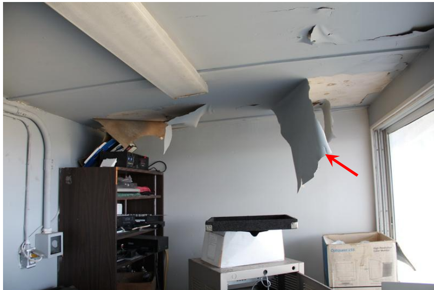
View of ceiling water damage.
