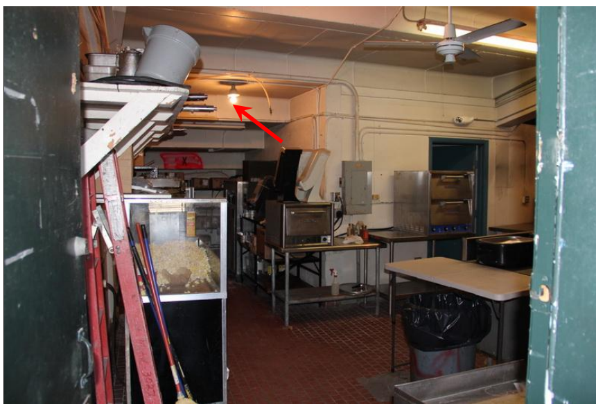
View of the missing light cover.
