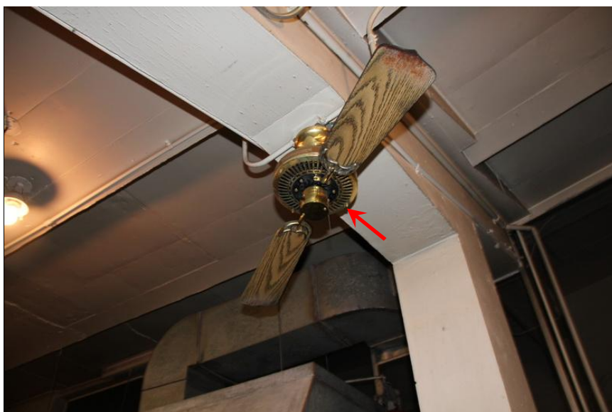
View of missing fan blades.
