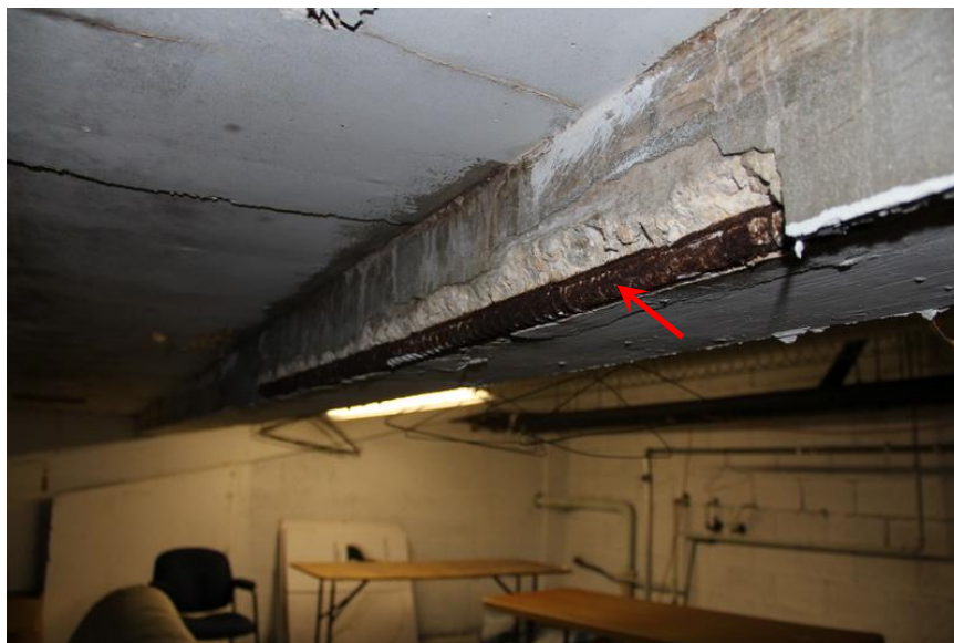
Typical view of exposed rebar.
