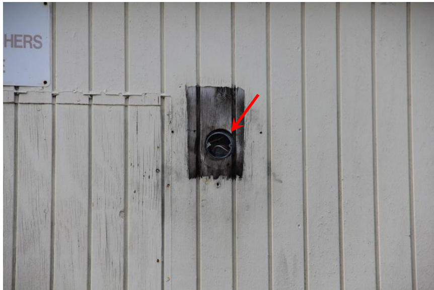
View of abandoned electrical opening.
