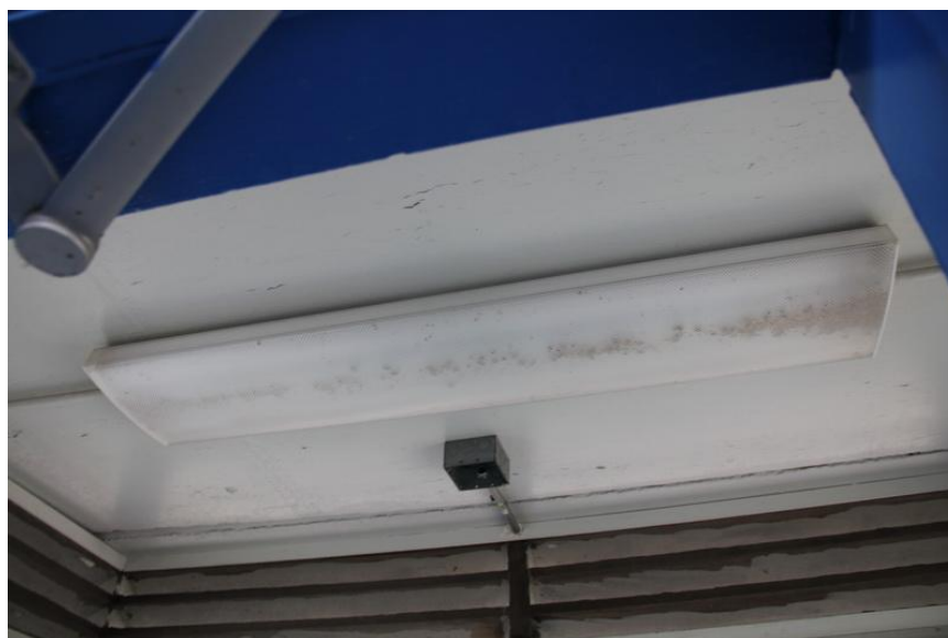
View of open electrical junction box.
