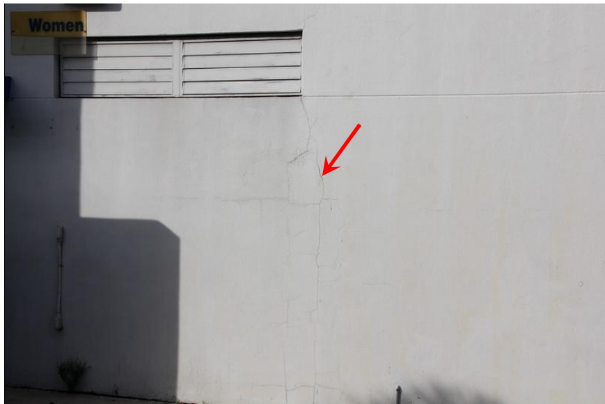
View of typical exterior cracking.
