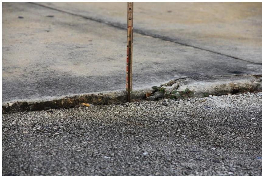
View of the 1-1/2" step from asphalt to concrete.
