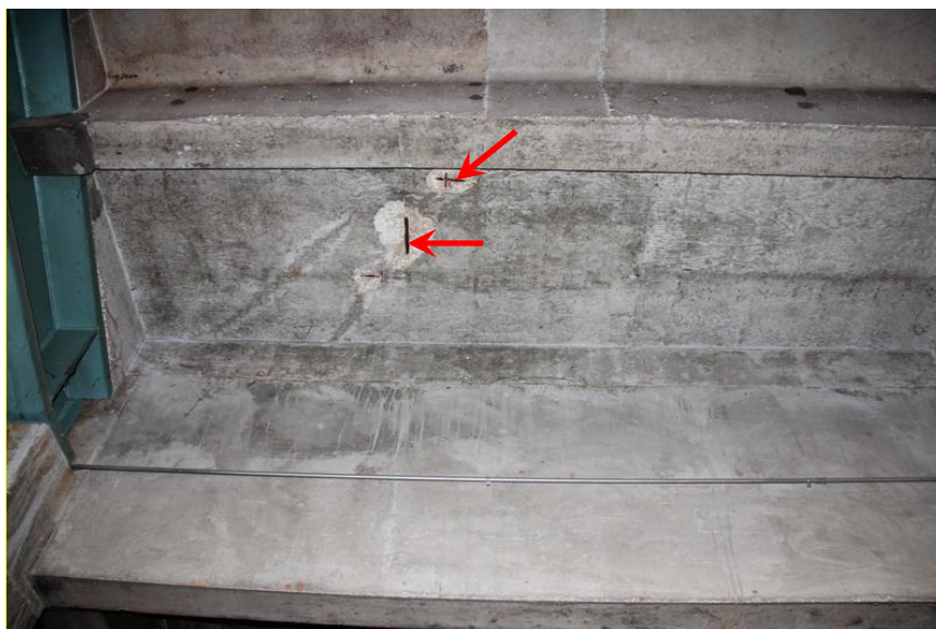
Typical view of the exposed rebar.
