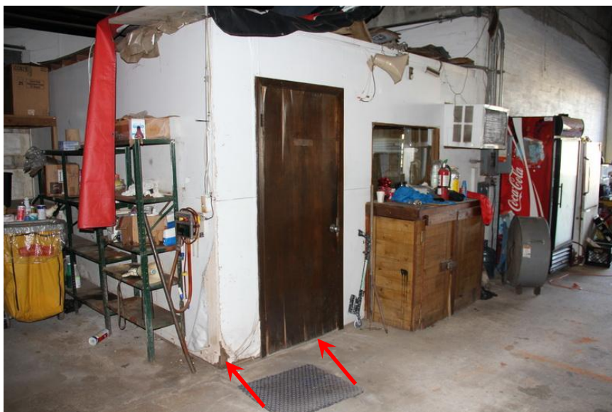
View of water damage to storage room.
