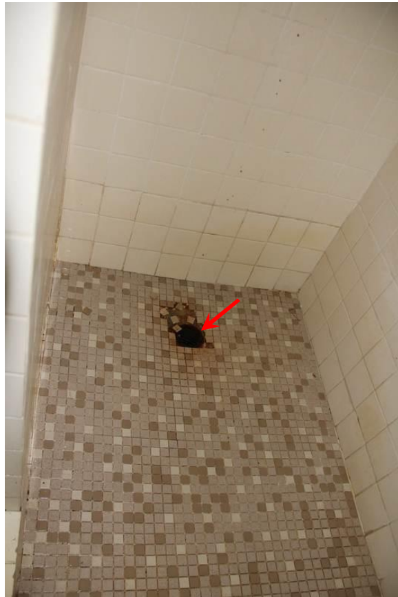
View of cracked tiles and corroded drain.
