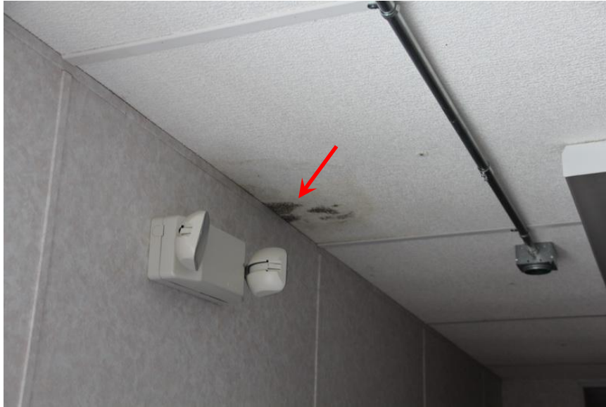
View of water intrusion at interior ceiling.
