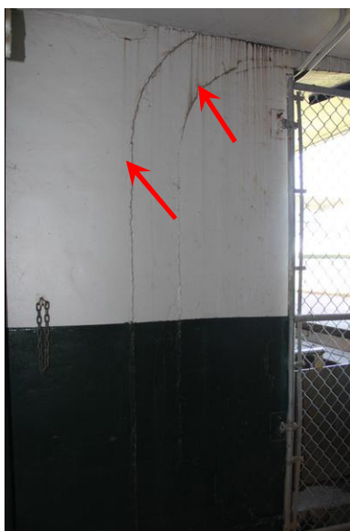
View of wall cracks.
