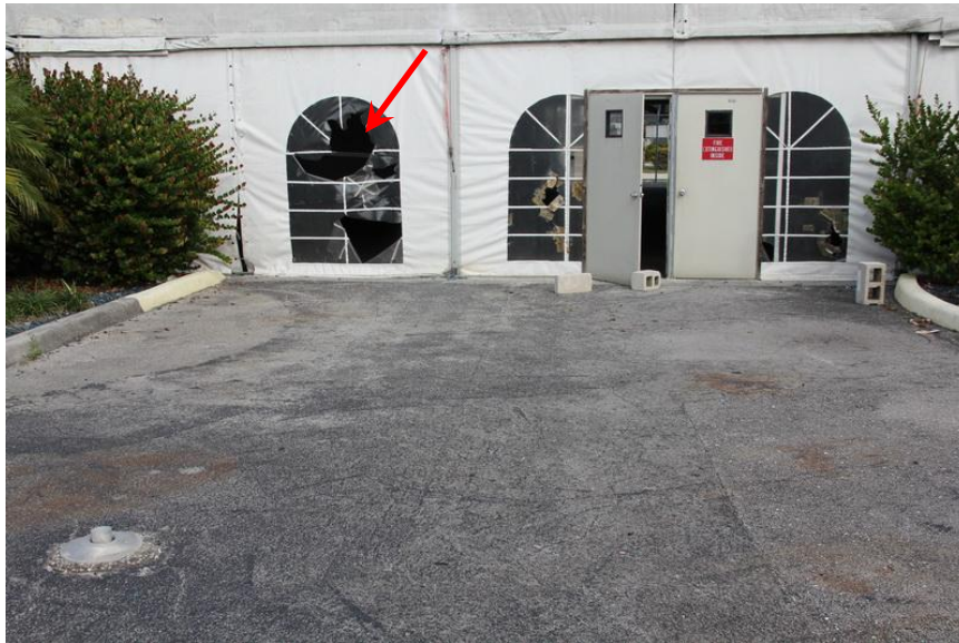
View of canvas wall deterioration.
