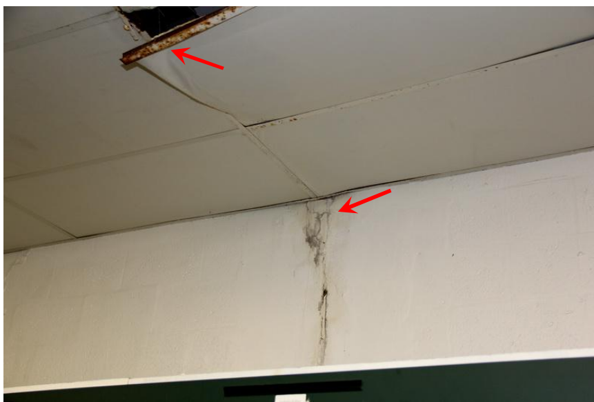
Typical view of water intrusion at the wall and ceiling.
