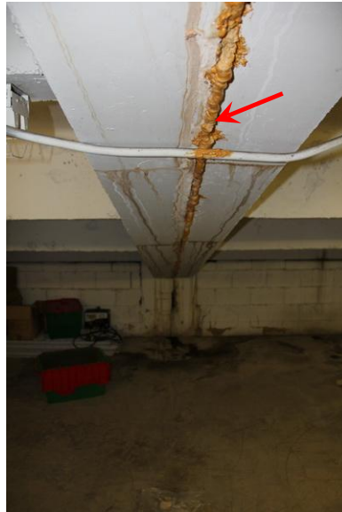
Typical view of deteriorated sealant.
