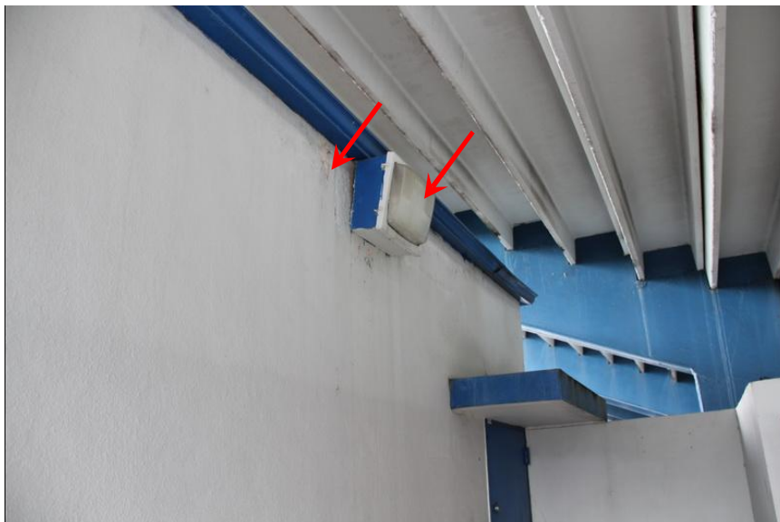
View of Failing Paint and wall pack lighting fixtures which is typical of all bathroom structures.
