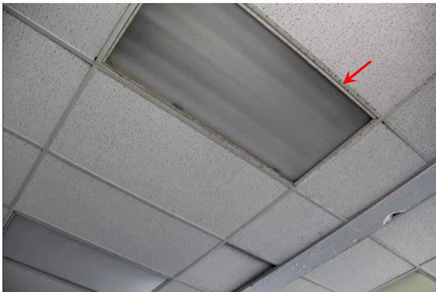
View of acoustic ceiling frame corrosion.
