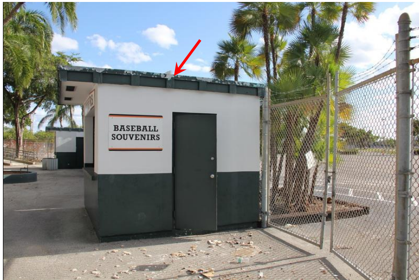
View of roof edge flashing paint peeling.
