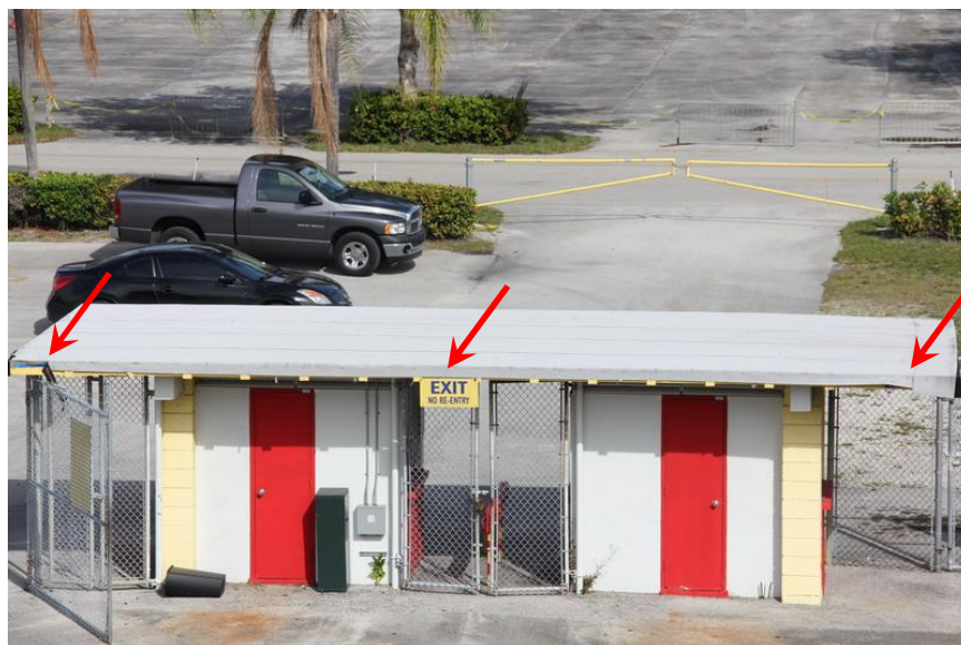
View of the Incomplete Roof Flashing
