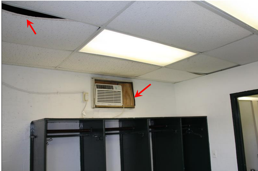
View of wall A/C unit and sagging roof tiles.
