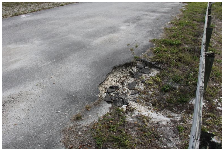
View of pavement edge deterioration.
