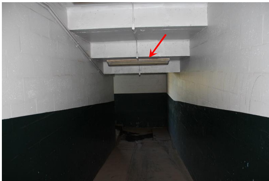
View of rusted and discolored ceiling light.
