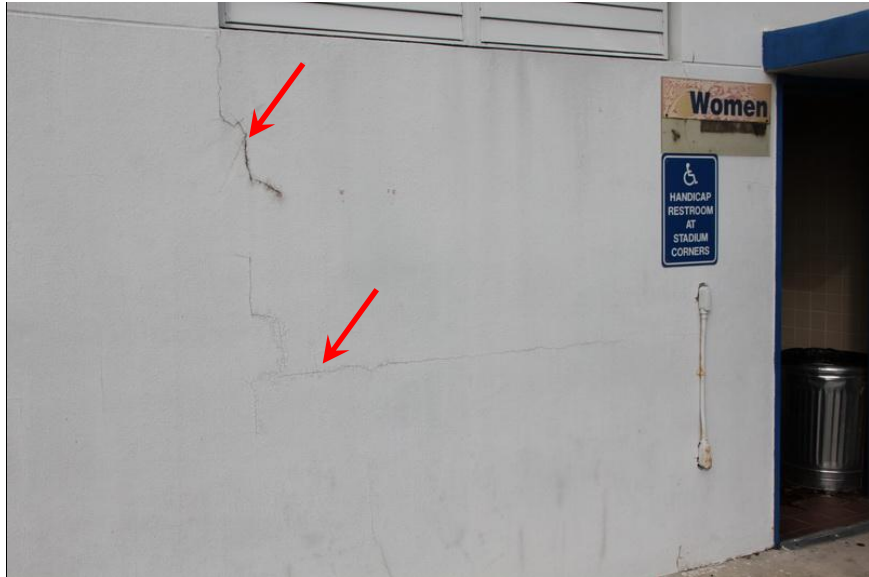
View of typical exterior cracking.
