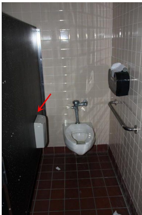
View of missing grab bar.
