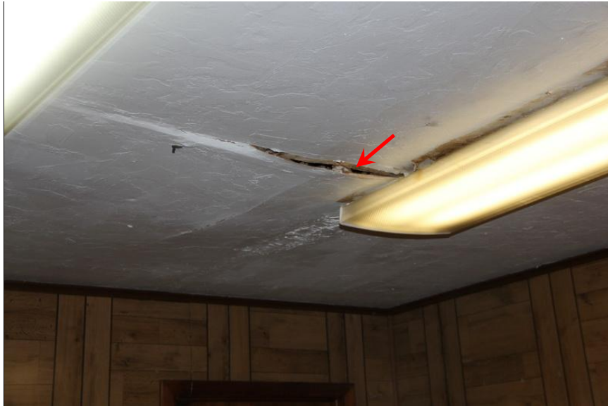
Typical view of failing roof member.
