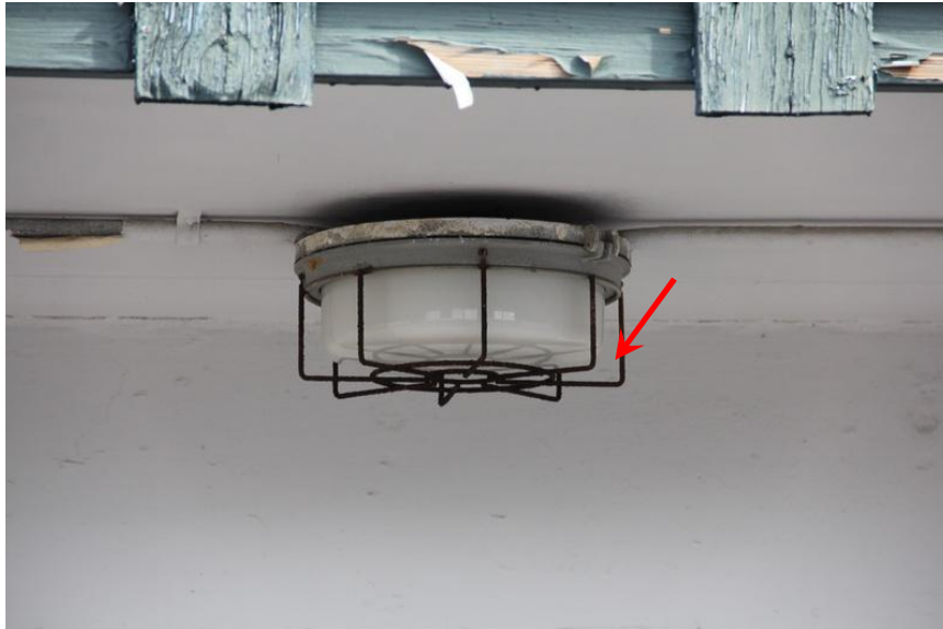
View of corroded wire guard.
