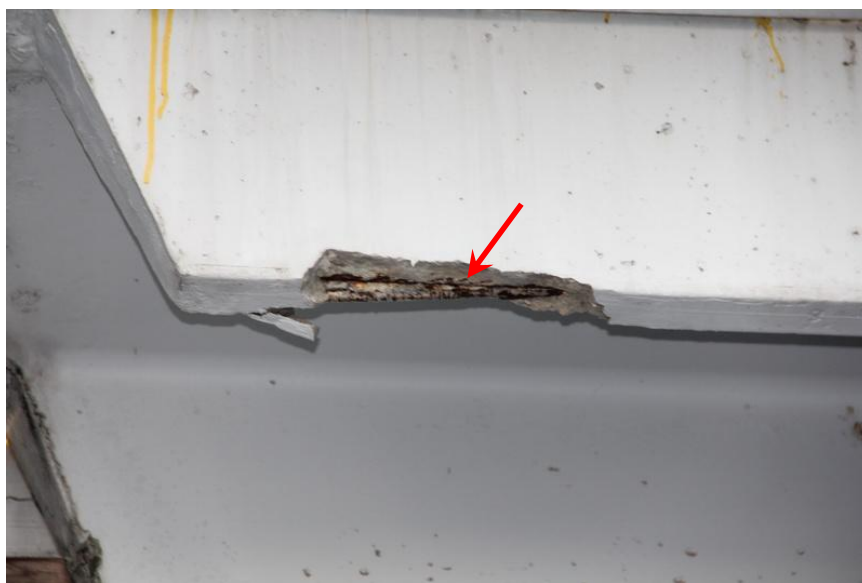
View of Exposed Reinforcing bars in the Concrete Stadium Beam.
