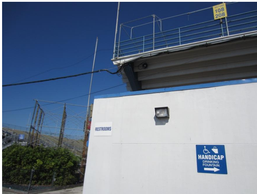
View of communications wires installed exposed along the stadium seating area.
