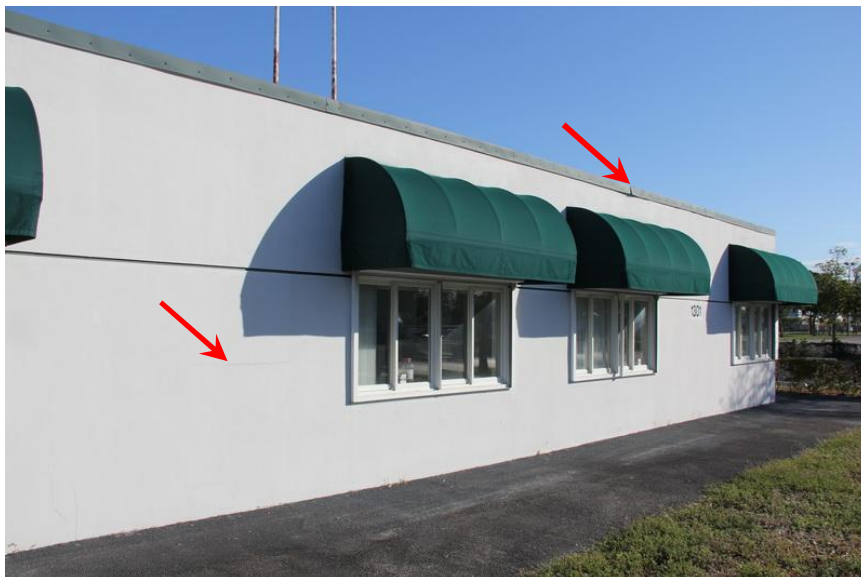
View of roof flashing and wall crack.
