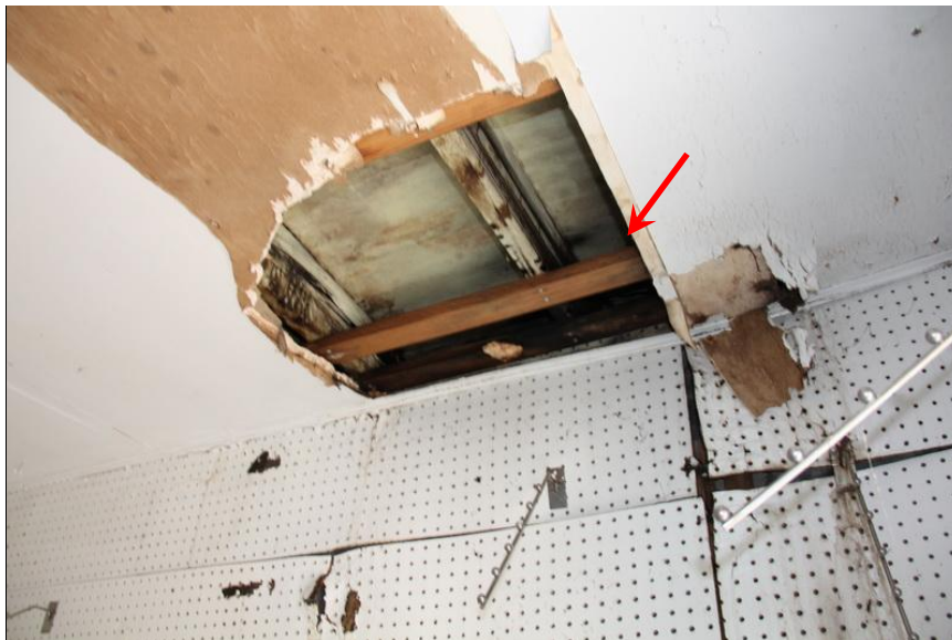
Typical view of interior ceiling water intrusion.
