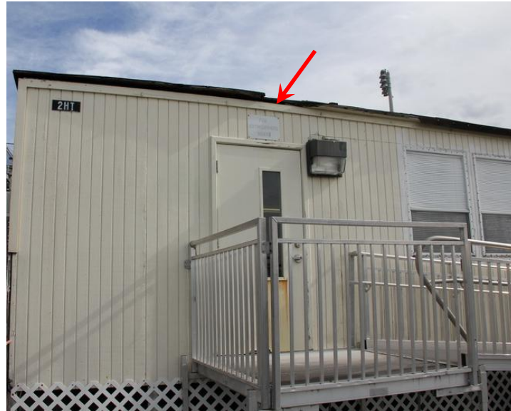
View of incomplete roof flashing.
