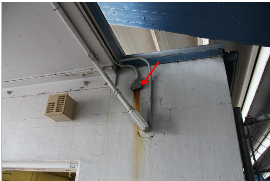
View of corroded junction box.
