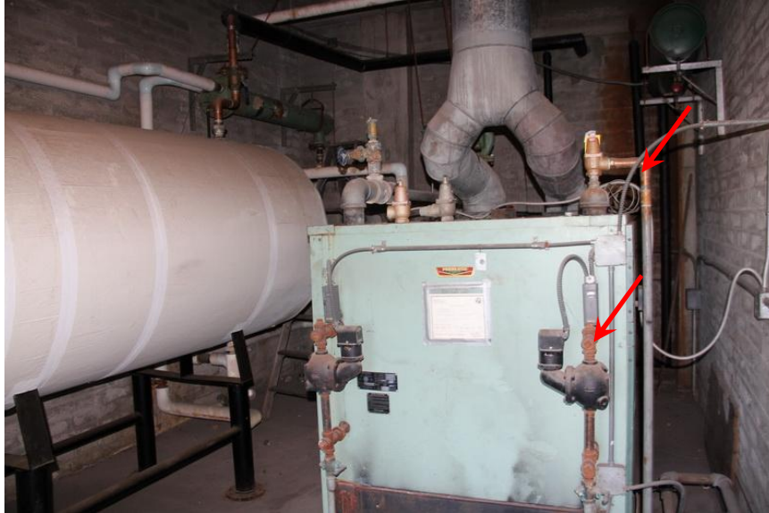
View of the corroded boiler components.
