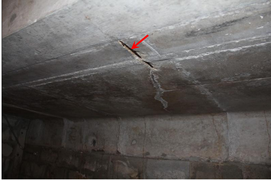
Typical view of the exposed rebar
