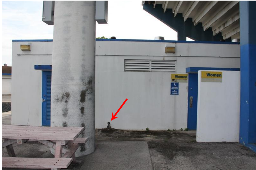
View of condensate line.
