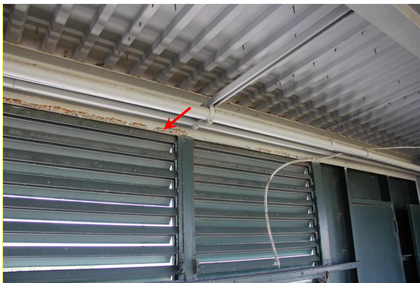
View of metal frame corrosion.
