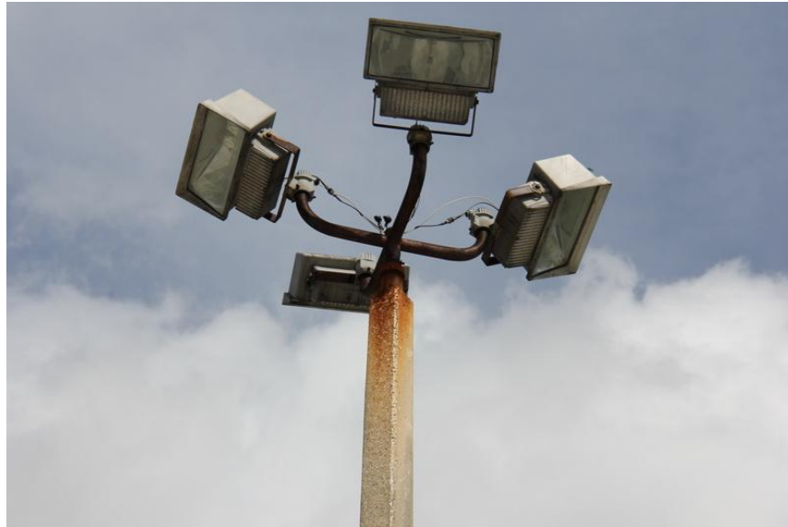
View of the pole mounted flood light fixtures that do not meet current lighting codes.
