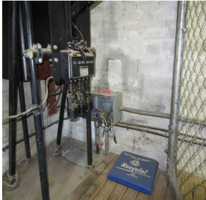
View of High Voltage breakers and equipment. Typically equipment of this voltage rating is housed inside the power company's transformer vault room. There are no electrical plans describing this equipment.
