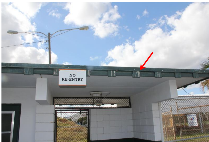
View of roof flashing paint flaking.
