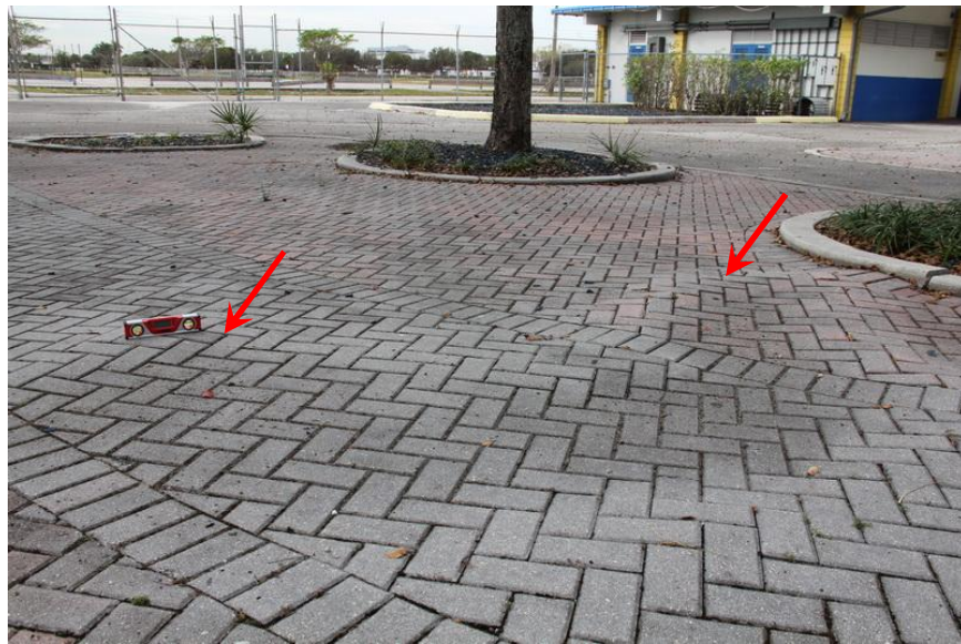
View of the typical raised and settled pavers.
