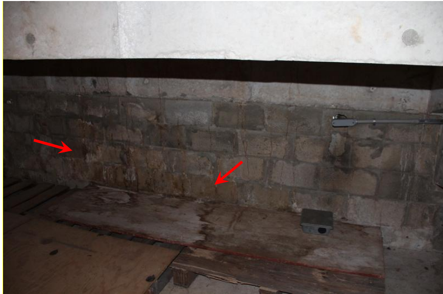
Typical view water intrusion
