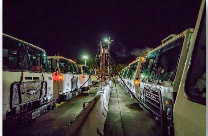
Our state-of-the-art CNG fueling station at WM's Southern Sanitation is ready and waiting to fuel the City's new fleet at the start of service.
