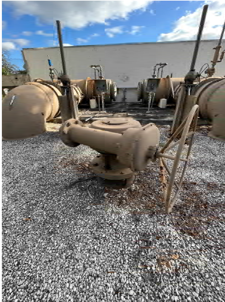
Figure 2: Existing valve on east side of manifold system and open in normal operating conditions letting flow into Repump B. Labeled as valve 2 in PDF markup.
