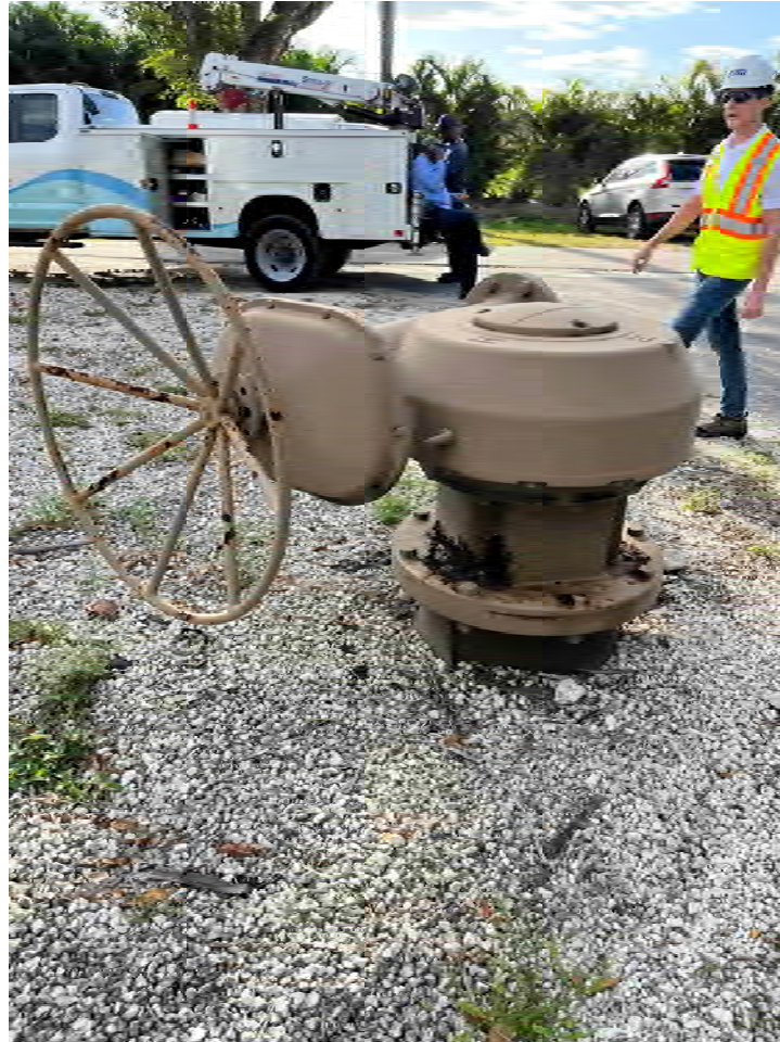
Figure 1: Existing Valve on south side of manifold appears to be in closed position. Labeled as valve 1 in PDF markup.
