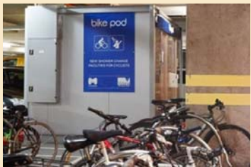
[Figure 4.256] Shower and change facilities for cyclists at the work place.
