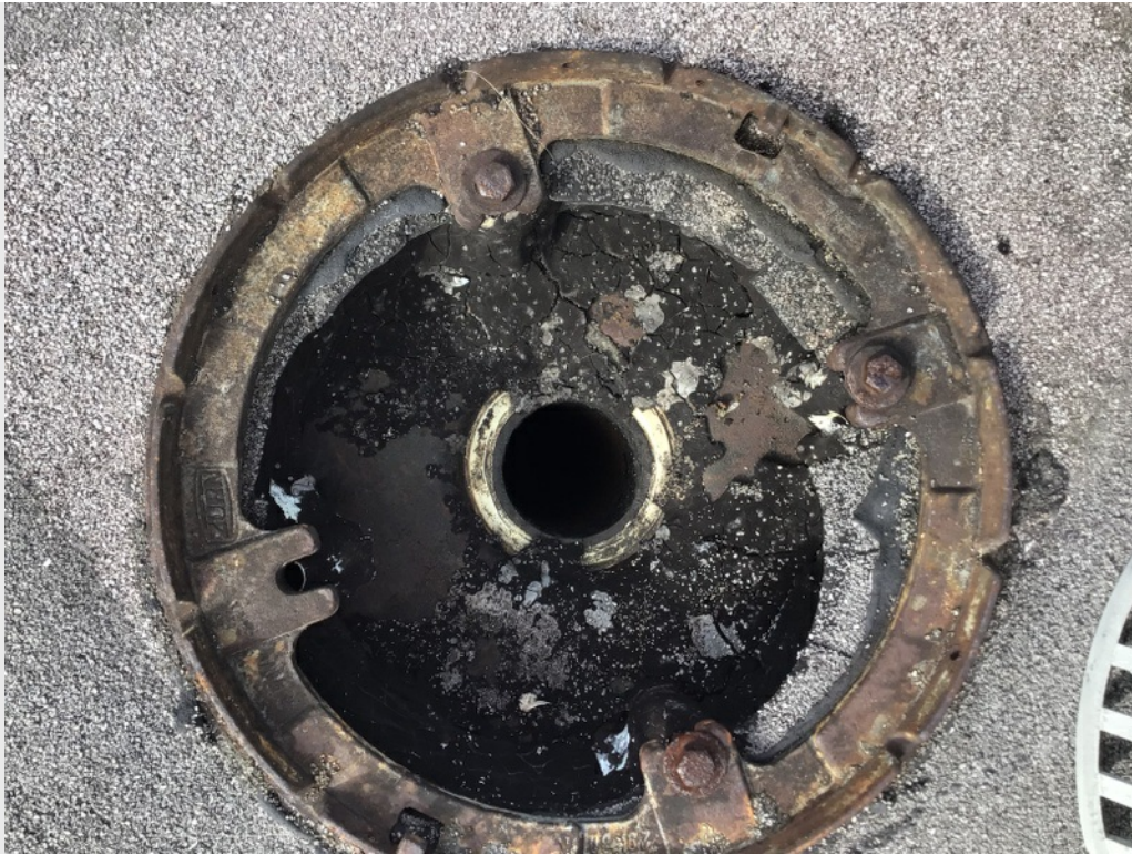
( 31 ) Internal drain, strainer bolt missing. (Typical detail)
