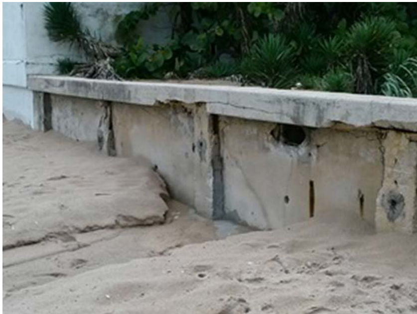
Location 3. NE 27 Street at Fort Lauderdale Beach (Looking West) Stormwater runoff is going through and over the top of the existing seawall causing the sand to washout to the Ocean.
