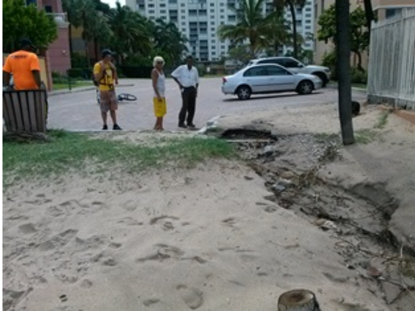
Location 1. NE 22 Street at Fort Lauderdale Beach (Looking West from Beach). Stormwater street runoff is causing the sand to washout to the Ocean.
