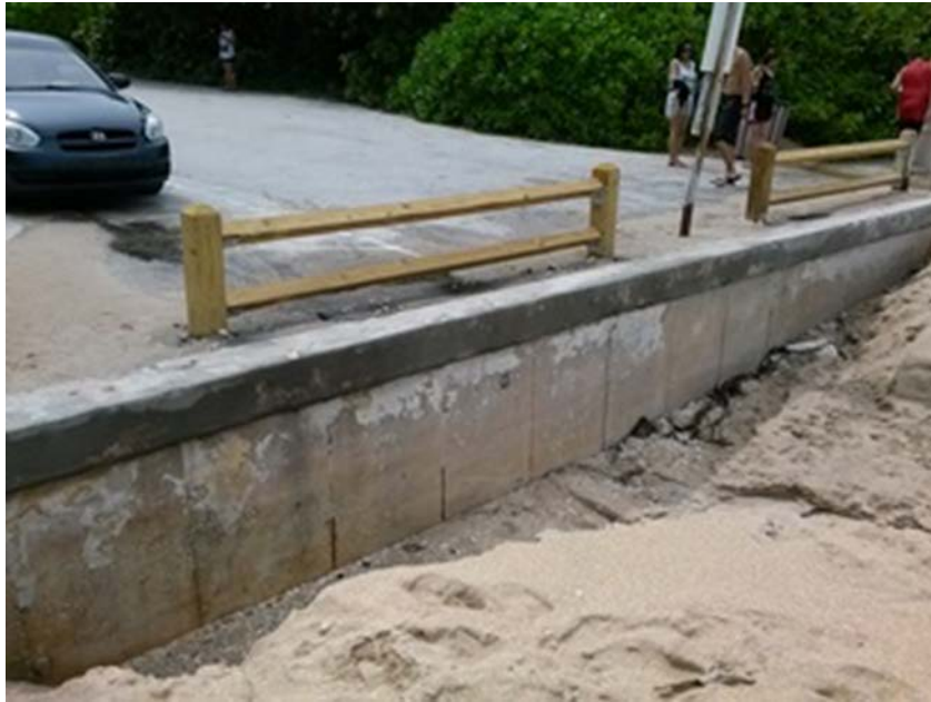
Location 2. NE 23 Street at Fort Lauderdale Beach (Looking West) Stormwater street runoff is going over the top of the existing seawall, causing the sand to washout to the Ocean.
